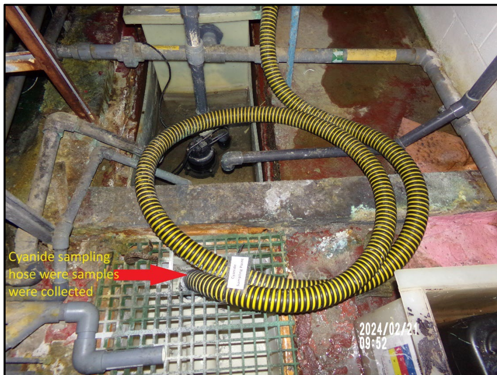
Photo 2. Facility cyanide sampling hose where samples are collected for laboratory analysis.
