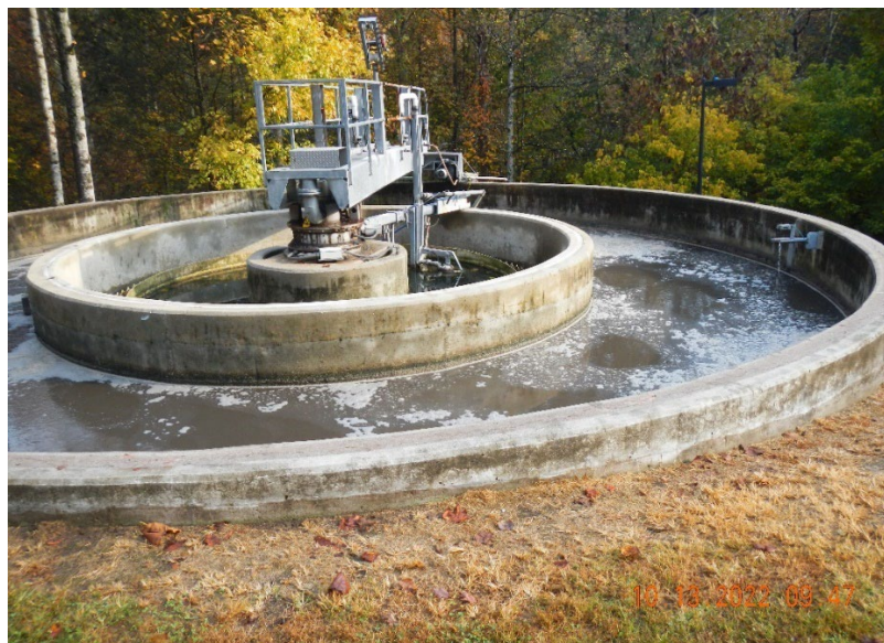
Picture 2. Thin MLSS in outer aeration basin.
