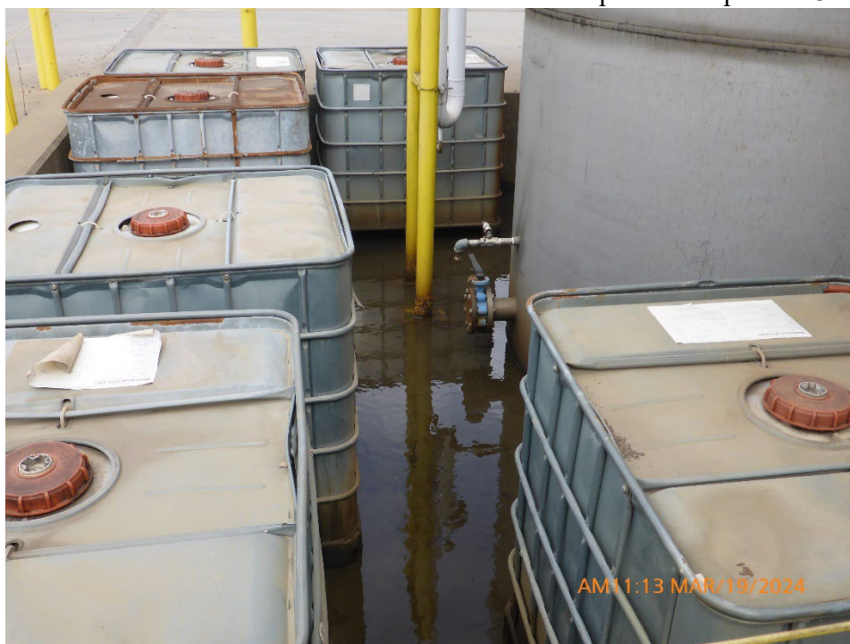
Photograph 3: Water inside containment area around methanol treatment column at Eureka Resources.
