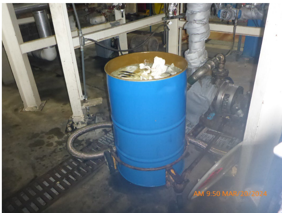
Photograph 4: Drum of various materials (a combination of liquid, fats, and solids) without secondary containment in the ethylene oxide production area at Arxada.
