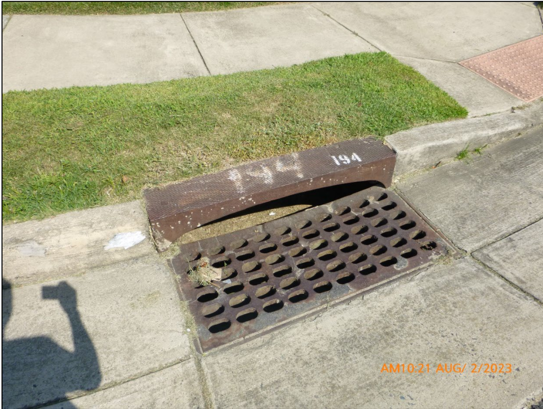
Photograph 17. Carson Avenue – View of an unlabeled storm drain on Carson Avenue.
