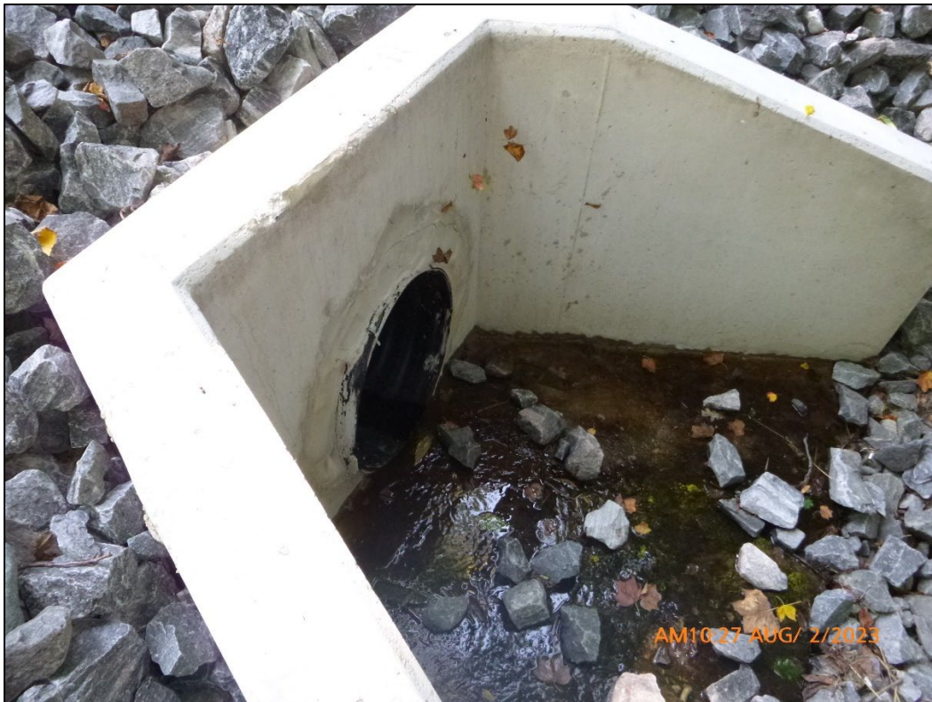
Photograph 16. Carson Avenue Stream Scouring – View of the mouth of the outfall.
