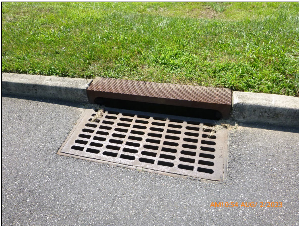
Photograph 20. Deptford Sports Complex – View, facing south, of an unlabeled catch basin that discharges stormwater to outfall B119.
