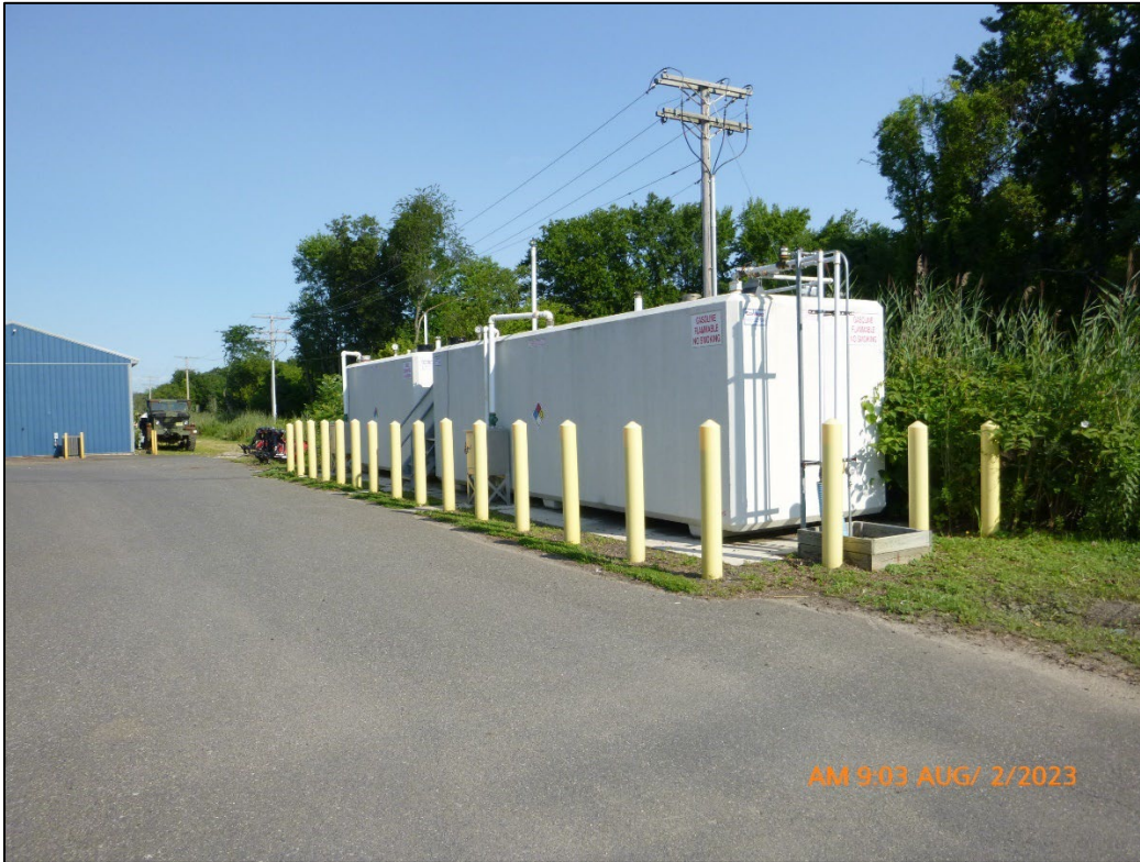
Photograph 5. Department of Public Works – View, facing northwest, of the 7,000-gallon gasoline and 3,000-gallon diesel double wall aboveground storage tanks.
