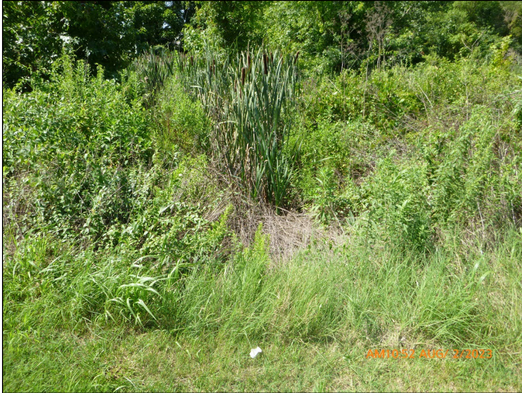
Photograph 21. Deptford Sports Complex – View, facing southeast, of the location of outfall B118. The vegetation around the outfall is overgrown making the outfall difficult to find and access.
