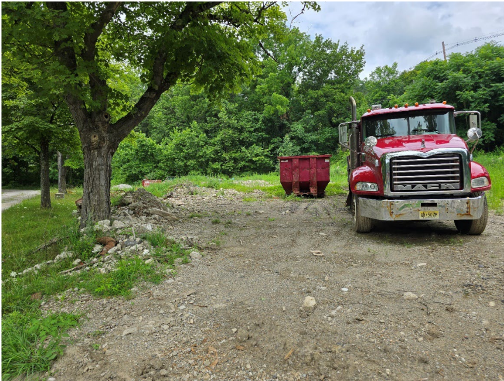
Figure 9: Bella Truck and debris, alternate angle. The red container was filled with metal at the time of inspection.
