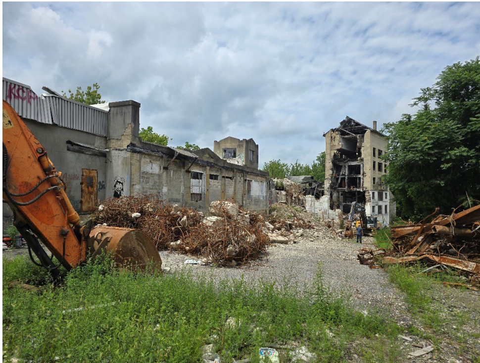
Figure 2: Demolition Site. Note the removed wall on the 7-story structure, and the concrete and metal debris.
