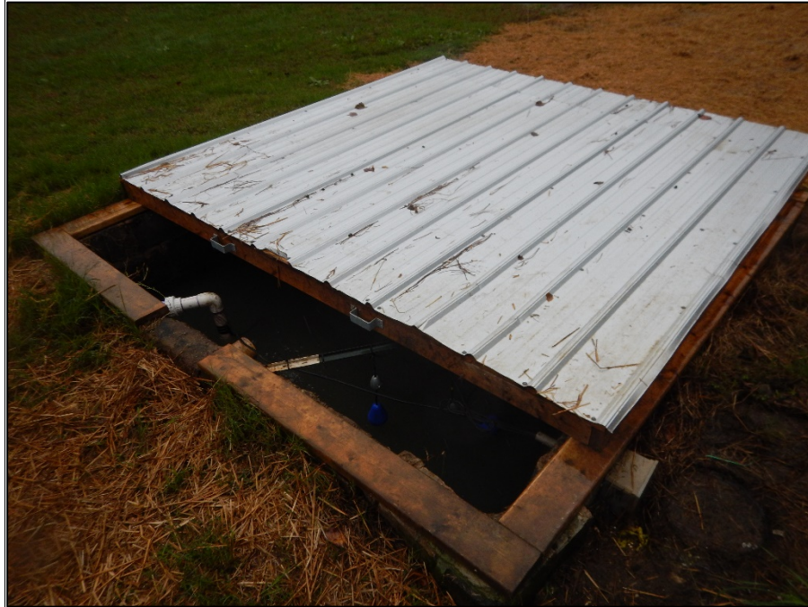
Photograph 1. View of the wastewater collection tank.
