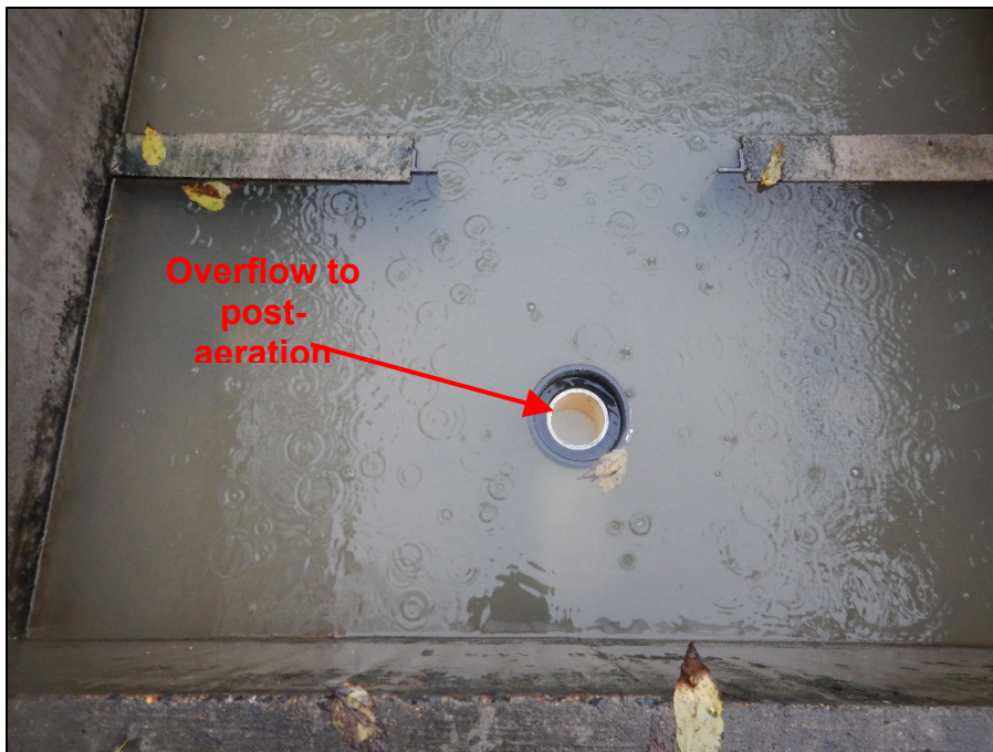
Photograph 10. Additional view the effluent in the holding tank. Note the turbidity.
