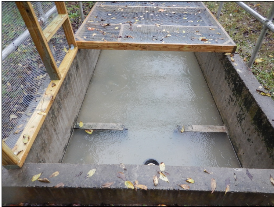
Photograph 9. View of the effluent holding tank. Note the effluent in the chamber was turbid.
