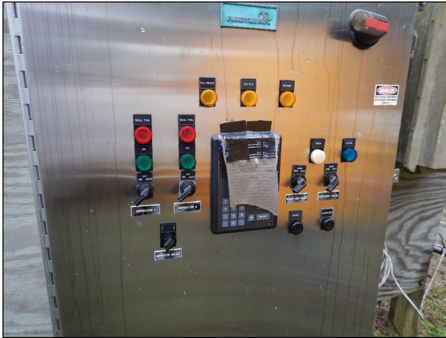
Photograph 5. View of the SBR control panel.
