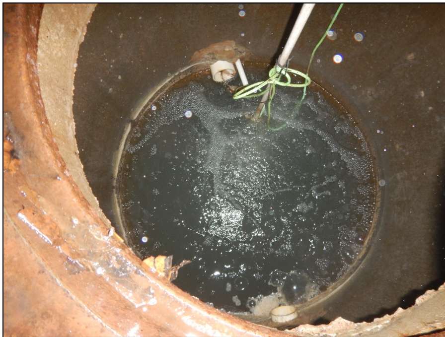
Photograph 11. View inside the post aeration chamber. Note that the effluent appeared cloudy.
