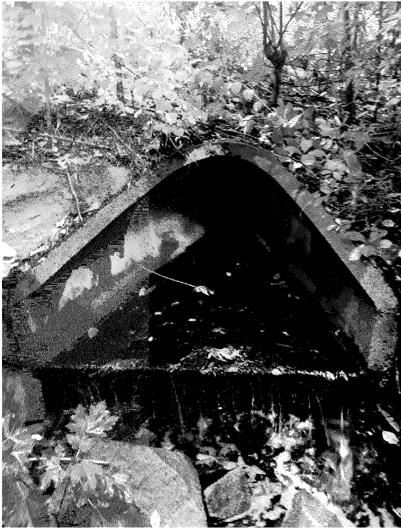
LundStS: Outfall flowing south into Salmon Brook. Note suds in pool in the lower left of photo. Location of dead mouse is indicated by a red circle.
