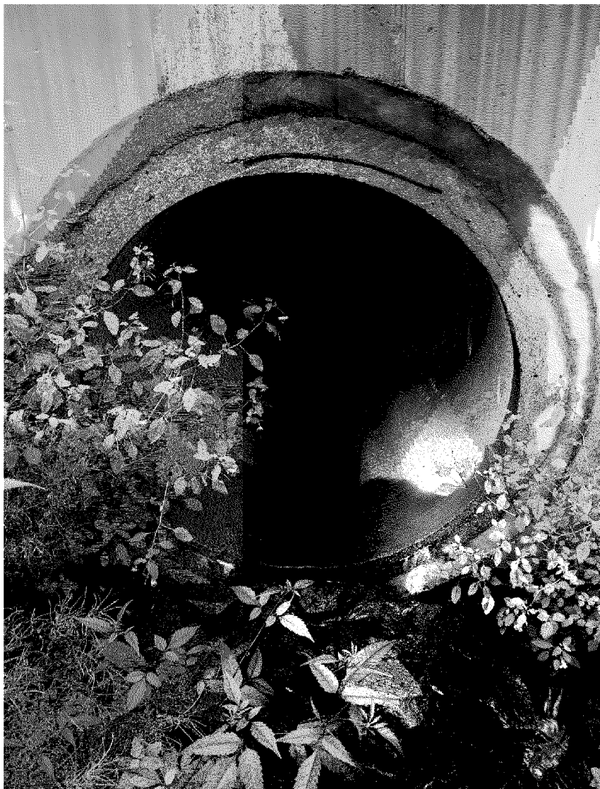
PineStE : Outfall flowing north into the Nashua River. Note the green algae growth in pipe.
