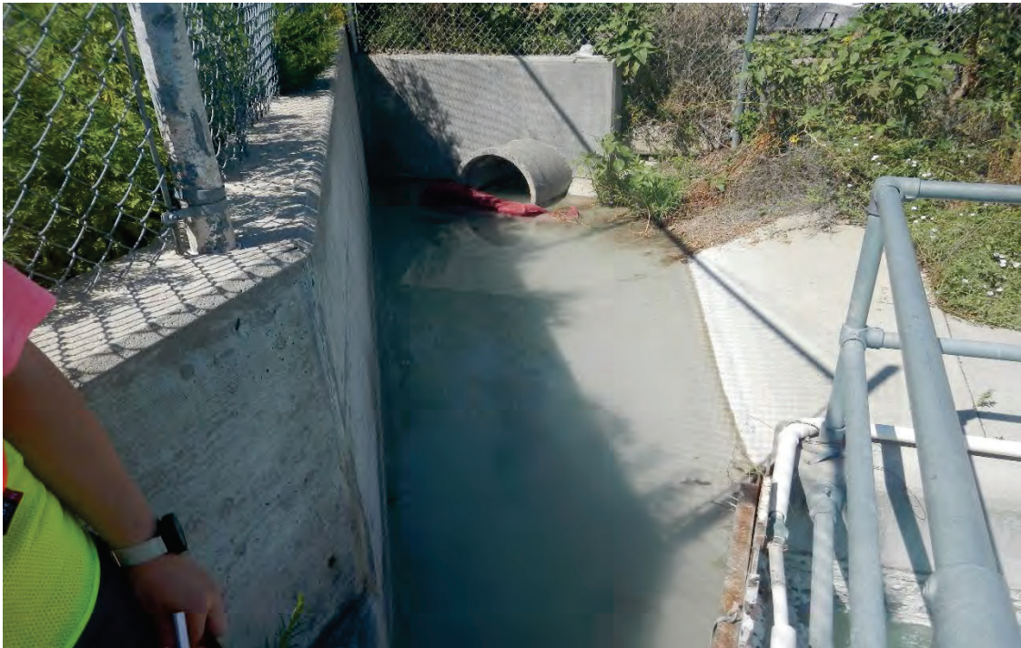
Photo 13, Outfall 01 discharging Washout Holding Pits water
