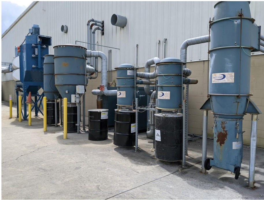
Photograph 3 of 3: Hazardous Waste Blast Media Collection Area
