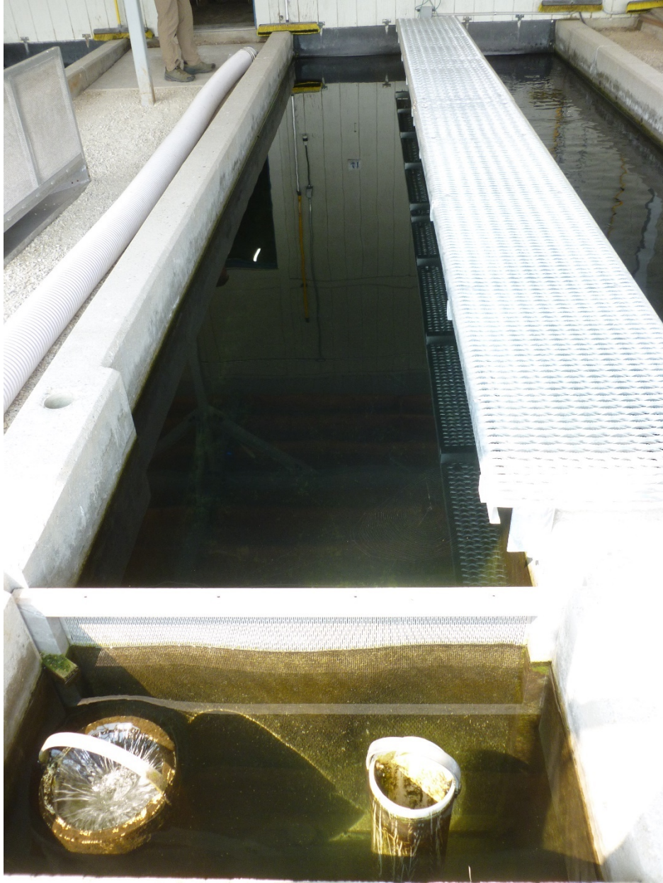
Photo 5 / P1000993 – Raceway, outdoor section facing toward building.
