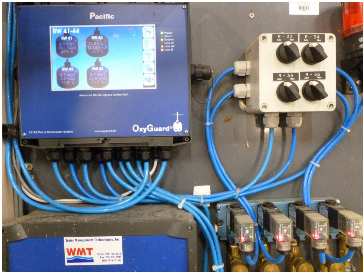
Photo 8 / P1000995 – Oxyguard® Monitoring and Control Unit.
