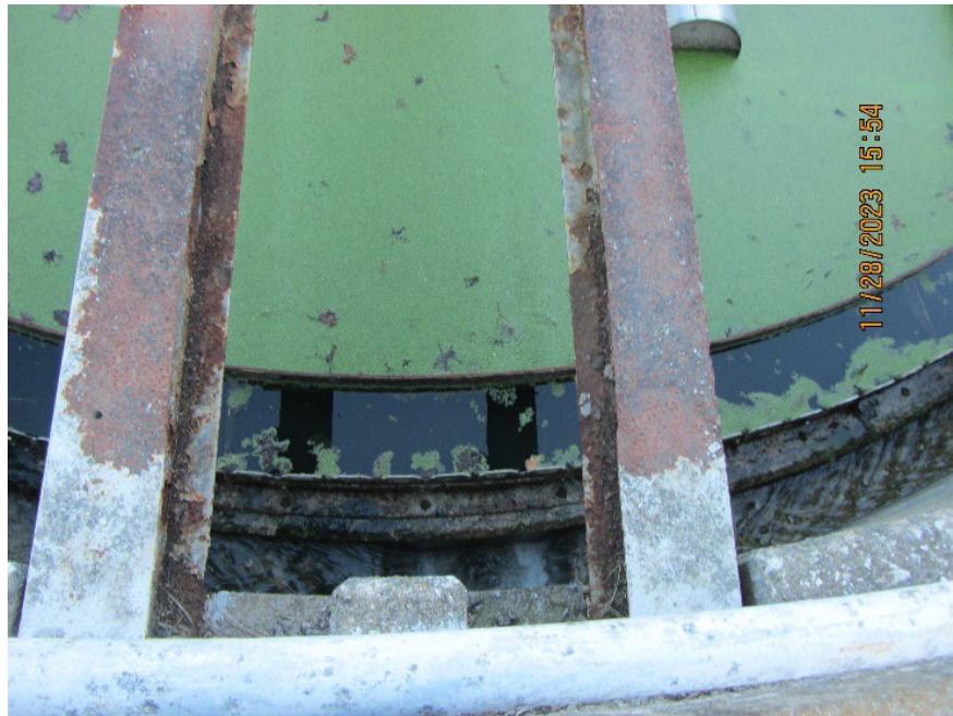
19: IMG_0417 Description: Effluent sampling location Location: Final clarifier Camera Direction: Northeast Date/Time: 11/28/23, 3:54 p.m.
