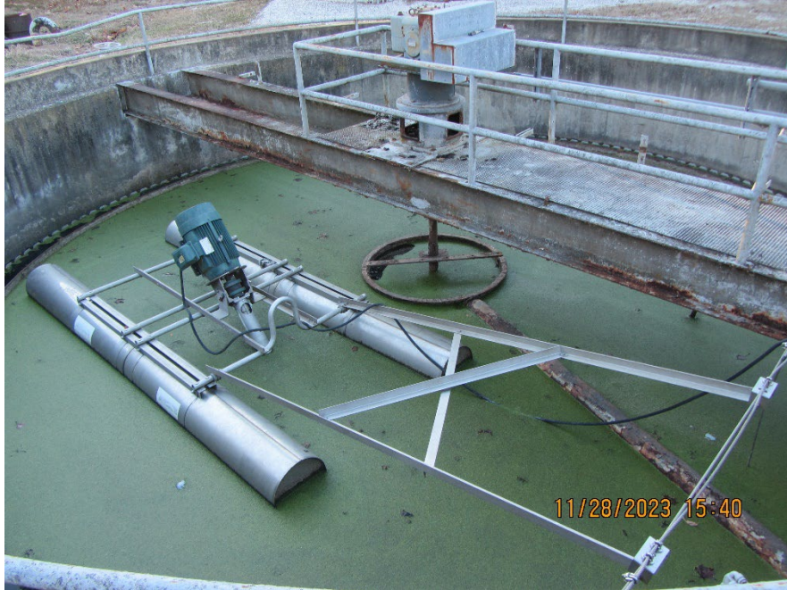
18: IMG_0416 Description: Final clarifier Location: Northwest of ASU Camera Direction: Wes Date/Time: 11/28/23, 3:40 p.m.
