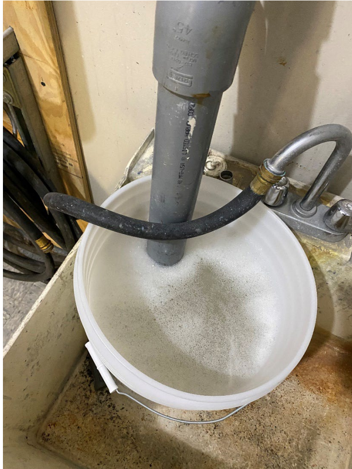
Photo 2: Bucket collection system located inside sink of utility room. Note: presence of bubbles on surface.
