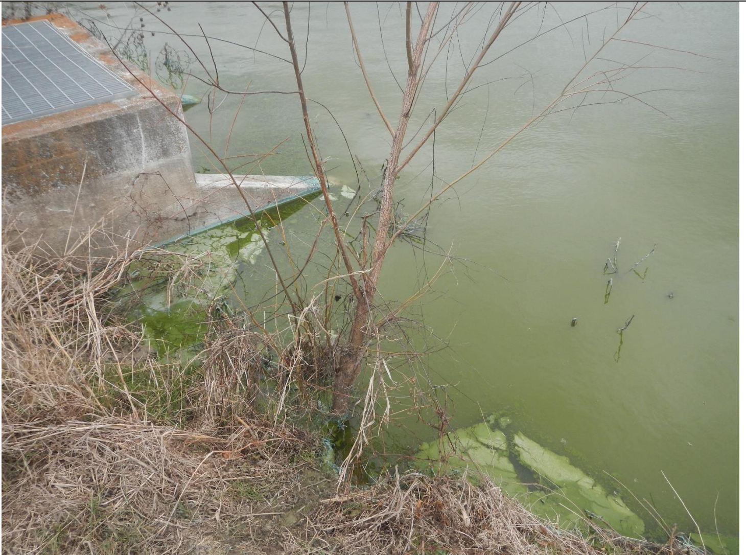
Figure 3: Vegetation growth that needs maintenance at cell 2.
