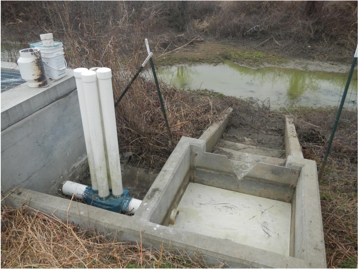
Figure 2: Discharge point to ditch with foamy liquid before V-notch weir.
