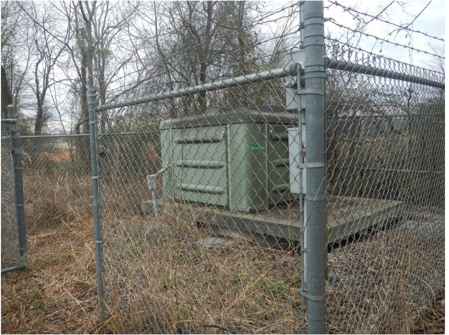
Figure 5: Washout at pump station pad.
