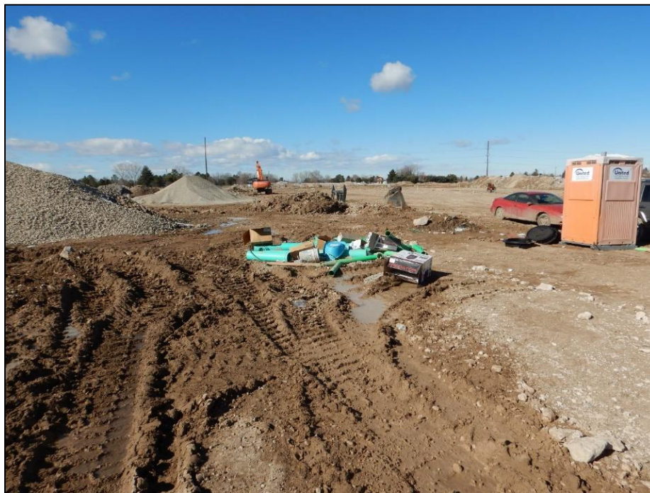
Photograph 4. View, facing south, of a pile of uncontained construction waste located at the center of the Site.
