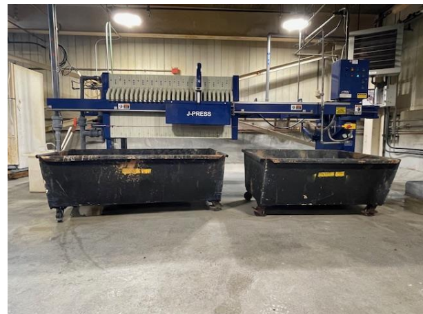
Photograph 32: WWTP #2 Filter press and sludge transfer containers.
