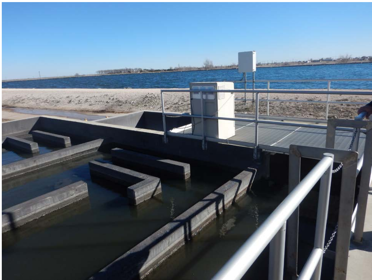
Picture of the chlorine chamber and the WWTP's automatic sampler. February 24, 2020 3:53 PM (DSCN 1721). Photographed by D. Esparza.
