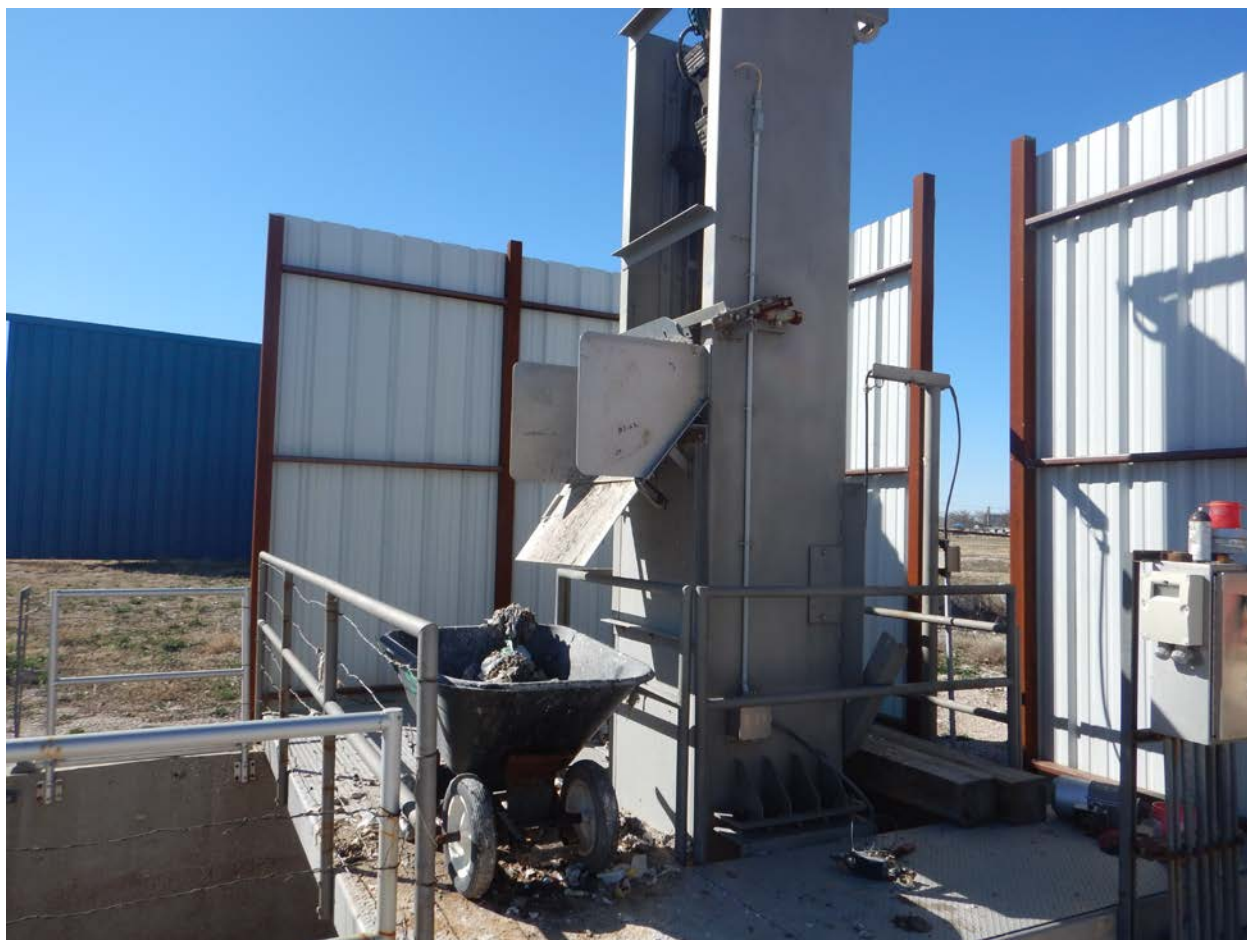
Picture of the WWTP's headworks/bar screen combination used in the removal of rags and other various large debris items contained in the influent flow. February 24, 2020 3:30 PM (DSCN 1714). Photographed by D. Esparza.
