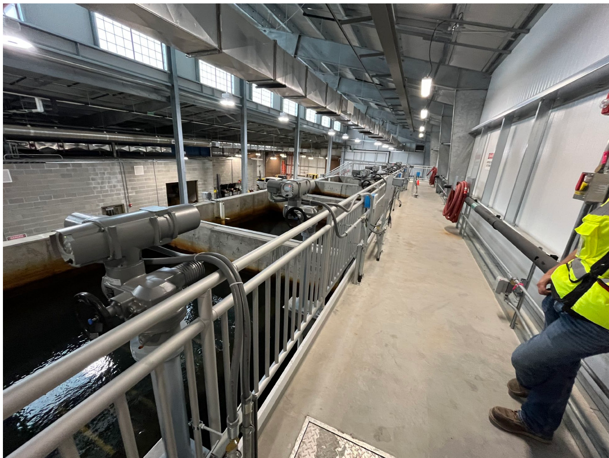
View of the filtration basin inside the CTPL facility. (IMG_0029) (July 10, 2024: 2:09 PM) Photographed by D. Esparza
