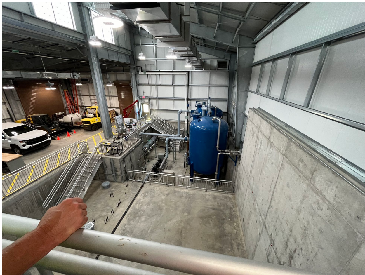
View of the granular activated carbon (GAC) filter system inside the CTPL facility. (IMG_0030) (July 10, 2024: 2:12 PM) Photographed by D. Esparza
