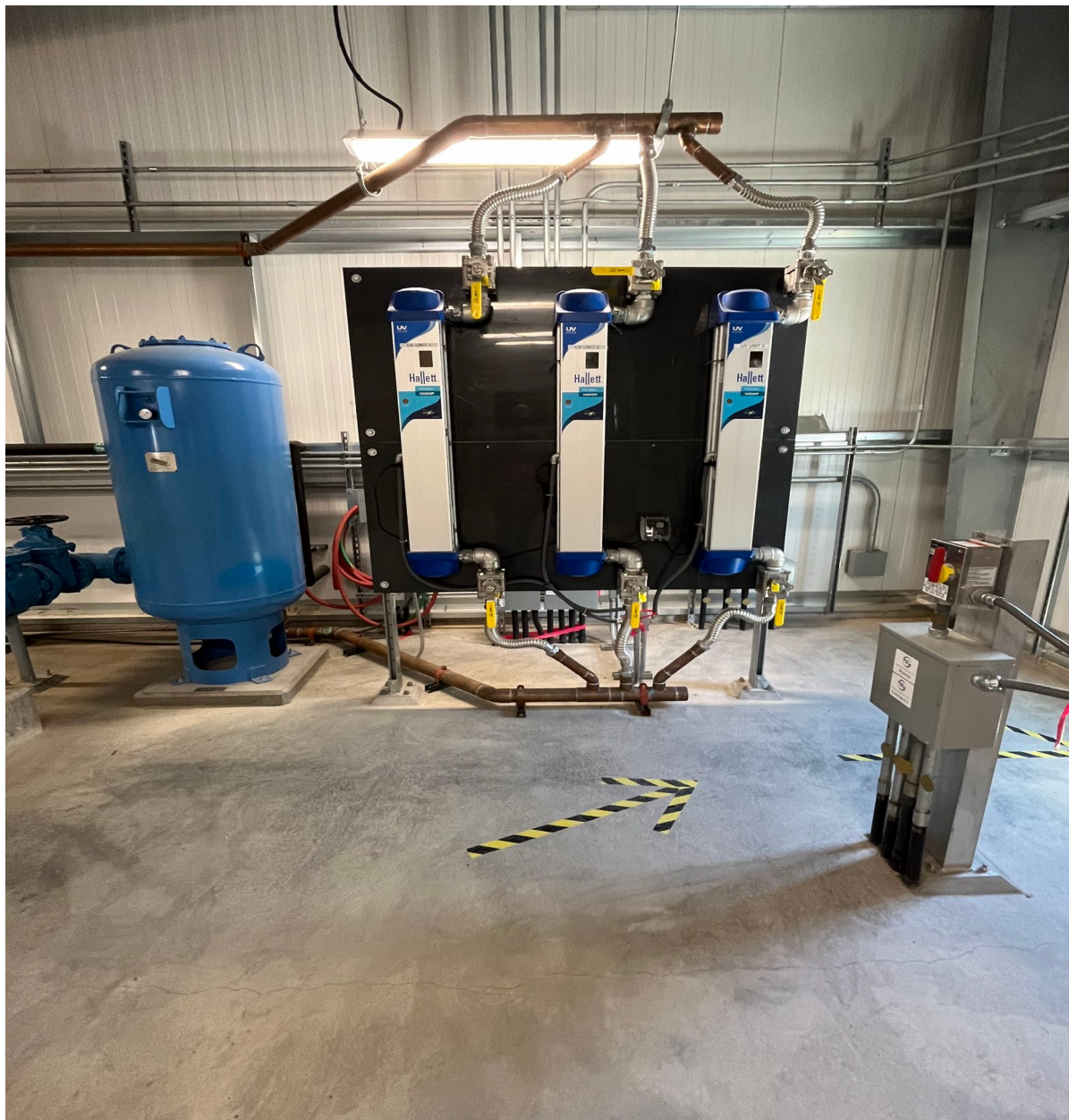
View of the Hallet ultraviolet (UV) disinfection system. (IMG_0039) (July 10, 2024: 2:30 PM) Photographed by D. Esparza
