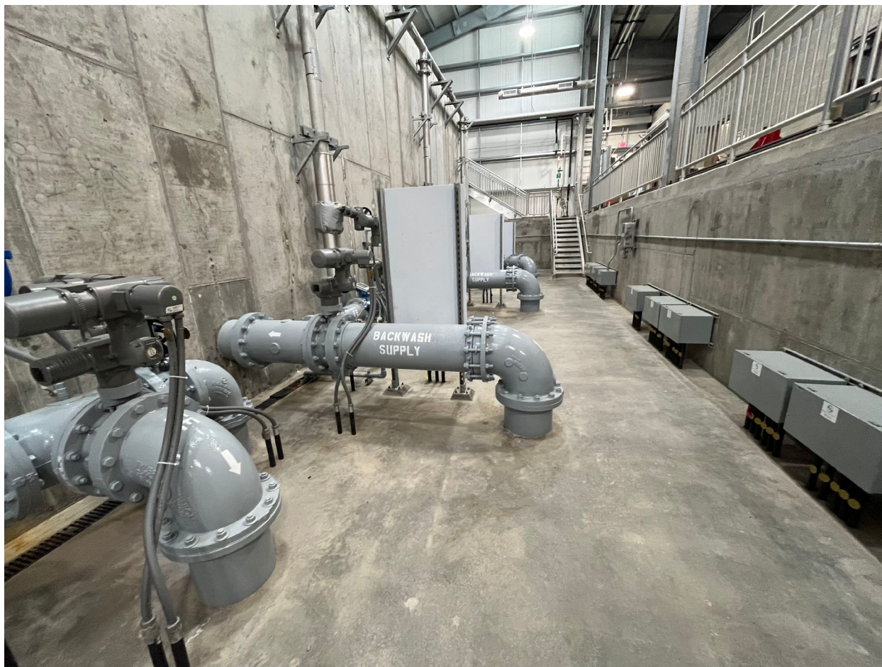
View of a portion of the process piping located inside the CTPL facility. (IMG_0031) (July 10, 2024: 2:17 PM) Photographed by D. Esparza
