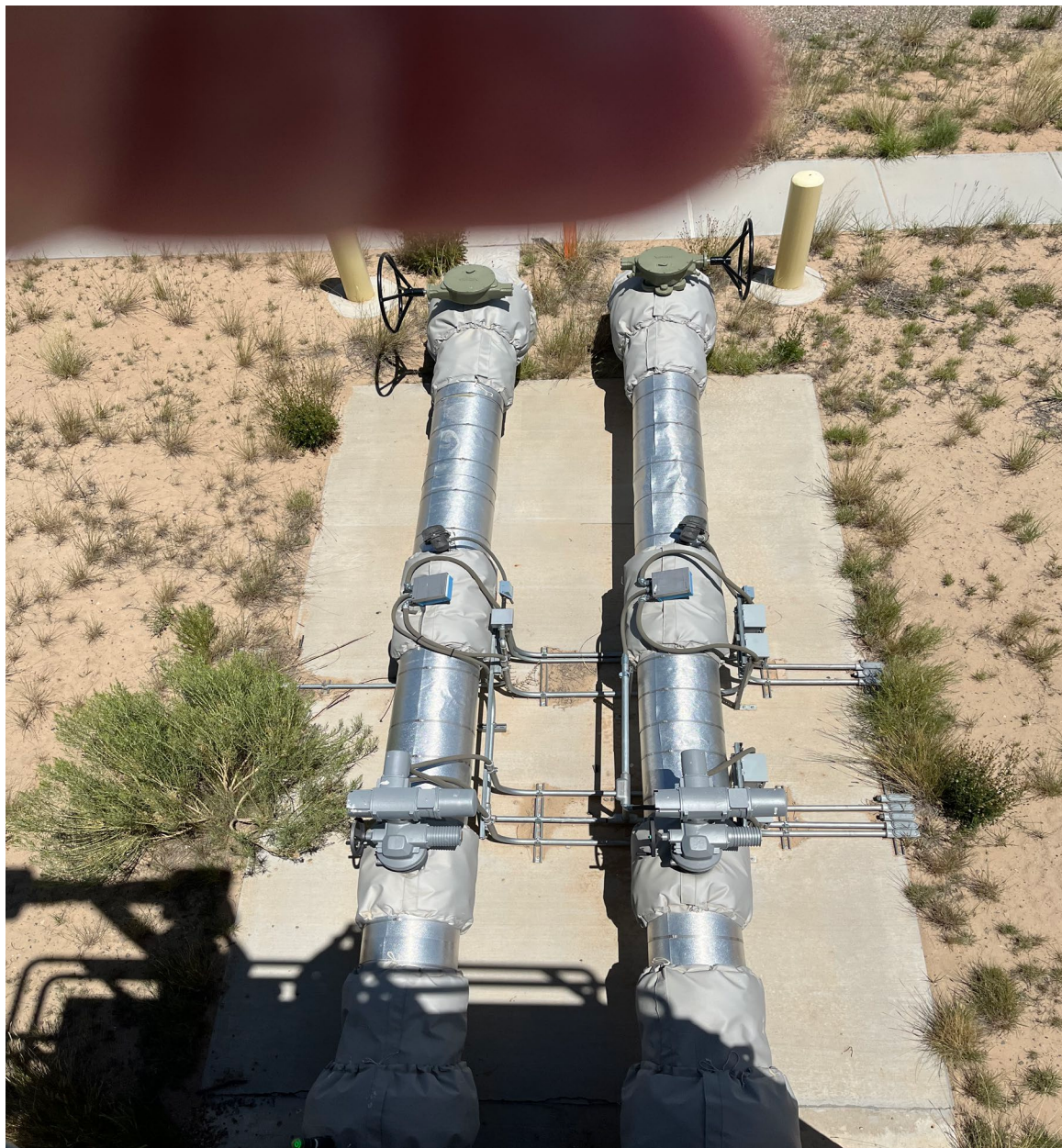
View of the raw water influent lines delivered from Pumping Plant #2 prior to the Rapid Mix process. (IMG_0013) (July 10, 2024: 1:51 PM) Photographed by D. Esparza
