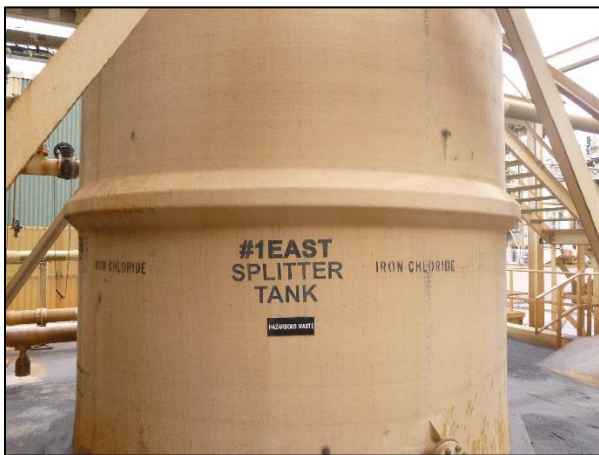
Photo 2: #1 East Splitter Tank.
