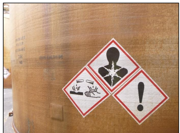
Photo 8: Primary Filter Storage Tank #2.
