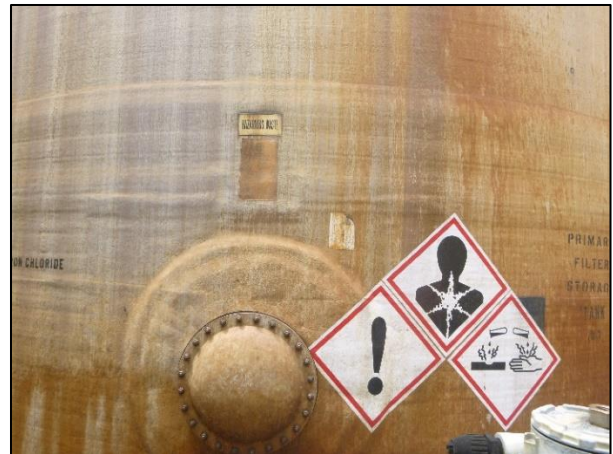
Photo 6: Primary Filter Storage Tank #1.
