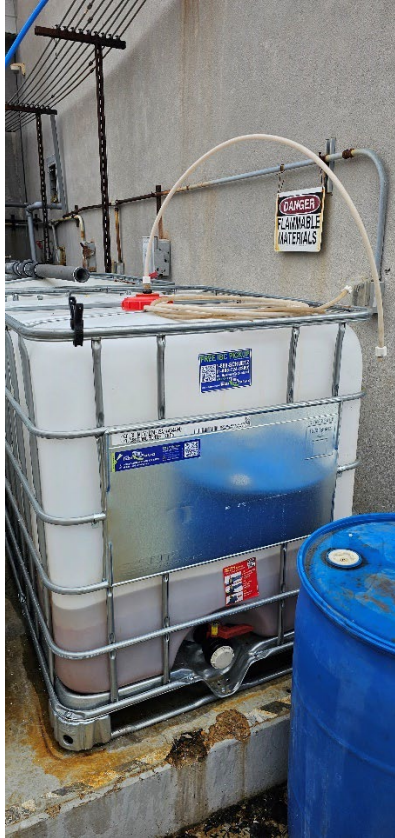
Figure 13: One tote located in the back pad area had an open hose connection attached to the top cap and was not closed.
