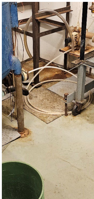
Figure 6: Absorbant pads observed in the polyramics lab were severely stained and saturated and no longer sufficient to properly contain hazardous waste spills.
