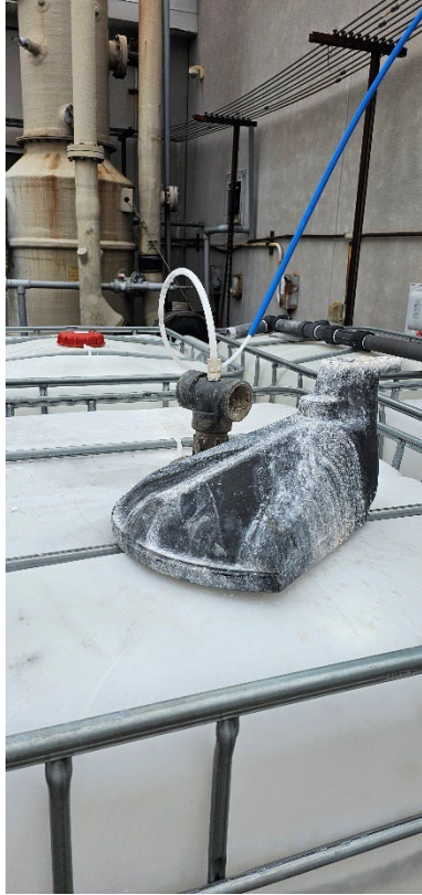
Figure 12: One tote located in the back pad area utilized a T pipe connector to vent vapors and was not closed.
