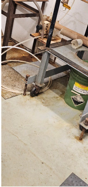
Figure 5: The 5-gallon satellite accumulation container located in the polyramics lab was not closed. Additionally, hazardous waste containing absorbant pads were observed in this figure. The absorbant pads were saturated and no longer sufficient to collect hazardous wastes.
