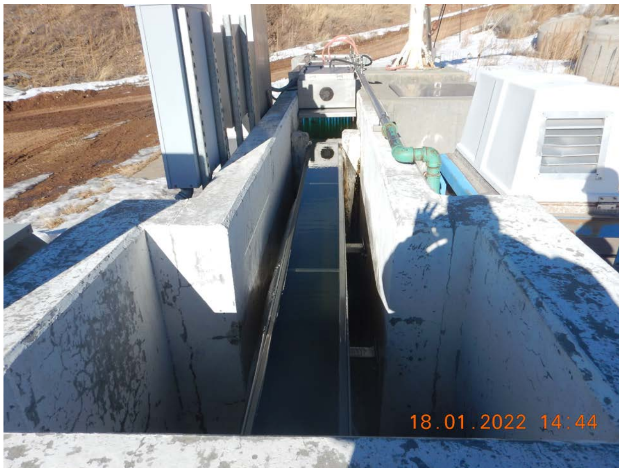
View of the Ultraviolet (UV) disinfection system situated over the concrete channels. (DSCN2087) Photographed by D. Esparza
