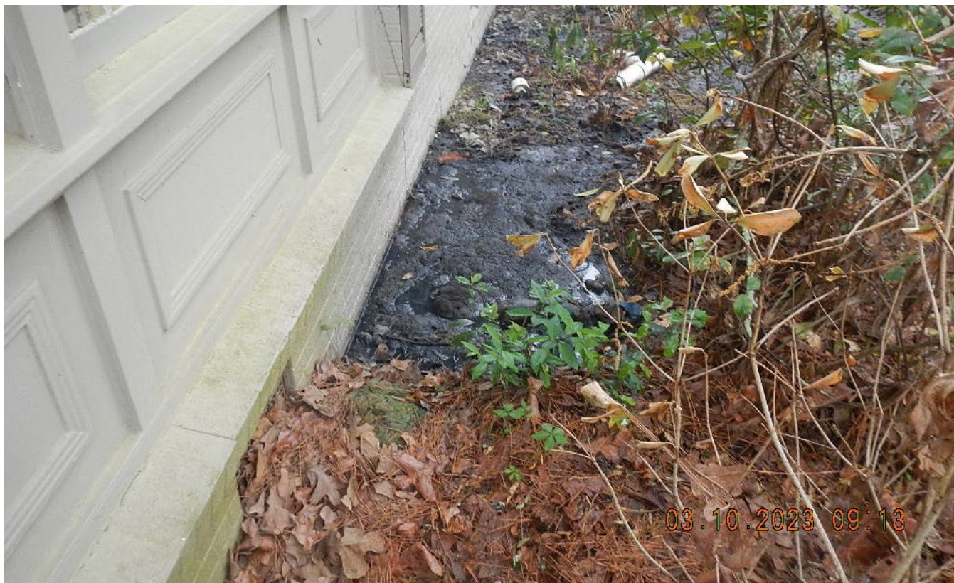
Photo 3. Raw sewage next to the house. The resident had to remove the lateral cap to prevent sewage from entering the house. It's unclear why a portion of the sewage lateral is removed but could be a result of washout from high sewage volume and pressure at the house being discharged from the sewer main.
