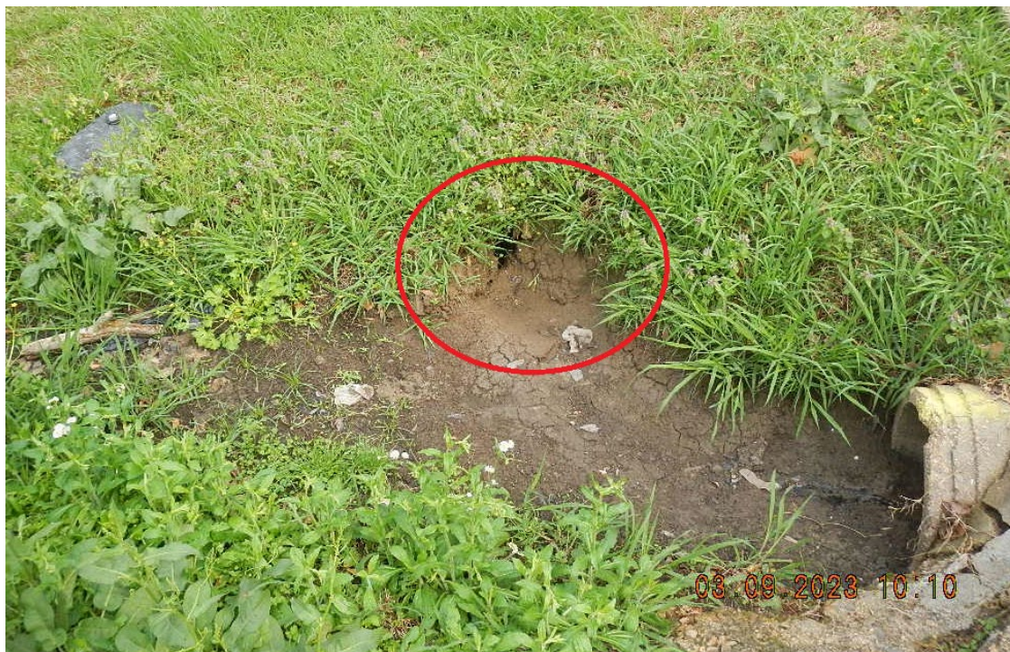
Photo 1. Sewage debris and sewer sludge was observed at the storm water ditch in front of 1444 Cherrie Avenue. Circled in red appears to be a weep hole where sewage is being released into the ditch.
