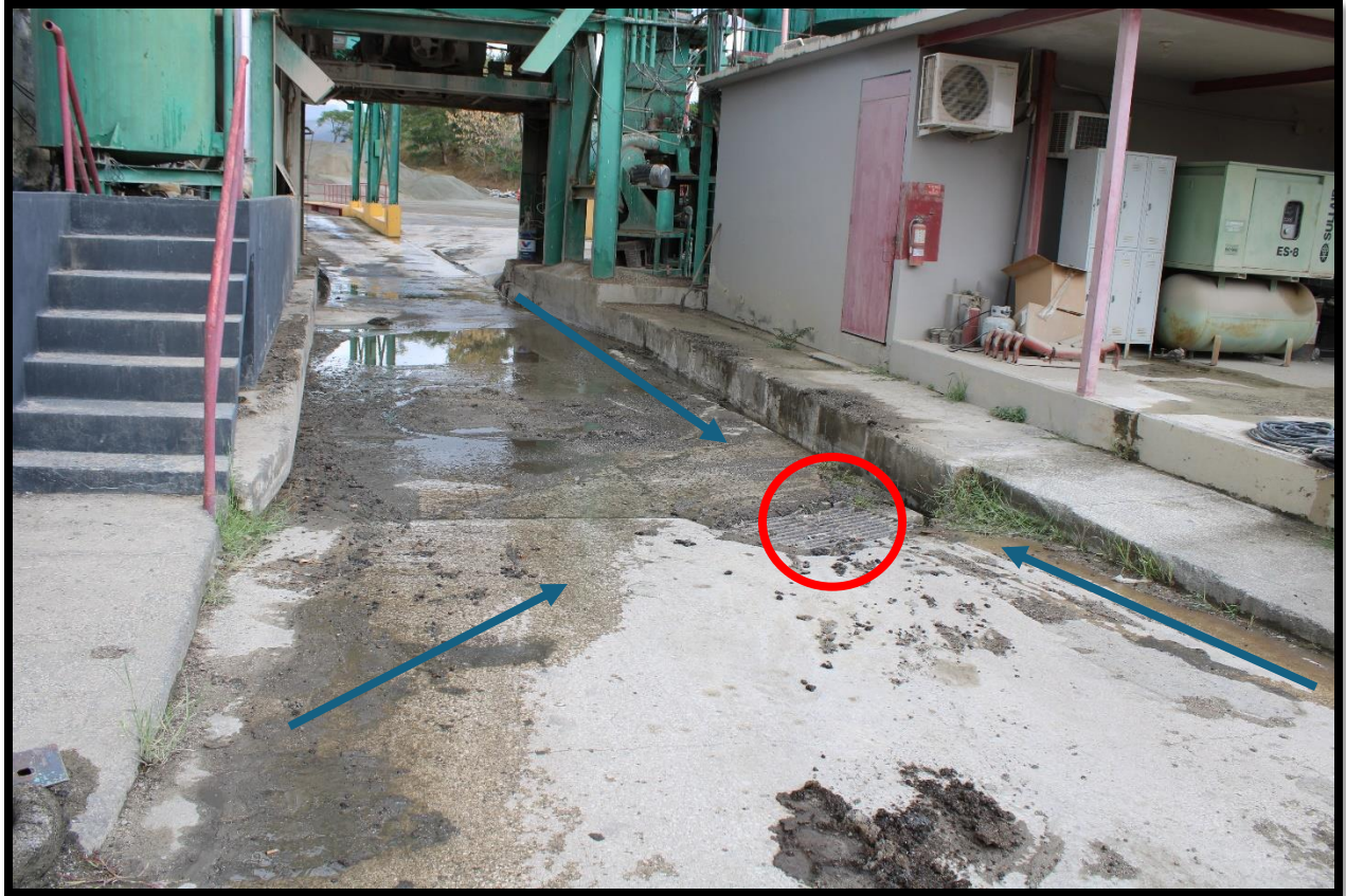
Picture 4 shows a storm sewer drain inlet (depicted by the red circle) located in the asphalt cement processing plant area. The inlet did not have inlet protection measure. A significant amount of sediment is visible around the inlet and in the stormwater runoff path. The blue arrows depict the flow path of stormwater runoff.
