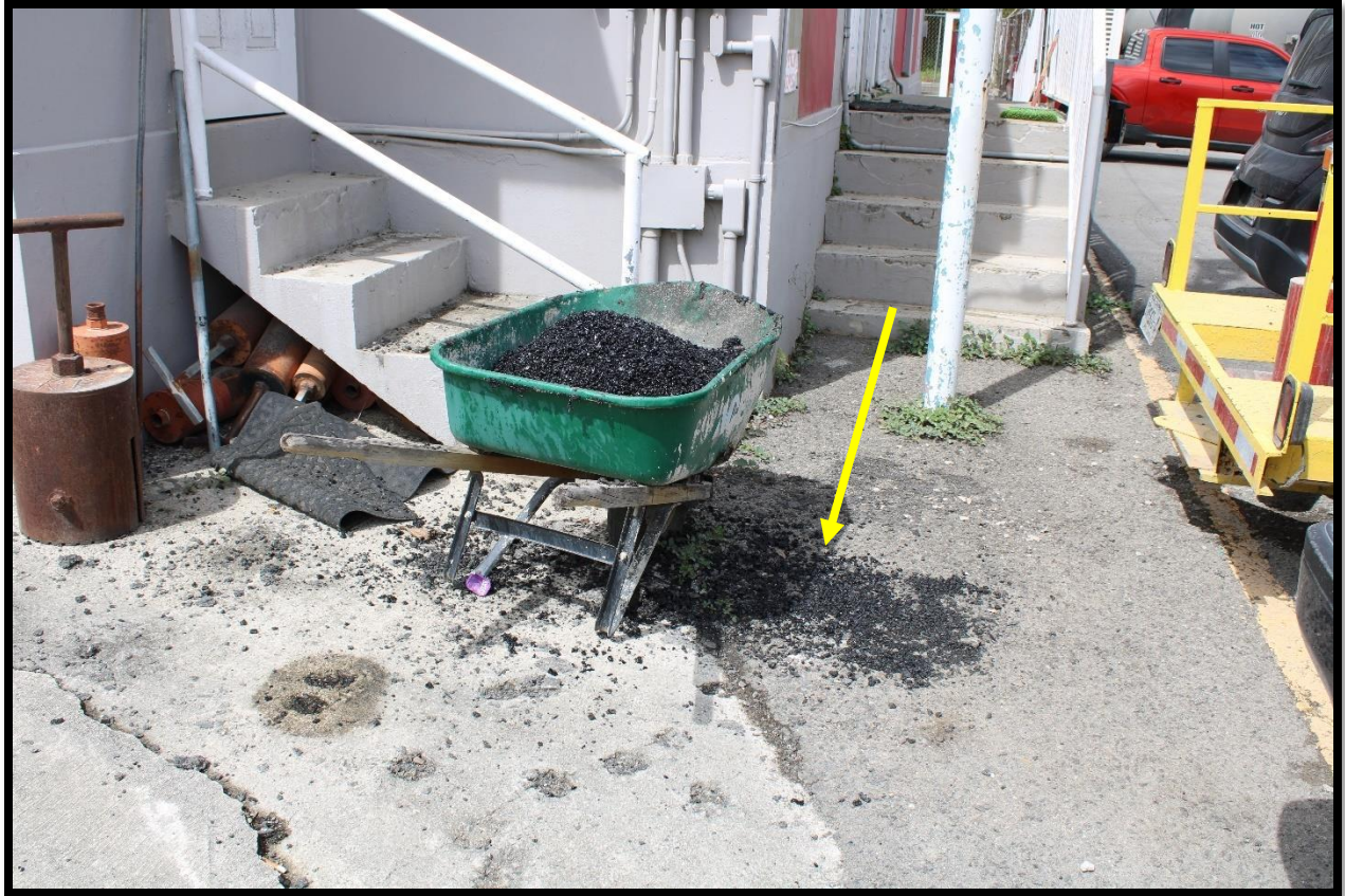
Picture 13 shows an asphalt concrete spill (yellow arrow). No organized housekeeping measures were evident in these areas.
