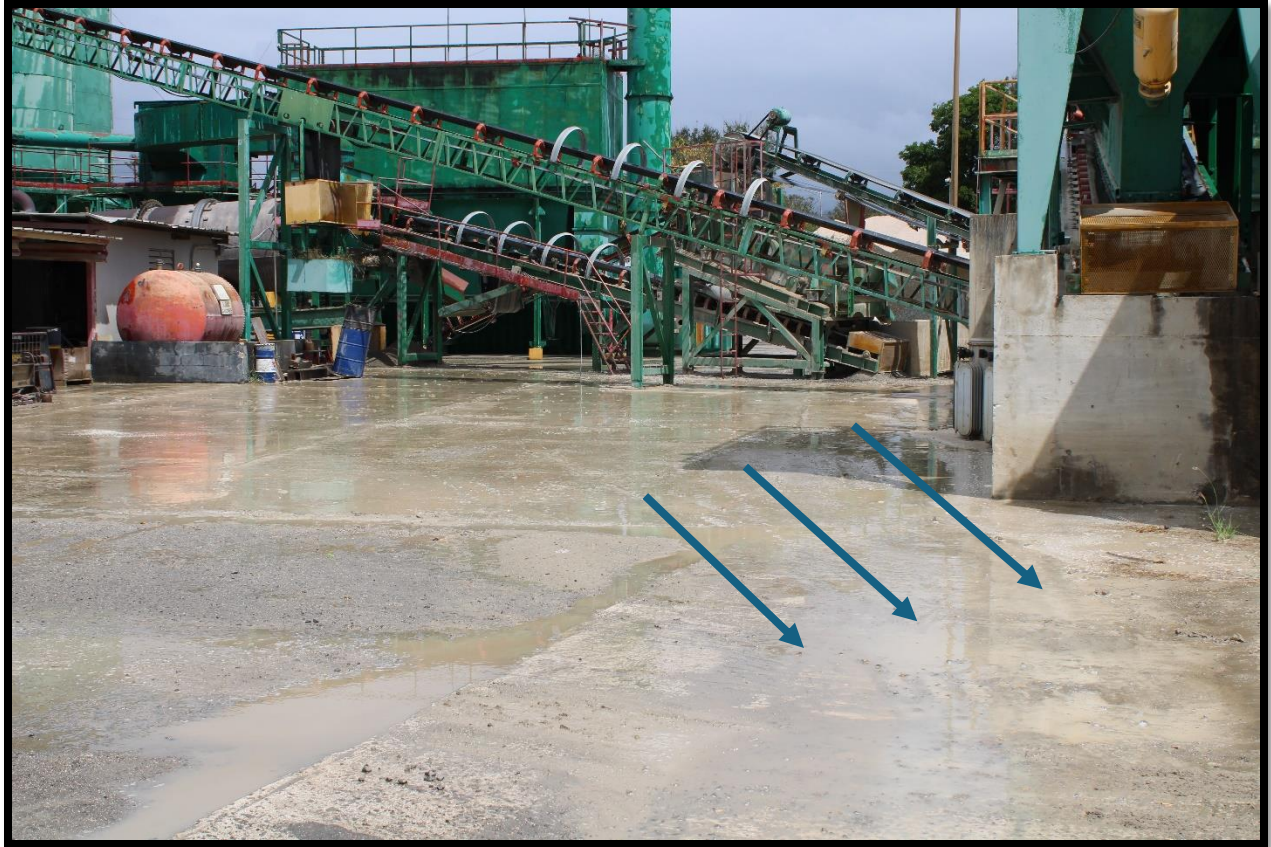
Picture 2 shows the asphalt cement processing plant and stormwater runoff flowing towards the storm sewer drain inlet shown in the previous picture. The blue arrows depict the flow path of stormwater runoff.
