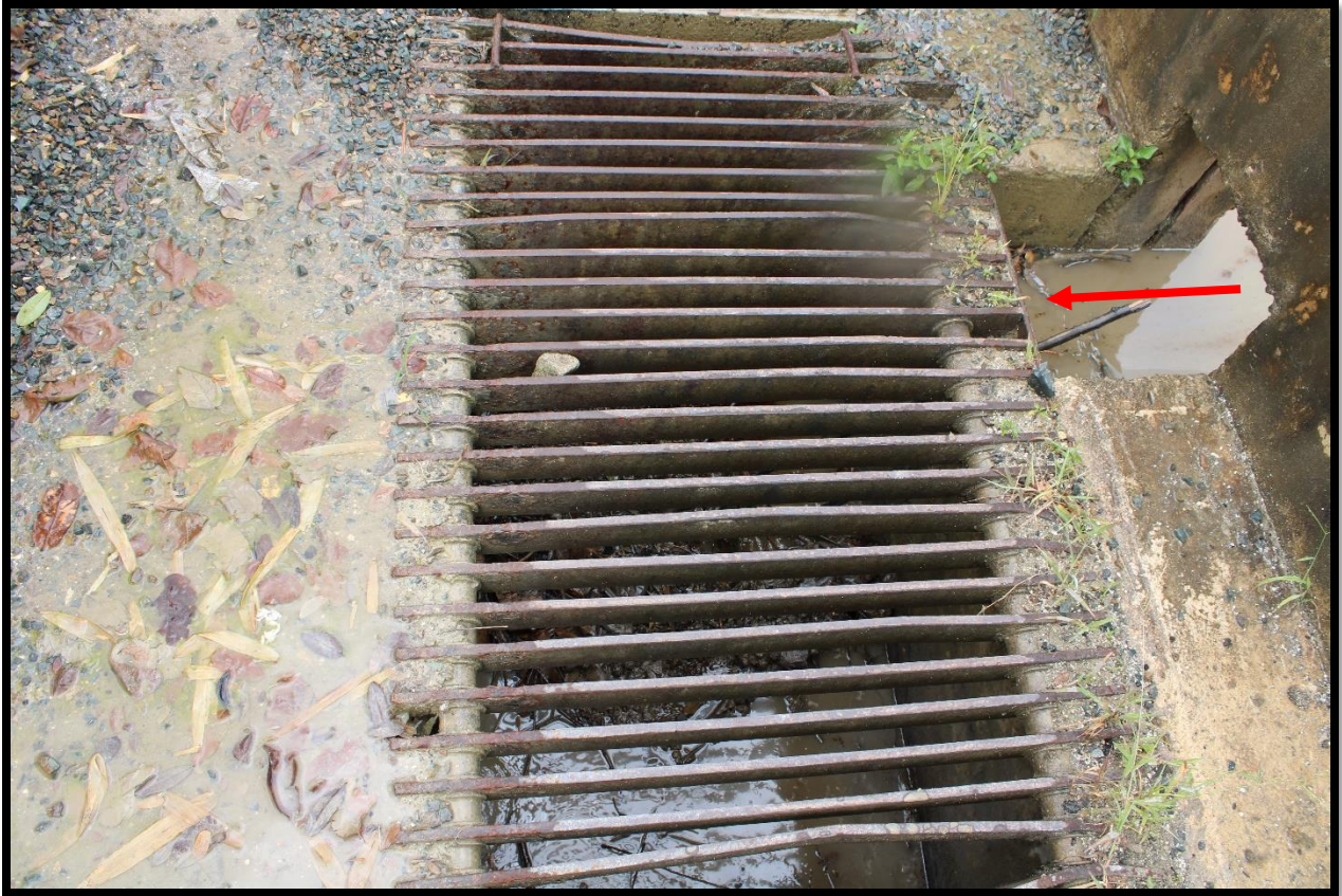
Picture 16 shows the storm sewer drain inlet located in the vehicle washing area. The inlet lacked a protection measure. Also, water containing oil was observed flowing the washing area into the inlet (indicated by the red arrow).
