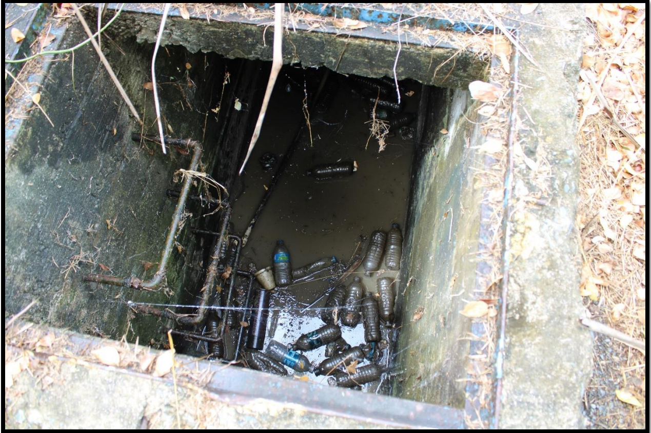
Picture 11 shows a buildup of plastic bottles found inside a storm drain inlet located in the aggregate storage area. The accumulated water is turbid and had a light brown color. The inlet lacked protection.
