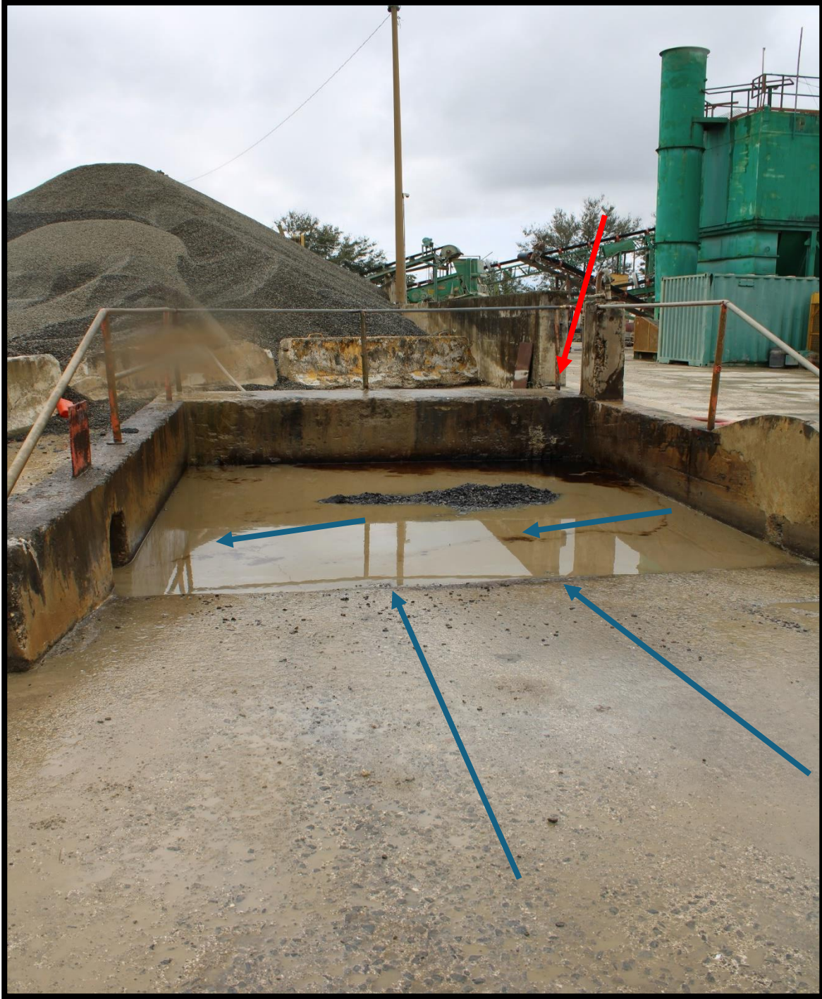
Picture 14 shows an oil spill (indicated by the red arrow) that reached the vehicle washing area. The water in the washing area had oil and was observed flowing into a concrete drainage. The blue arrows indicate the flow path of stormwater runoff into the washing area. Also, they show the flow path into the concrete drainage.
