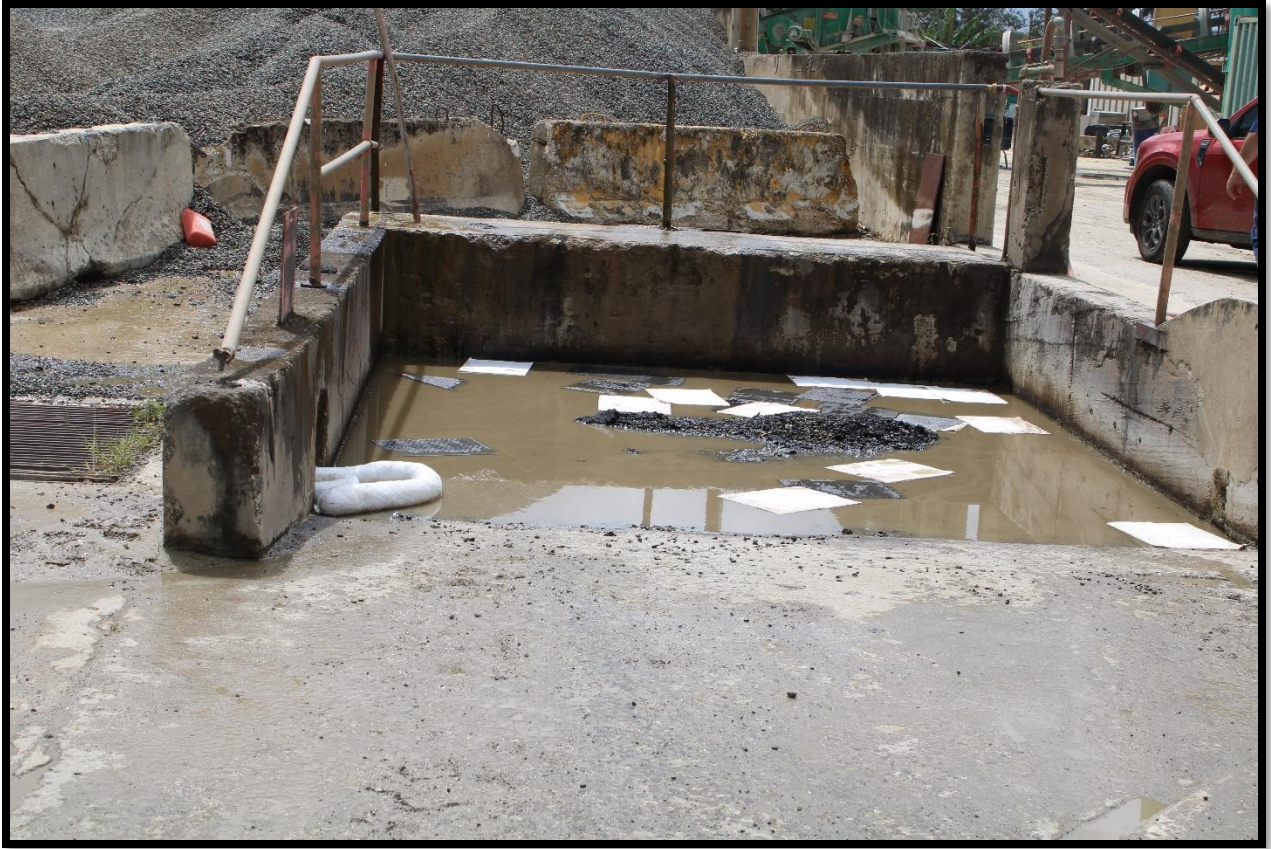
Picture 15 shows the corrective measure implemented by the facility staff at the washing area.
