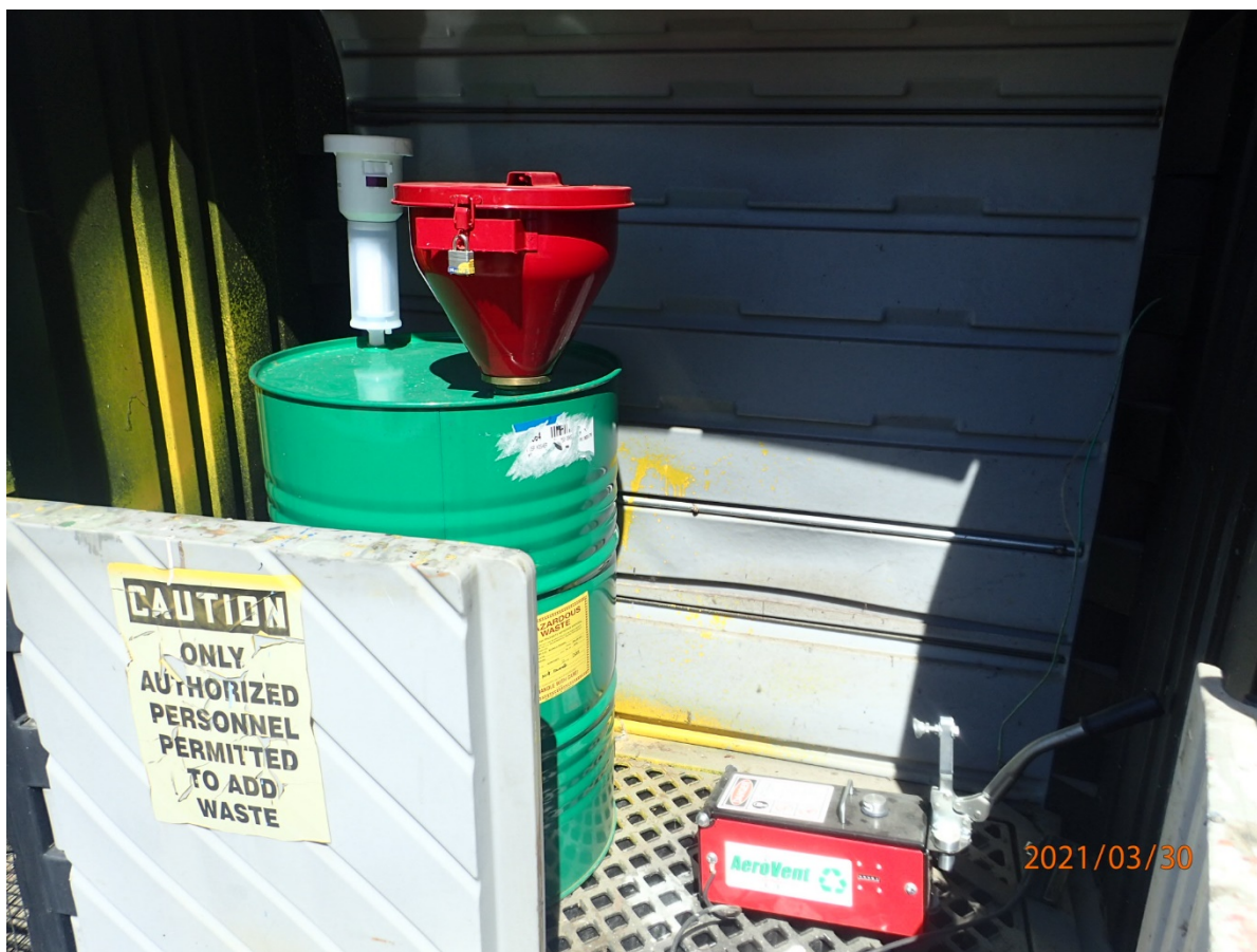
Photo 21: SAA – 55-gal drum labeled D001 Hazardous Waste Used Paint. Magnolia Plant.
