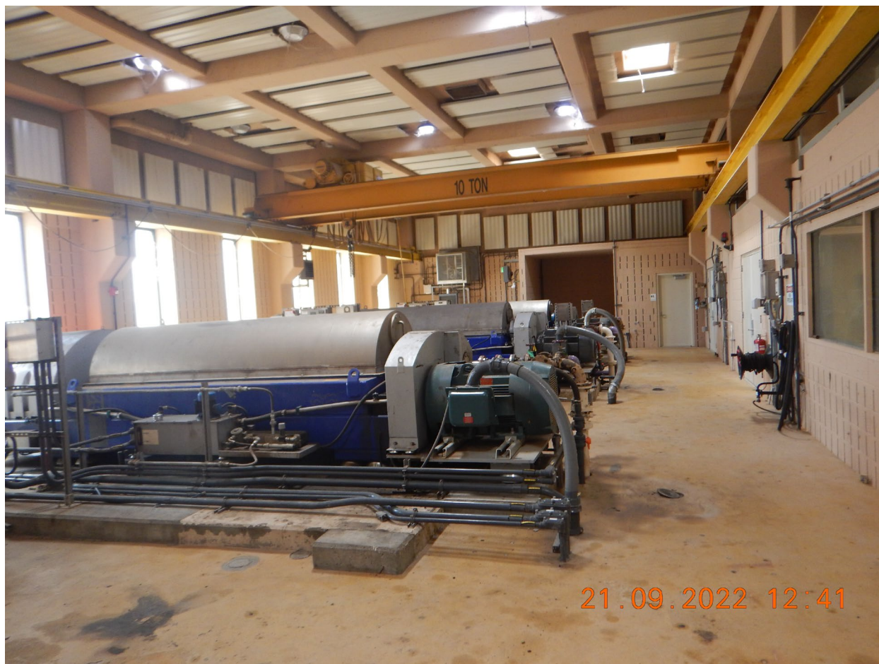
View of several centrifugal drums utilized in the thickening and dewatering of the sludge. (DSCN2326) Photographed by D. Esparza
