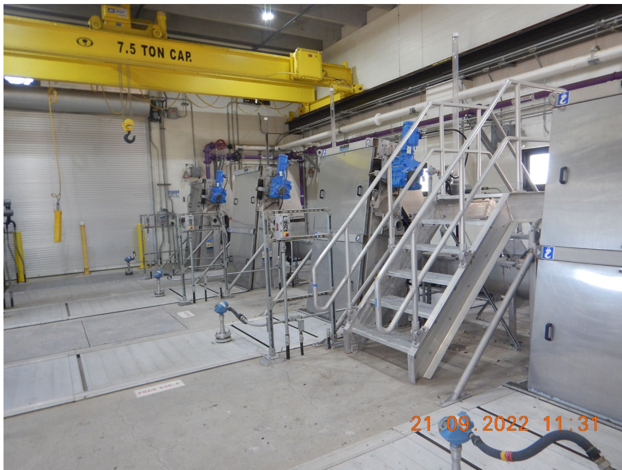
View of process treatment equipment inside the Course Screening Facility (CSF). (DSCN2320) Photographed by D. Esparza
