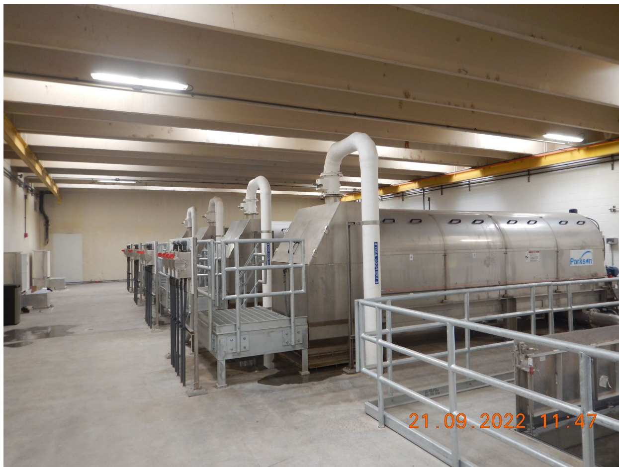
View of process treatment equipment inside the Rotating Drum Thickener Facility (RDT). (DSCN2321) Photographed by D. Esparza
