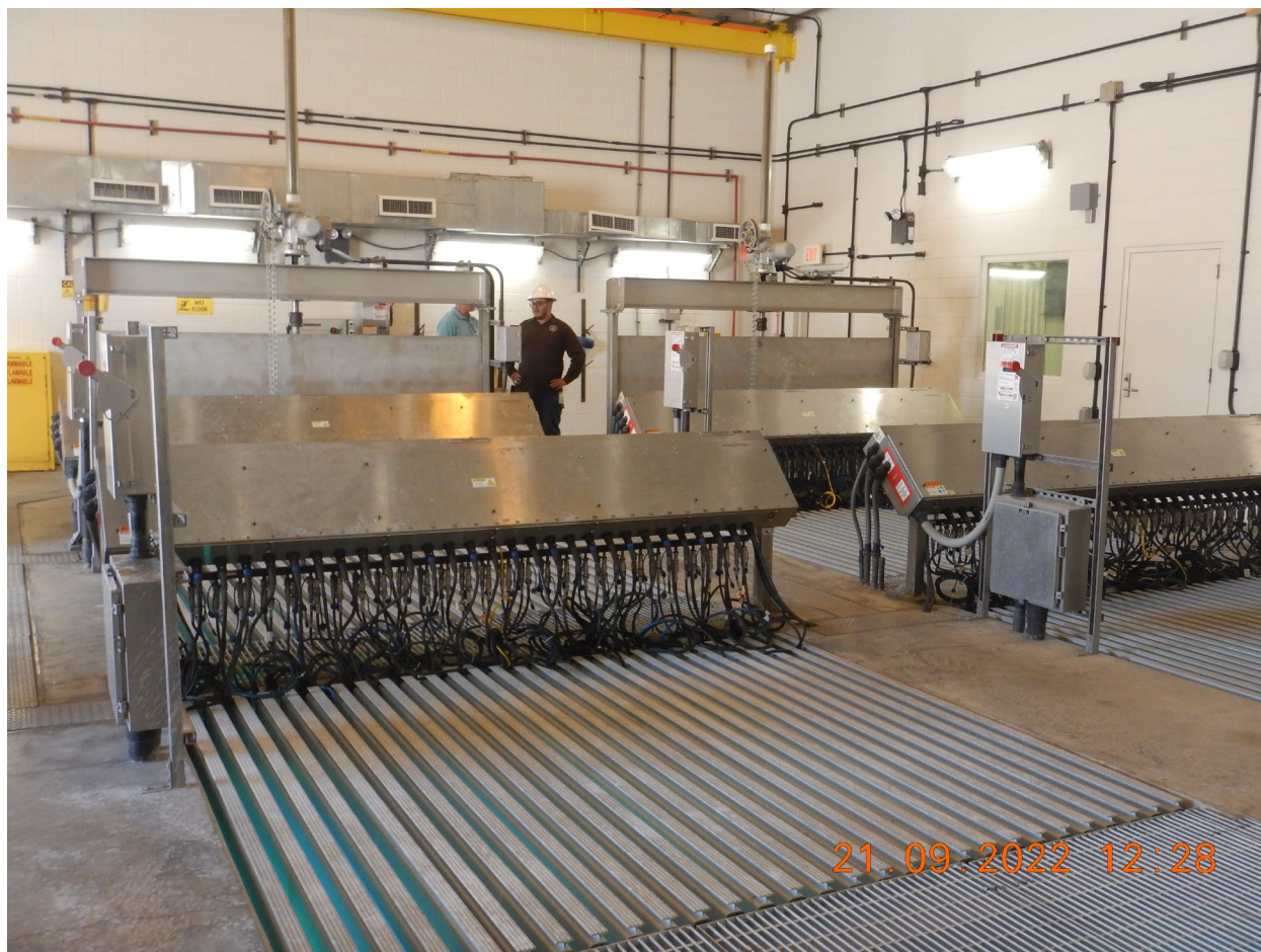
View of ultra-violet (UV) disinfection banks inside the UV Disinfection Building before the Siphon Towers and the eventual discharge to the Rio Grande at Outfall 001. (DSCN2324) Photographed by D. Esparza
