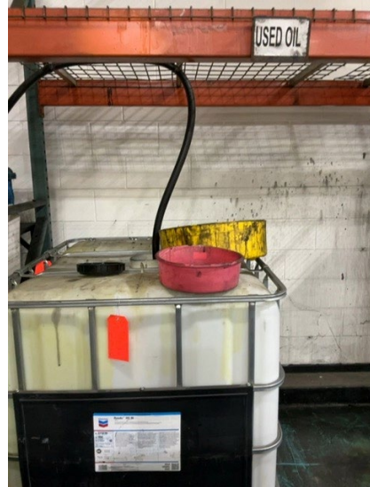
Photo 6: 250-gal tote with used oil. Container is not labeled “Used Oil”.
