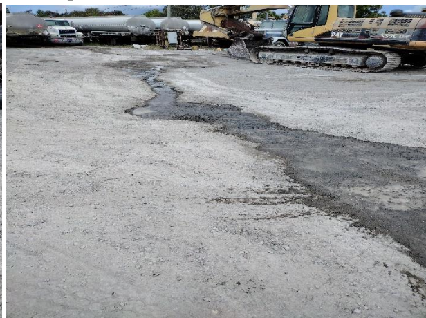
IMG 6639 -Dry-weather flow draining along the ground towards the northwestern corner of the Facility.
