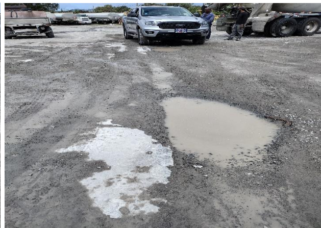
IMG 9313 -Continuation of dry-weather flow going into central section of the Facility, before draining to towards the lower entrance and into the road.
