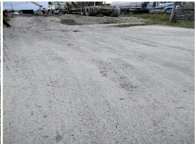
IMG 2419 -Entrance/exit into product loading bay. Ready-mixed concrete residues cover the pavement, and exposed to all environmental conditions.
