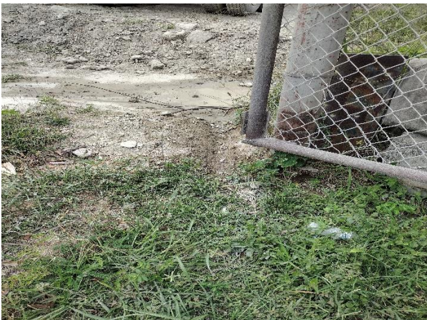
IMG 2968 -Close-up view of drainage point where ready-mixed concrete, wash water and stormwater runoff flow drains-off at end of installed berm.
