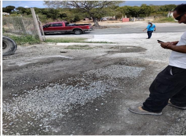
IMG 6690 -Product loading bay and flow path into Outfall 1. Ready-mixed concrete residues, exposed to storm water runoff.
