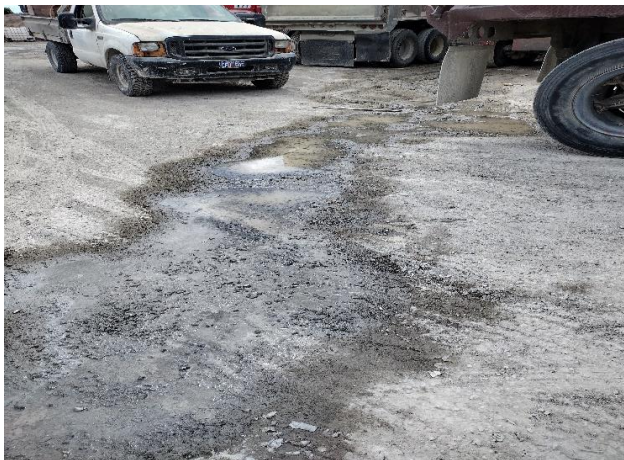
IMG 6346 -Dry-weather flow draining from central Section and towards northwest corner of Facility.
