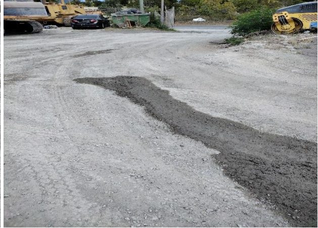
IMG 9755 -Evidence of dry-weather flow draining to the lower entrance (Outfall 2) captured during the 2023 Inspection.
