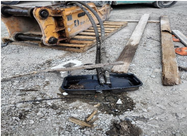
IMG 0136 -Close-up view of equipment repair occurring in the open. Spilled oil-based fluid onto ground.
