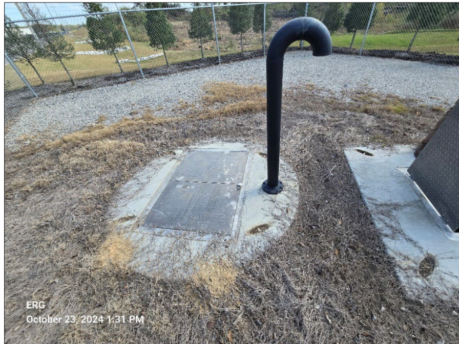
Photograph 14. Legacy Park East lift station.
