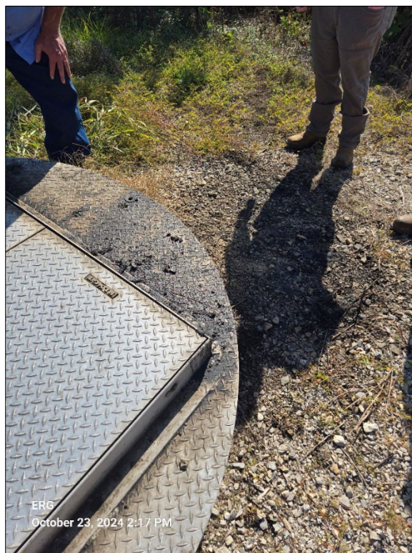
Photograph 23. Oil residual and/or evidence of overflow by the wet well at High Point lift station.
