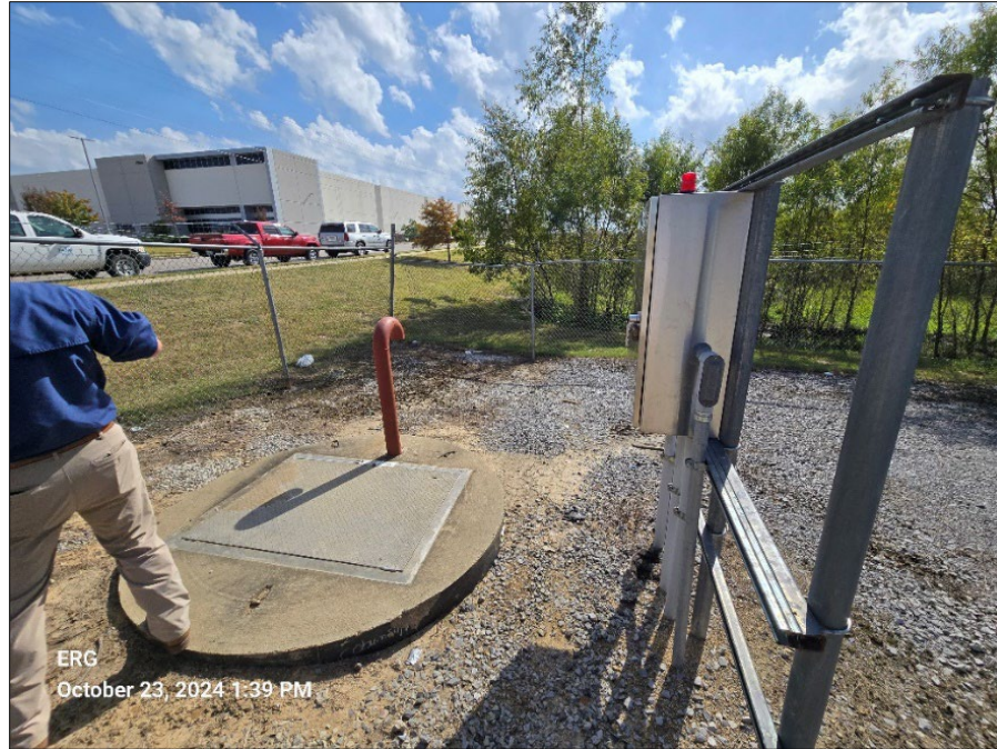
Photograph 17. Legacy Park North lift station.
