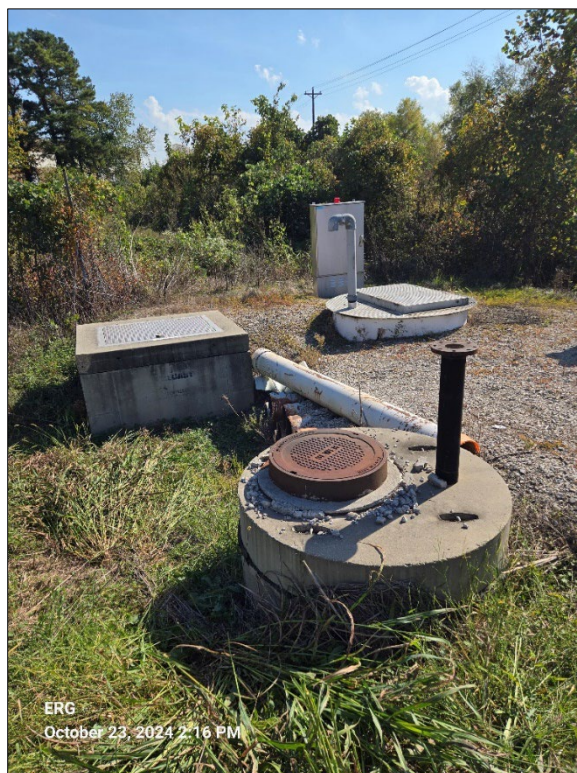
Photograph 22. High Point lift station. Note the valve pit and wet well were not locked.
