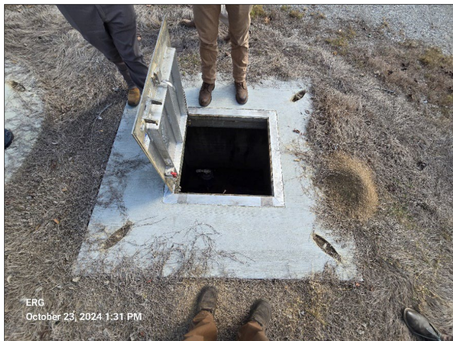
Photograph 15. Legacy Park East lift station wet well.
