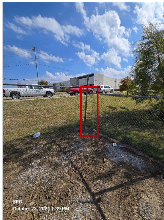
Photograph 18. Legacy Park North lift station perimeter fencing. Note the gap in the fence, outlined in red.
