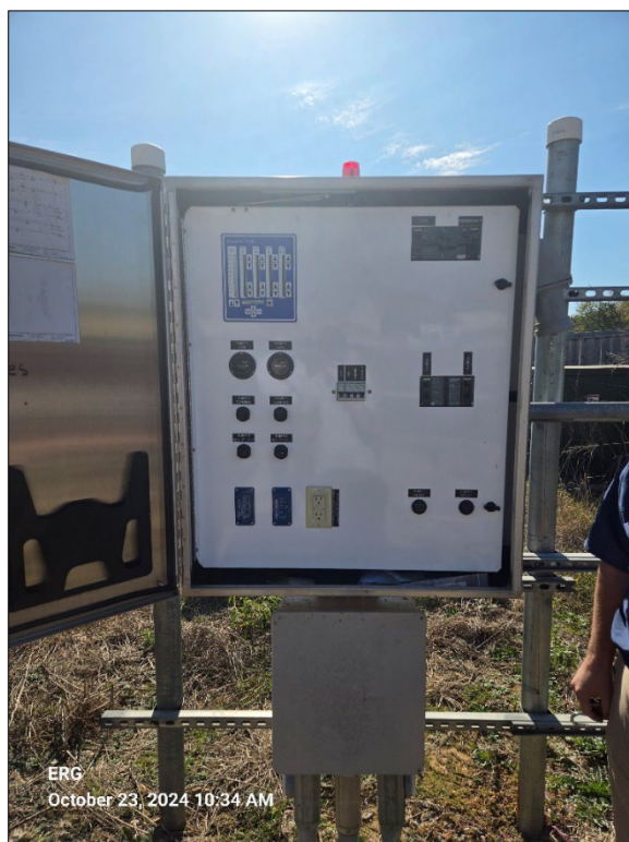
Photograph 2. McElroy Farms lift station pump control panel.
