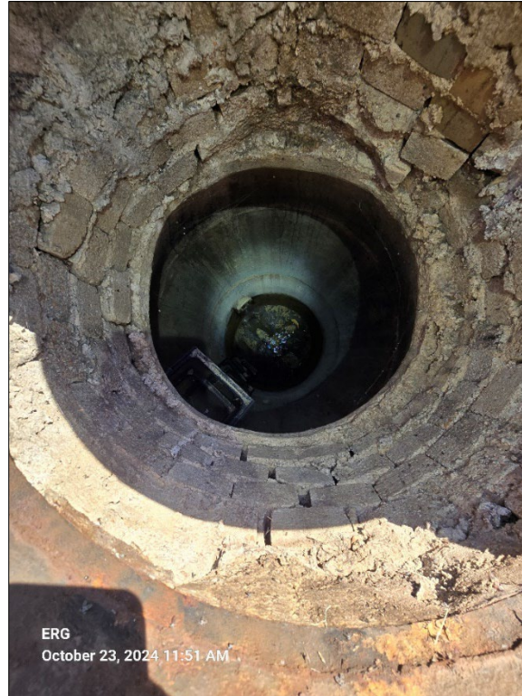
Photograph 13. Interior of the manhole at Braybourne & Sandbourne. Note the small solids and grease accumulation in the manhole.
