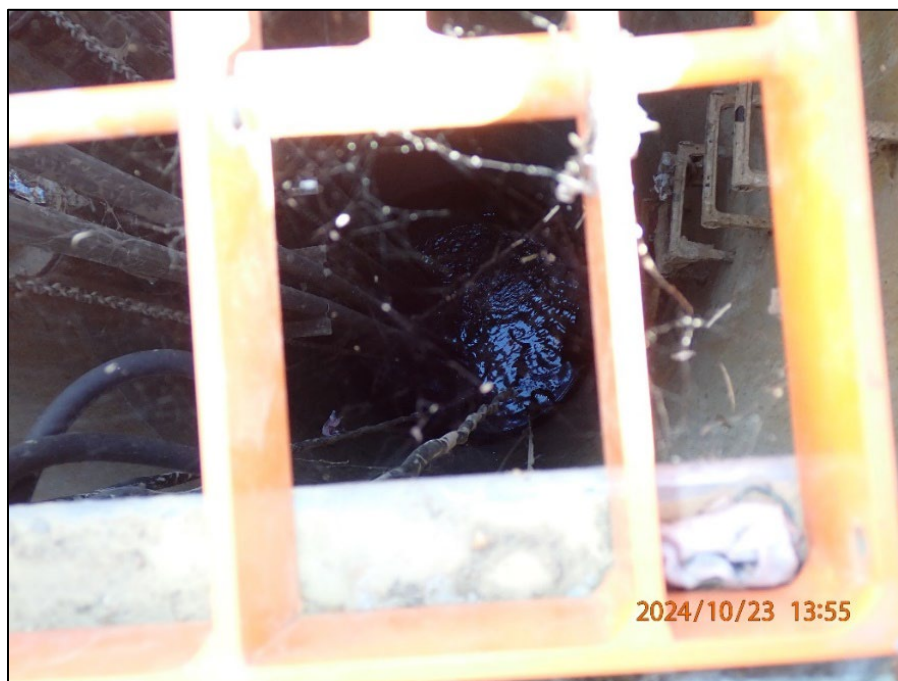
Photograph 21. Legacy Park North lift station wet well.
