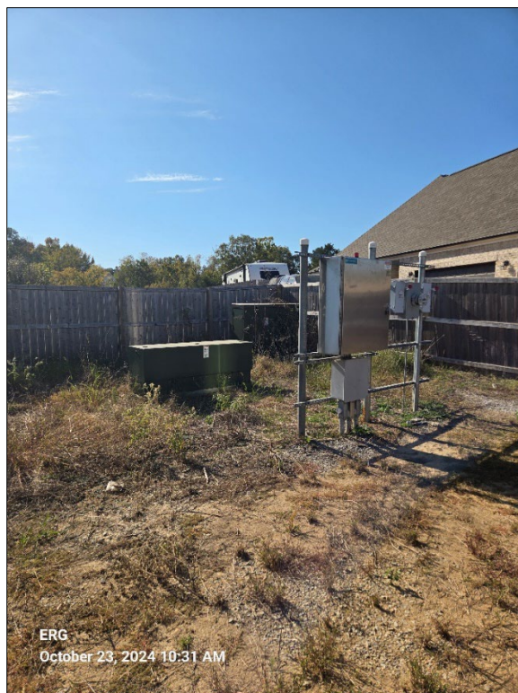
Photograph 1. McElroy Farms lift station. Note the excessive vegetation around the lift station.
