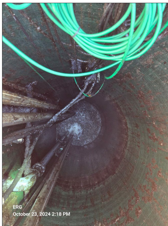
Photograph 24. High Point lift station wet well. Note the black fluid and black solids in the wet well.
