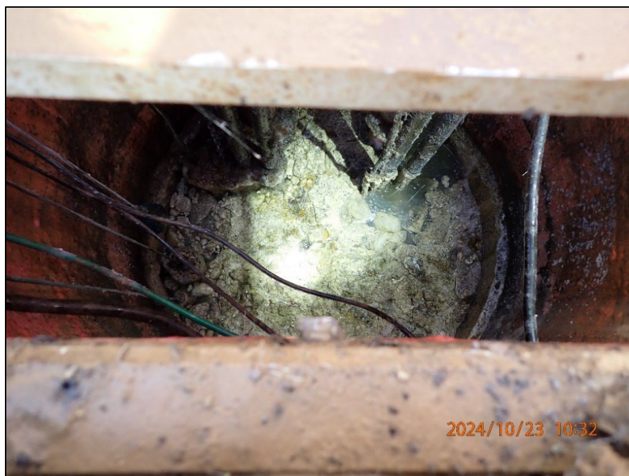
Photograph 3. McElroy Farms lift station wet well. Note the grease accumulation.
