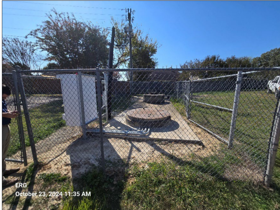
Photograph 9. Braybourne lift station.
