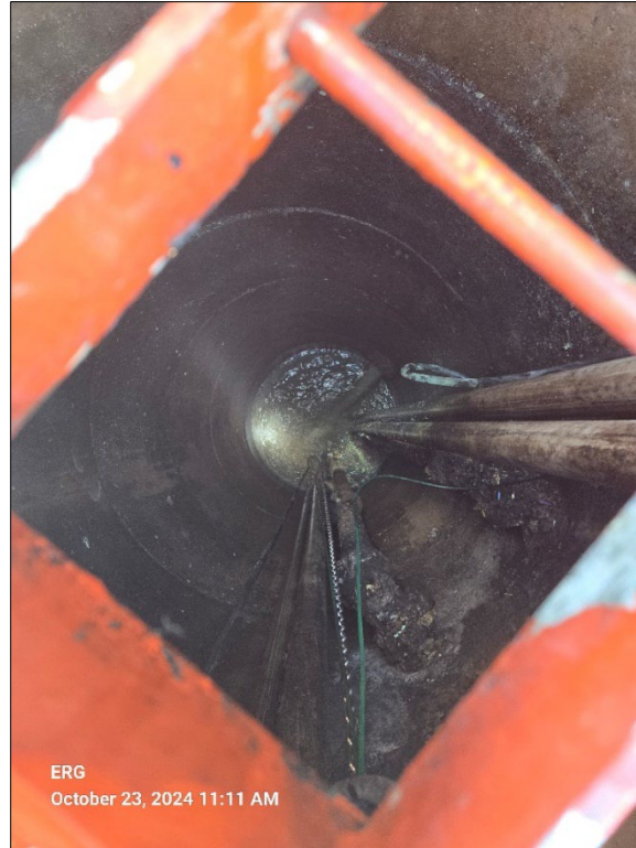
Photograph 7. Yahweh lift station wet well.
