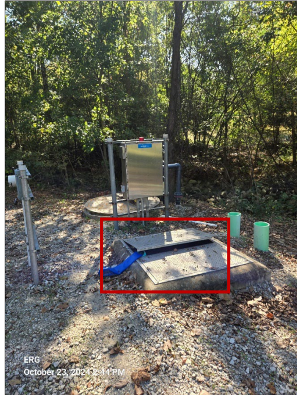
Photograph 25. East State Line lift station. Note one of the doors to the old valve pit (outlined in red) was open and not locked.
