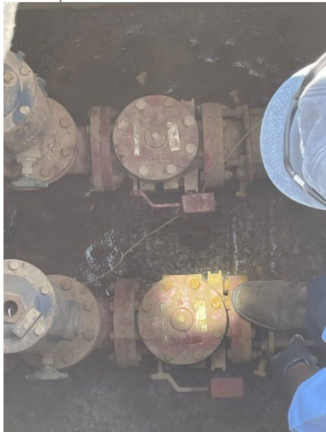
The High Point Lift Station was cleaned 10-25-24. As requested, cleaning frequency is being increased scheduled at least 3 times annually.
