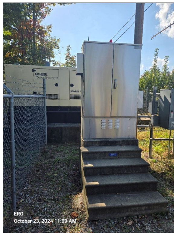
Photograph 6. Yahweh lift station. Note the pump control panel in the foreground and the Kohler onsite backup generator in the background of the photograph.
