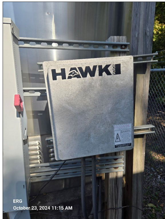
Photograph 8. Yahweh lift station local control system.
