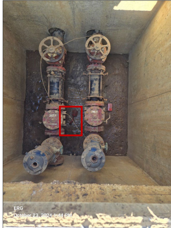
Photograph 19. Legacy Park North lift station valve pit. Note the counterweight (outlined in red) is disconnected for the left check valve.
