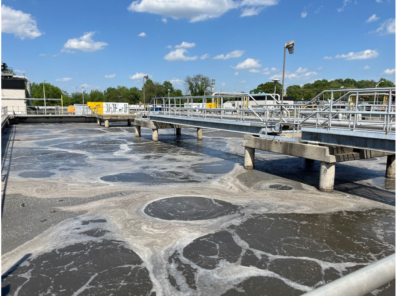
Photograph #5: Air rising unevenly, and dead zones were observed in the aeration chambers.
