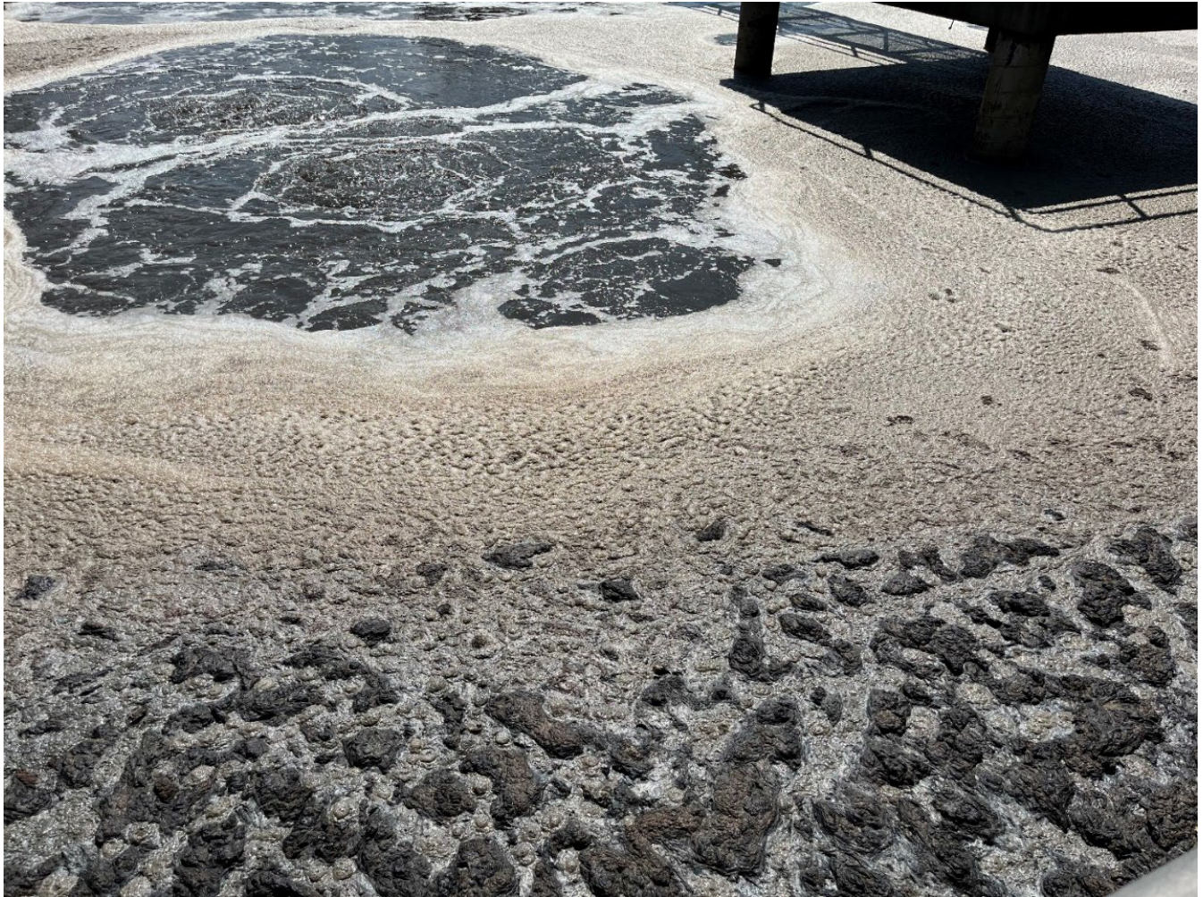
Photograph # 4: Dead zones were observed in the aeration chambers.
