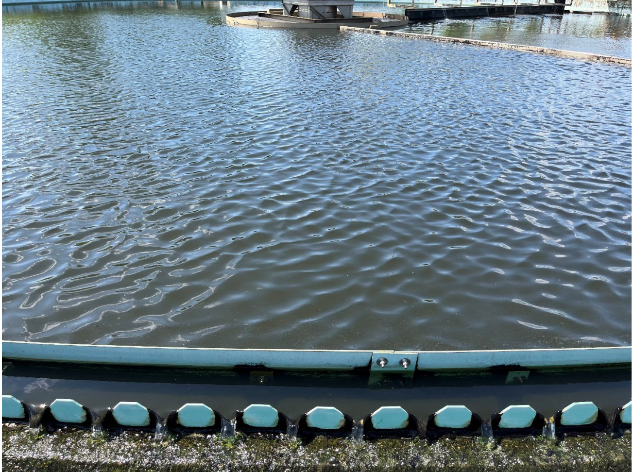
Photograph #6. Pin floc was observed overflowing the V-notch weirs from final clarifiers.
