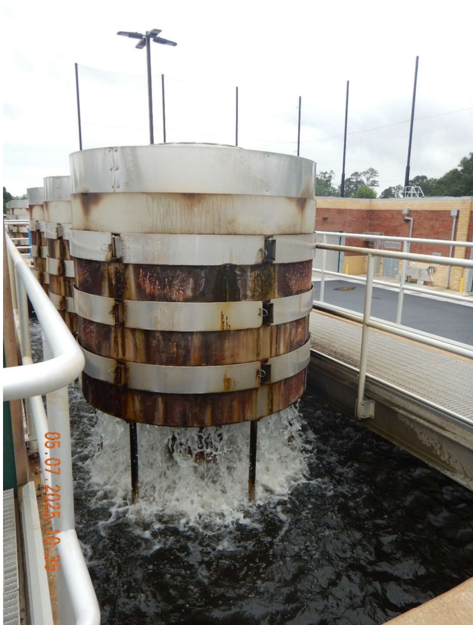
Aerators View of aerators.
