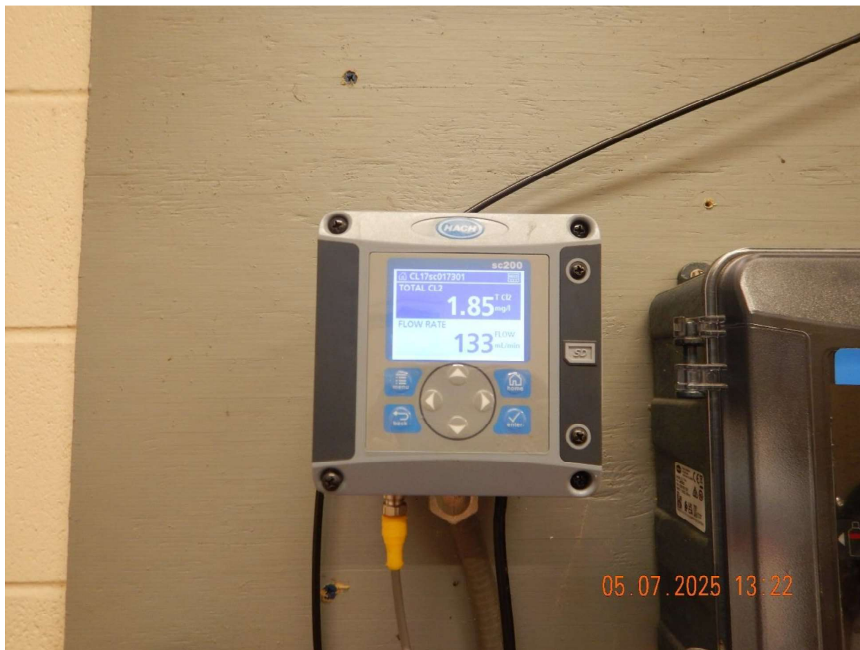
Chauvin Booster Station Total Chlorine residual reading and flow rate at Chauvin booster station.
