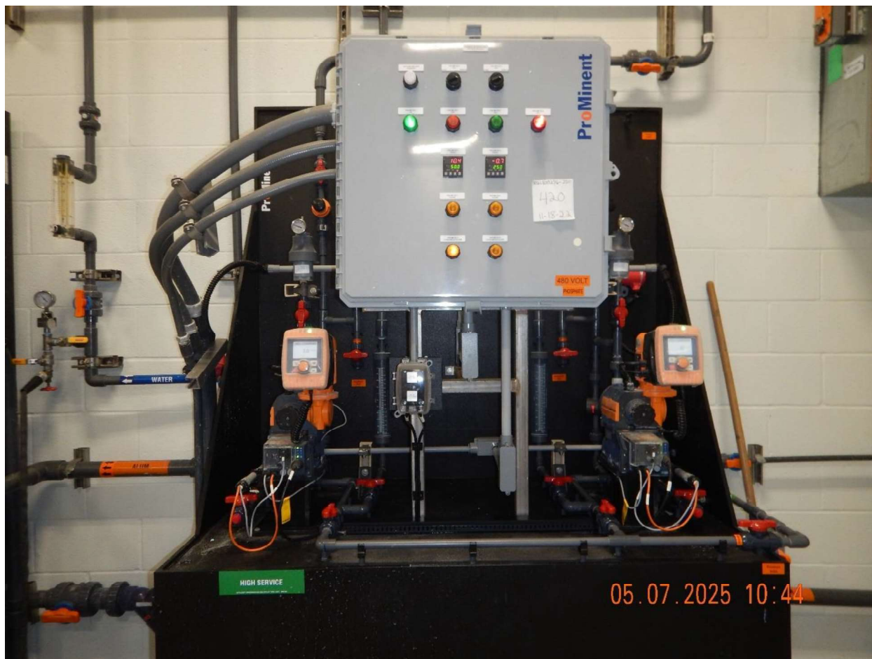
View of pumps View of chemical feed pumps for Aluminum Sulfate.
