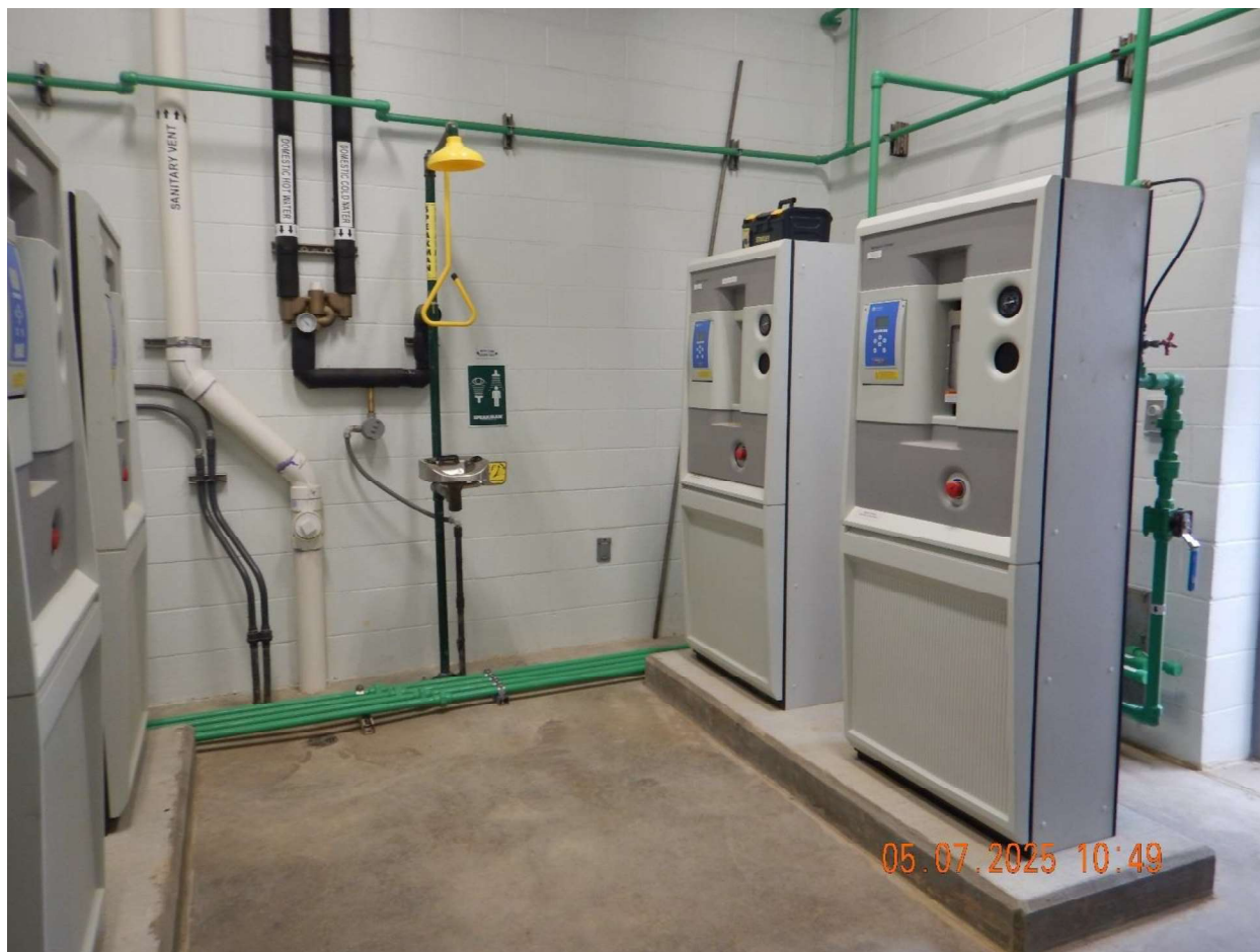
Ammoniators View of ammoniators and eyewash station.
