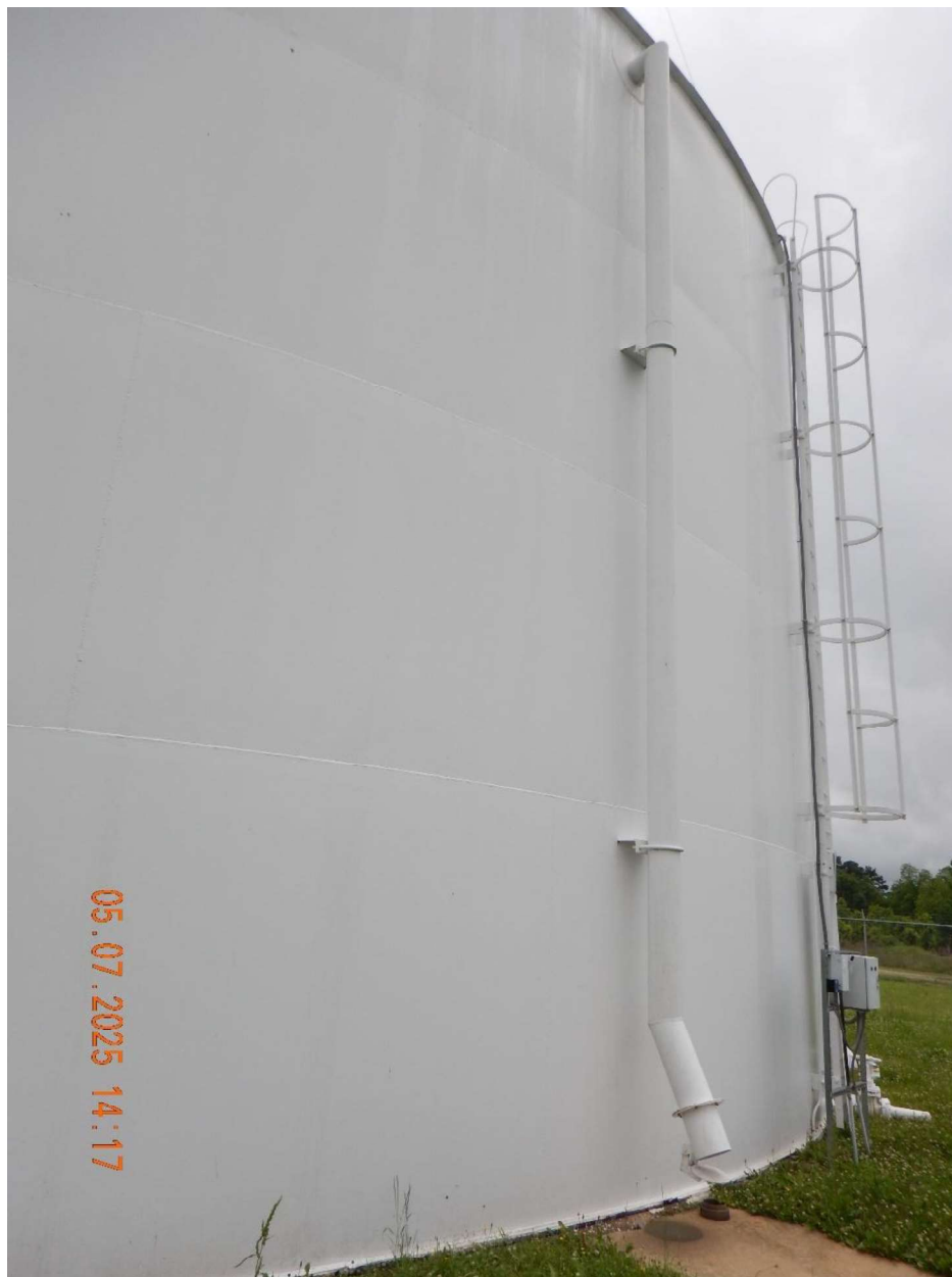
Thomas Tank View of overflow pipe at Thomas Tank.
