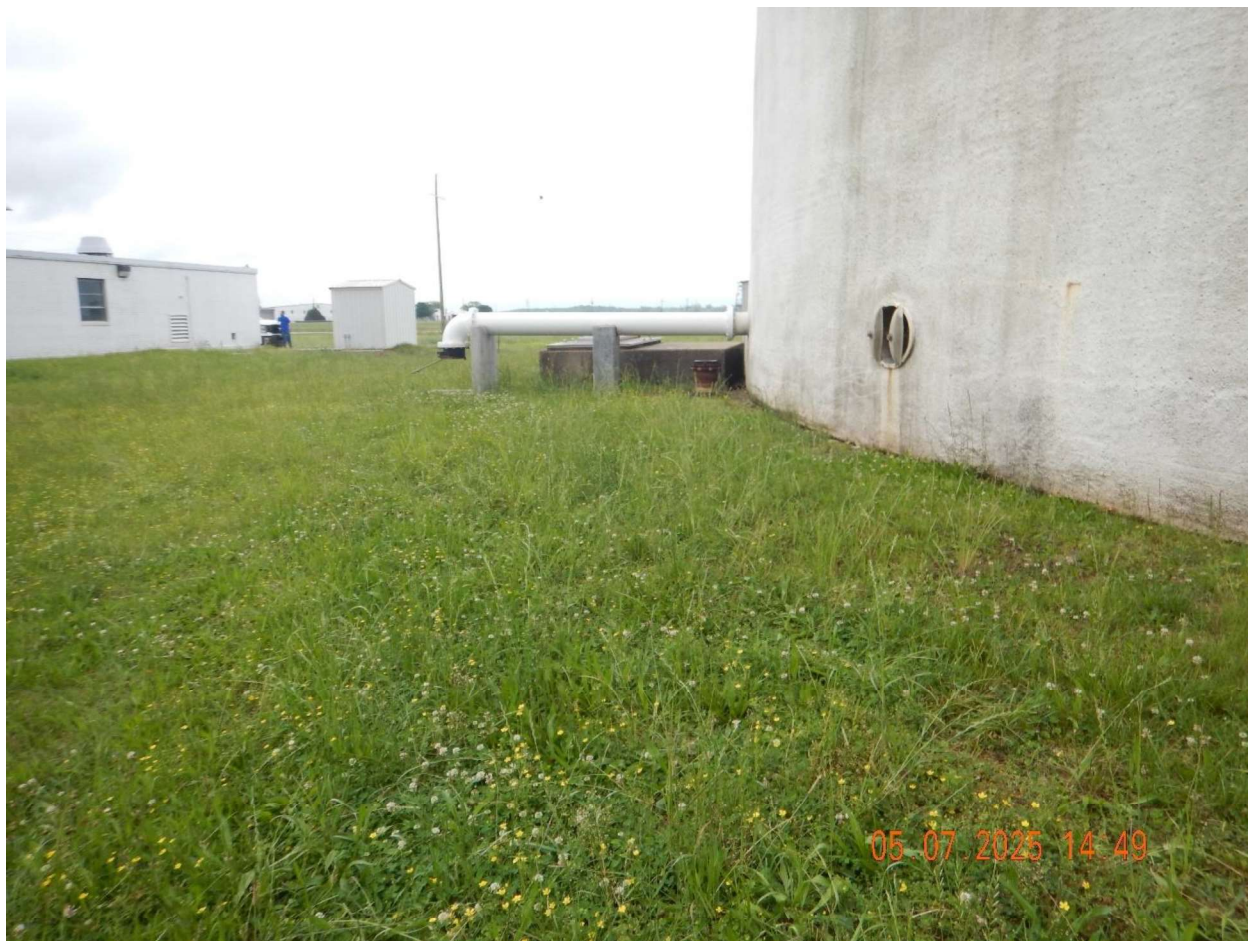
Overflow View of overflow pipe at Selman tank.
