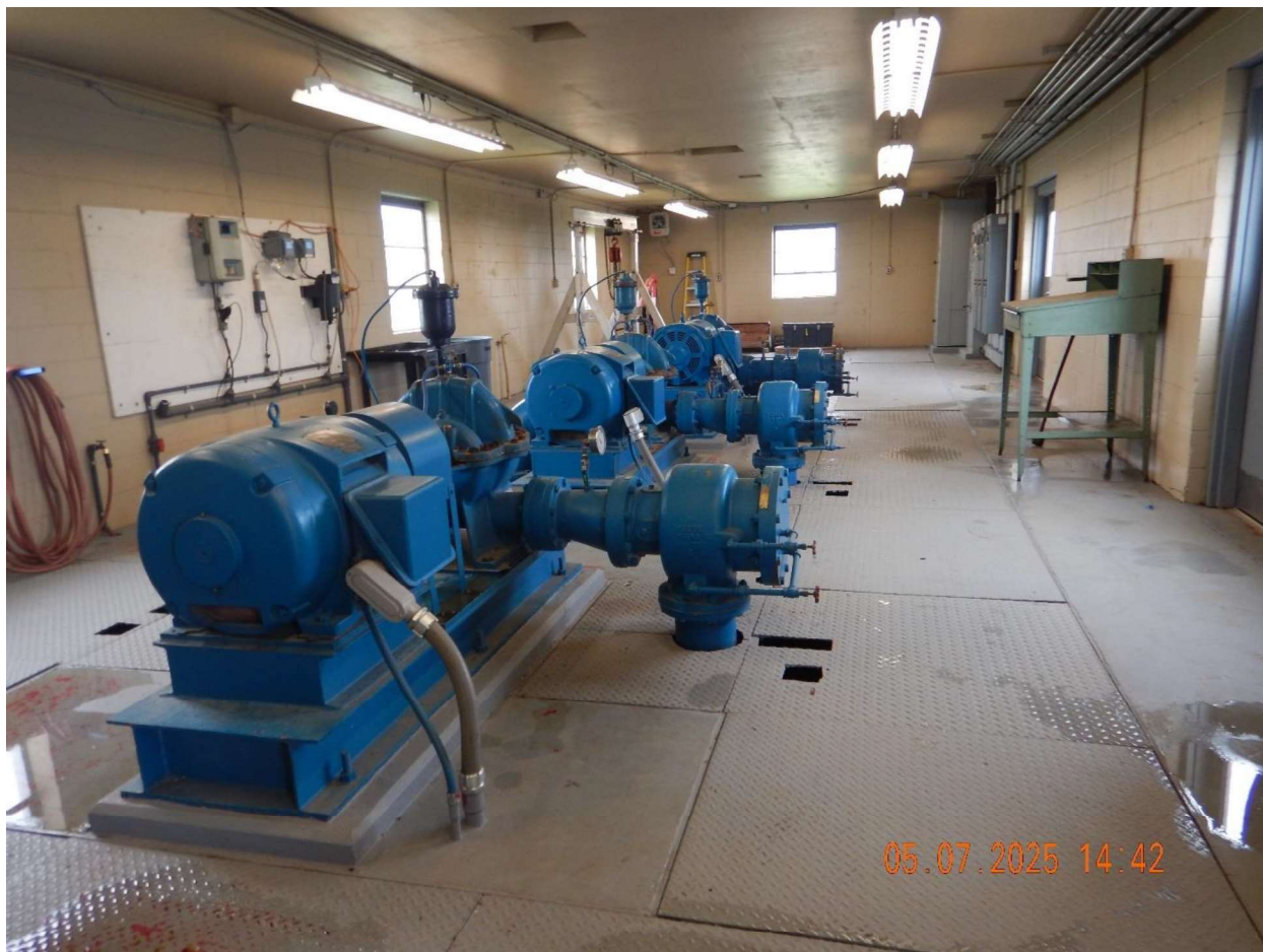
Thomas Booster Station View of pumps at booster station.
