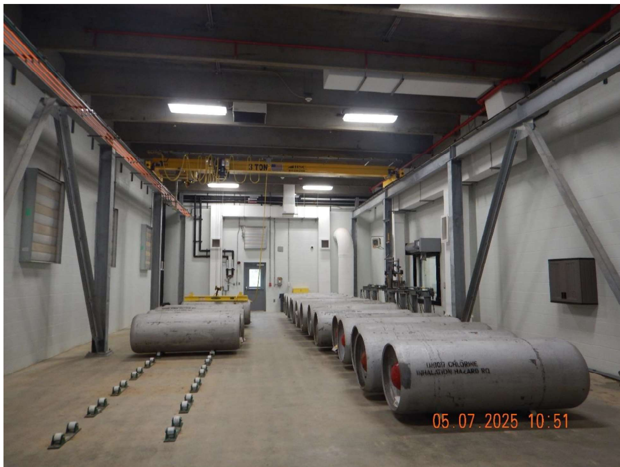
Chlorine Storage View of Chlorine gas tanks storage.
