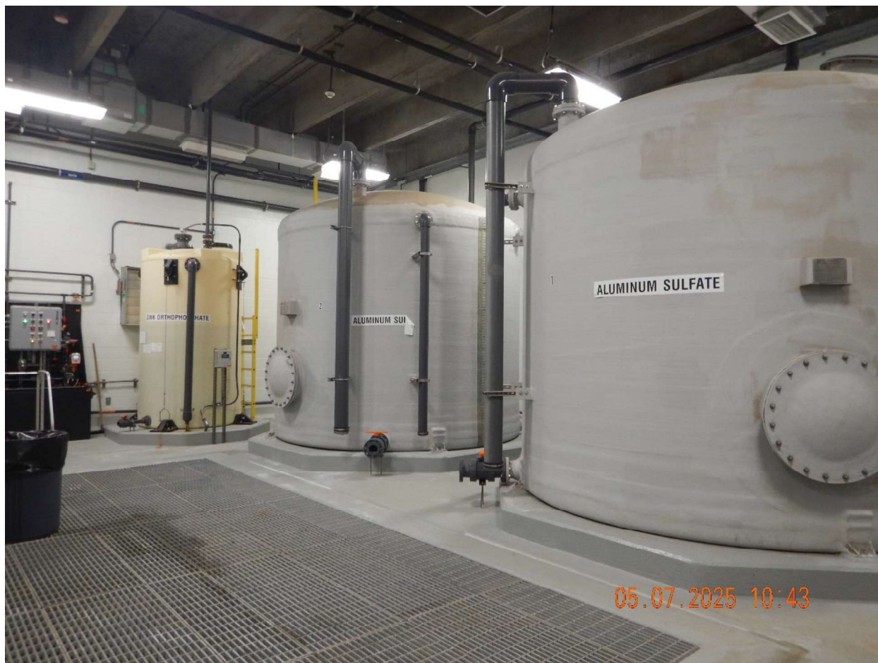
Alum Room View of Aluminum Sulfate and Zinc Orthophosphate tanks.
