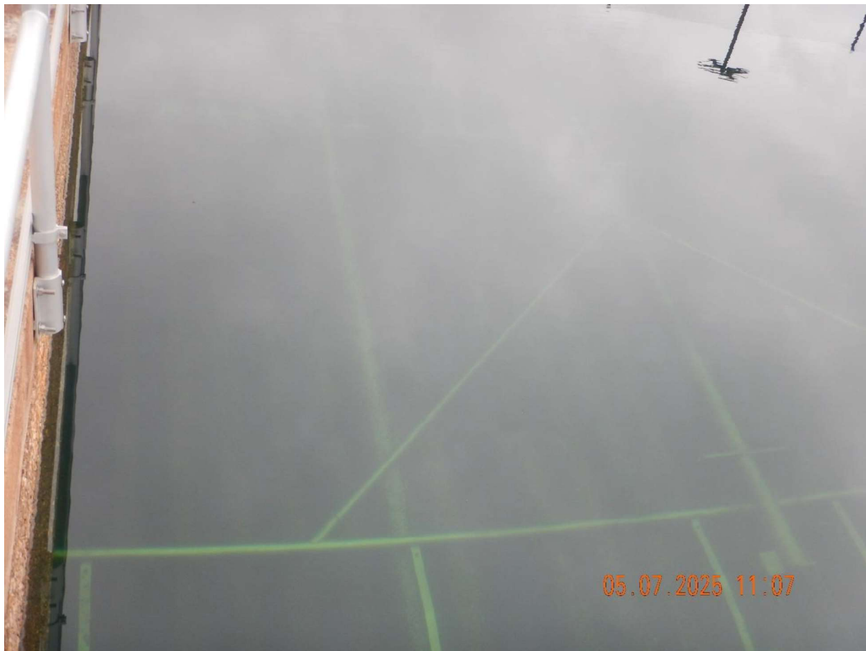
Flocculator View of walking beam flocculator.
