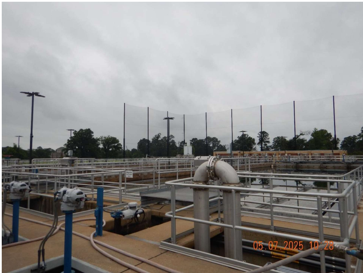
Water Treatment Plant Process View of sedimentation and flocculation basins.
