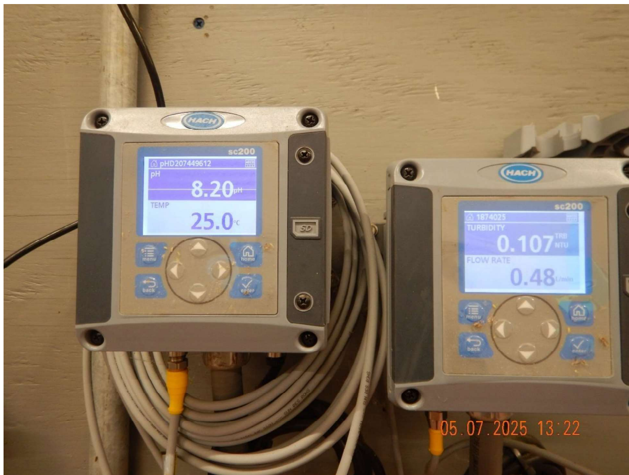
Chauvin Booster Station pH, temperature, turbidity, and flow rate readings at the Chauvin booster station.
