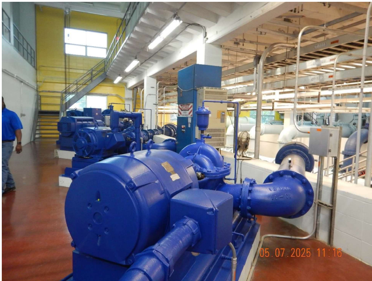
Pumps View of high service pumps.
