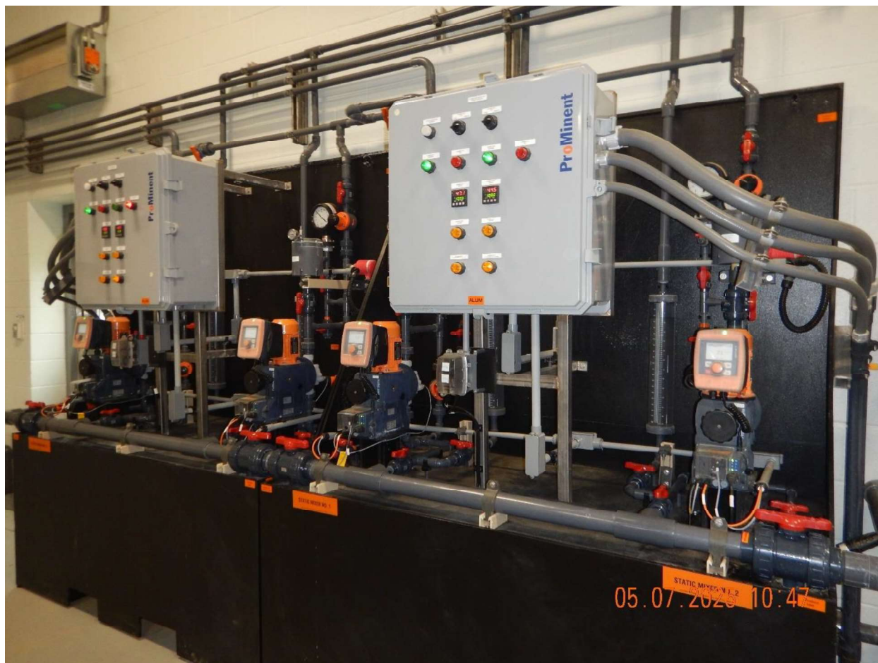
Chemical Feed Pumps View of chemical feed pumps for Aluminum Sulfate.
