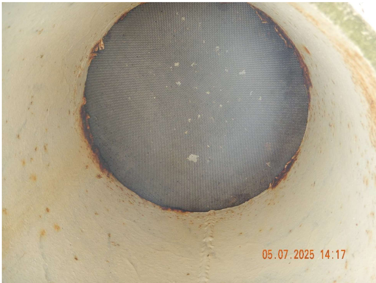
Overflow View of screened overflow pipe at Thomas Tank.
