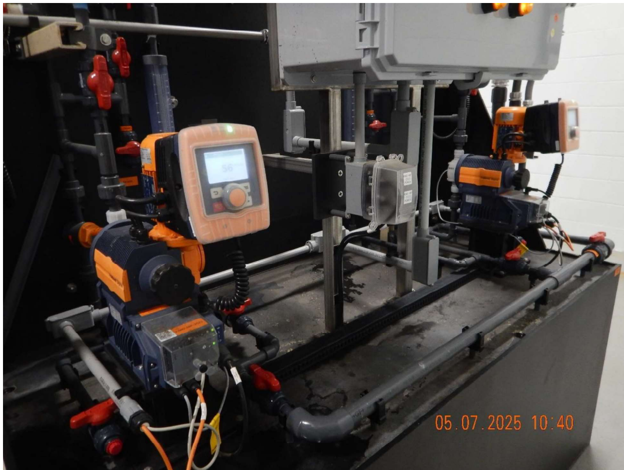
Chemical Feed Pumps View of chemical feed pumps for potassium permanganate.
