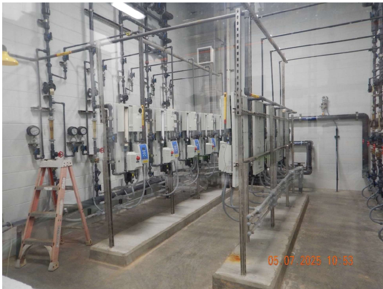
Chlorine Analyzers View of chlorine analyzers.
