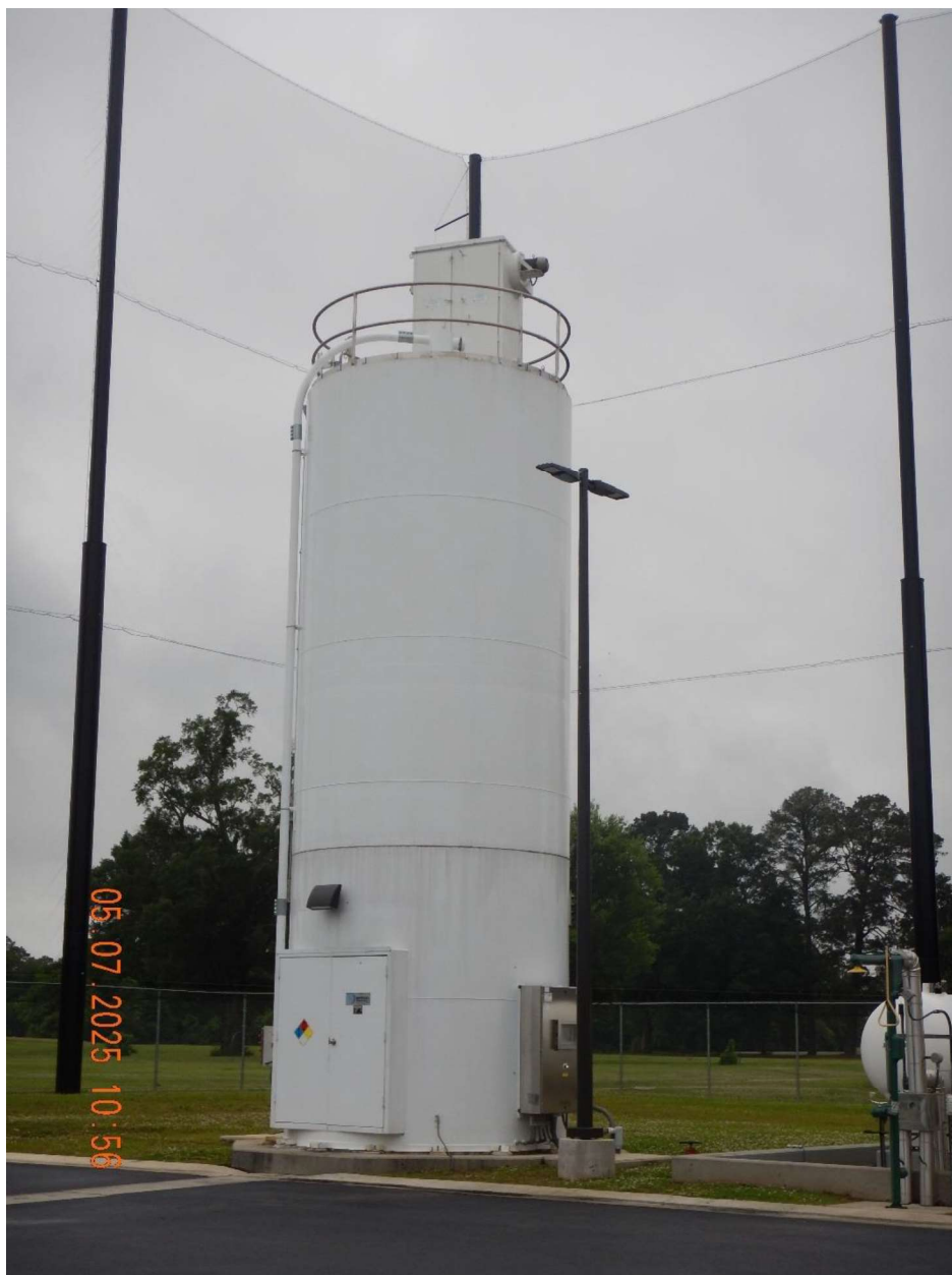
Activated Carbon Tank View of activated carbon tank.
