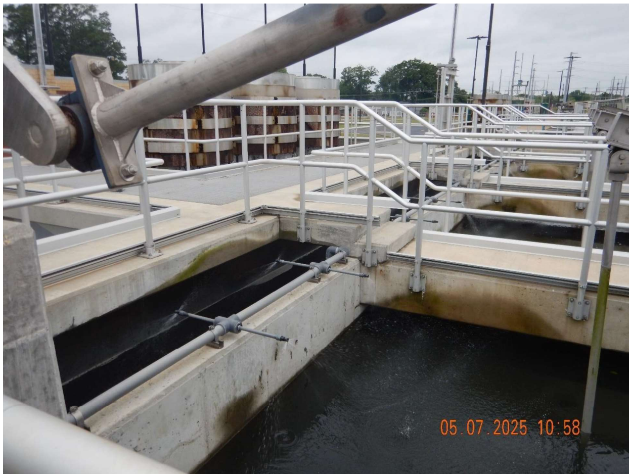
Static mixers View of static mixers.
