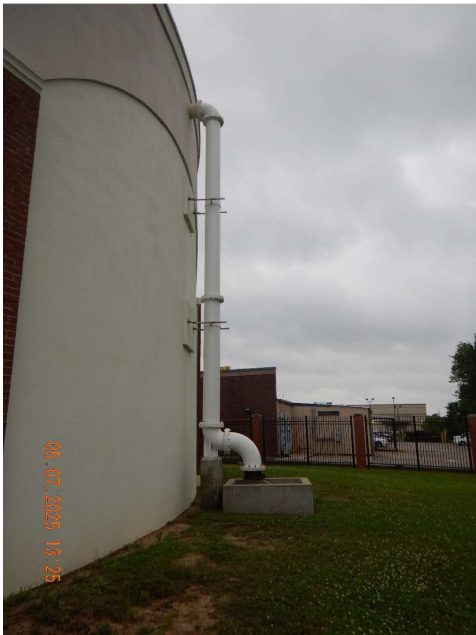
Chauvin Tank Chauvin tank overflow pipe.
