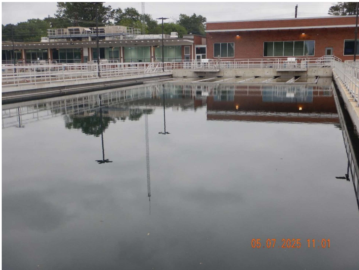
Sedimentation Basin View of sedimentation basin.
