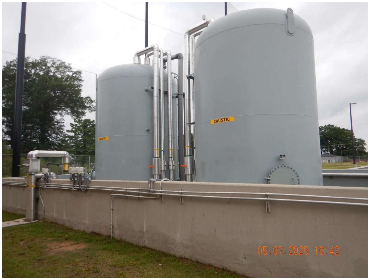
Bulk Tanks View of bulk tanks for caustic in secondary containment.
