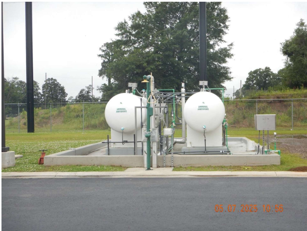
Ammonia Tanks View of ammonia tanks.
