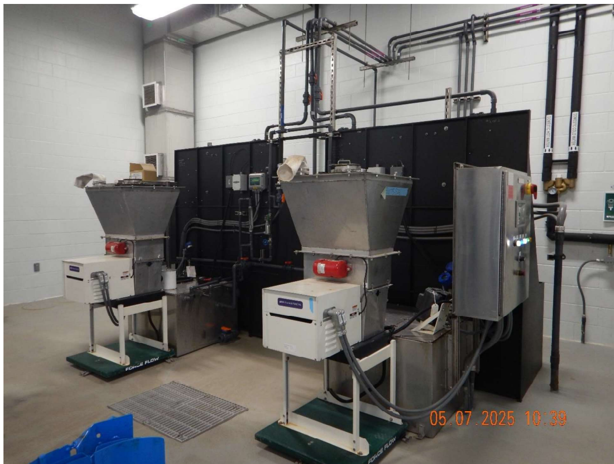
Potassium Permanganate Room View of Potassium Permanganate room.
