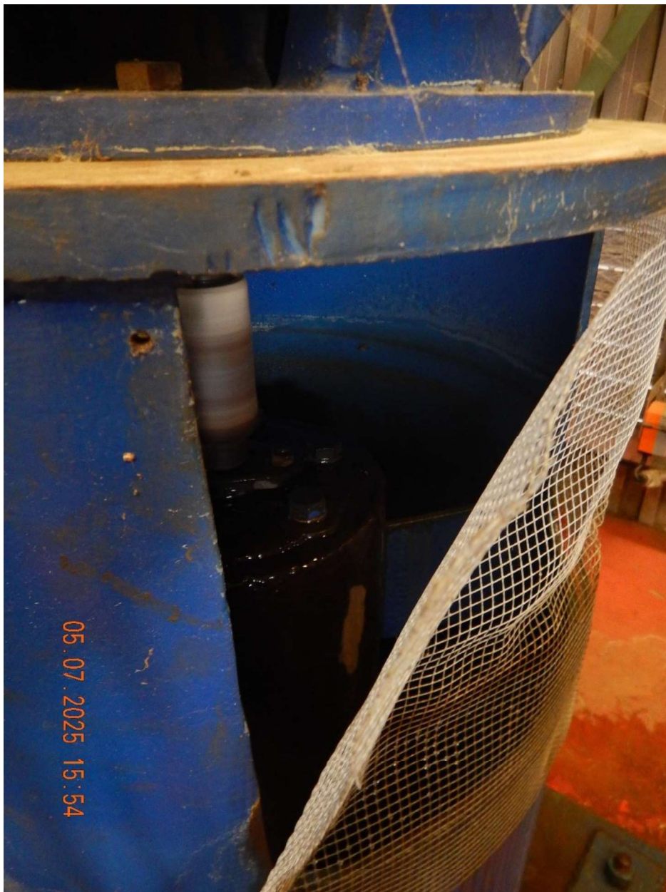
Pump 3 View of leak at pump 3.
