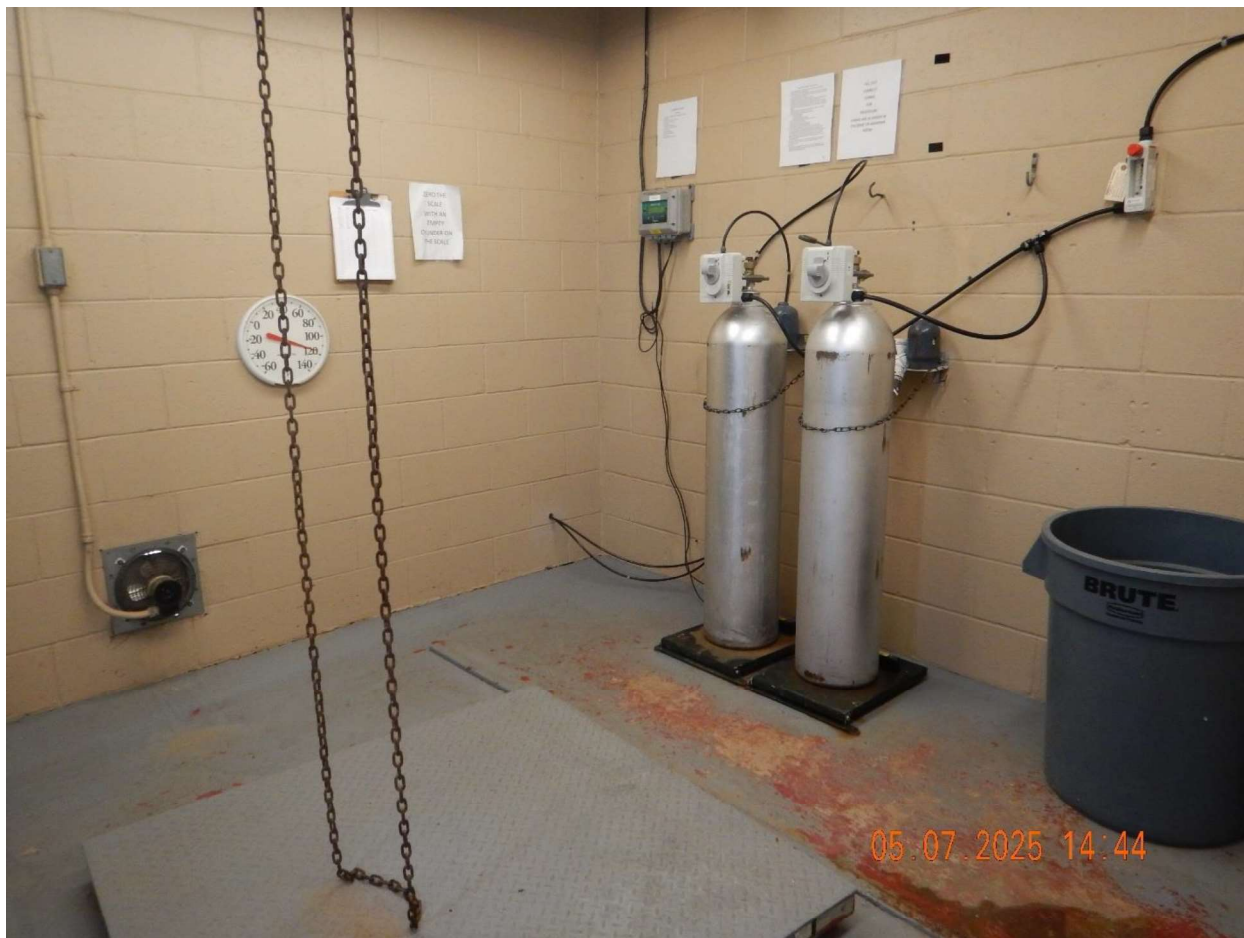
Thomas Booster Station View of gas chlorine tanks at Thomas booster station.
