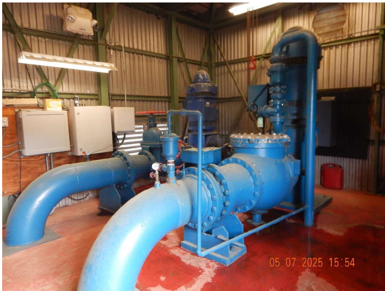
Pumps View of pumps at Bayou intake.
