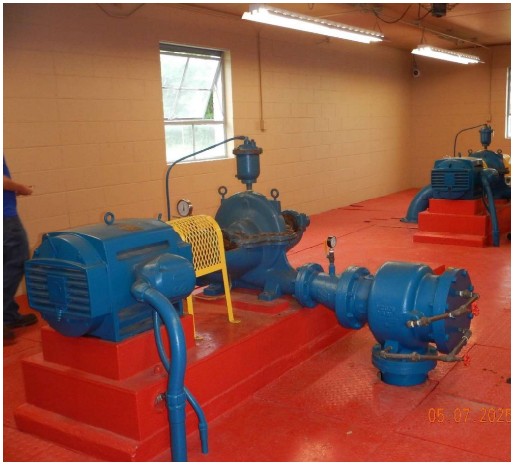
Ruffin Tank Booster Station View of Ruffin Tank booster station.
