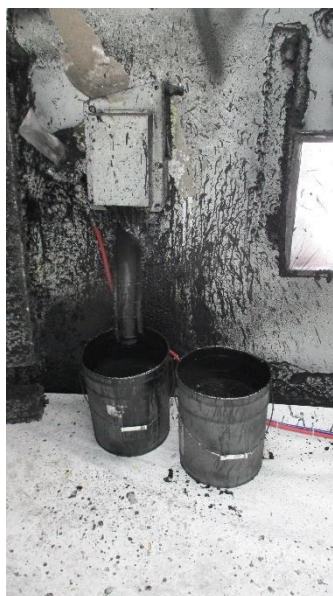
Figure 25: 12:19 PM - Building 1 - Spray Booth
