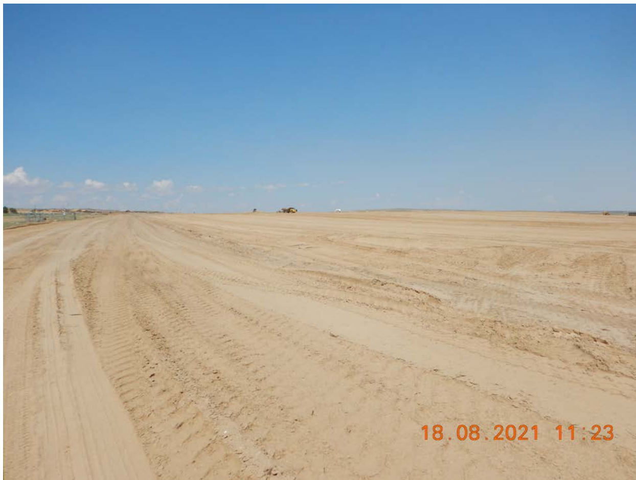
View looking approximately Northwest inside of Facebook facility. August 18, 2021 (DSCN1955).
