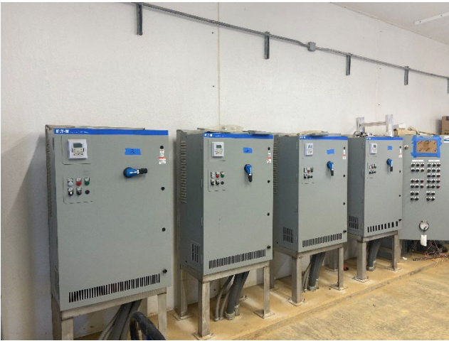
Photo 1: New blower controls.
