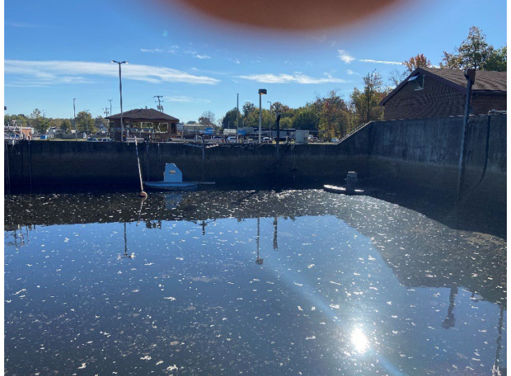
Photo 4: SBR Tank #1 (out of service).
