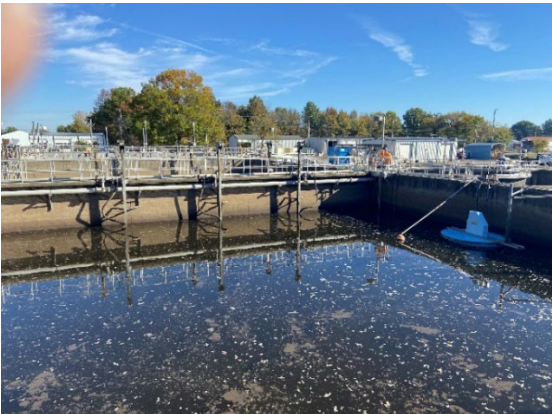
Photo 5: SBR Tank #1 (out of service).
