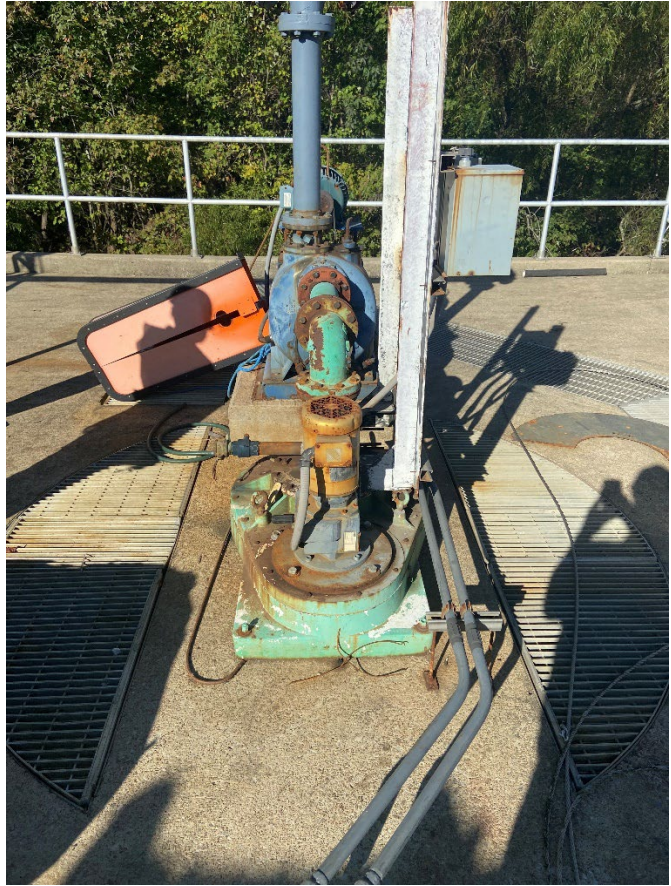
Photo 2: Vortex grit separator being out of service.
