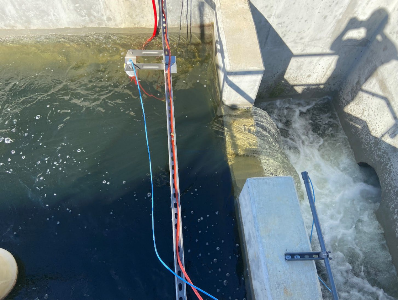
Photo 7: Effluent weir (with discharge).
