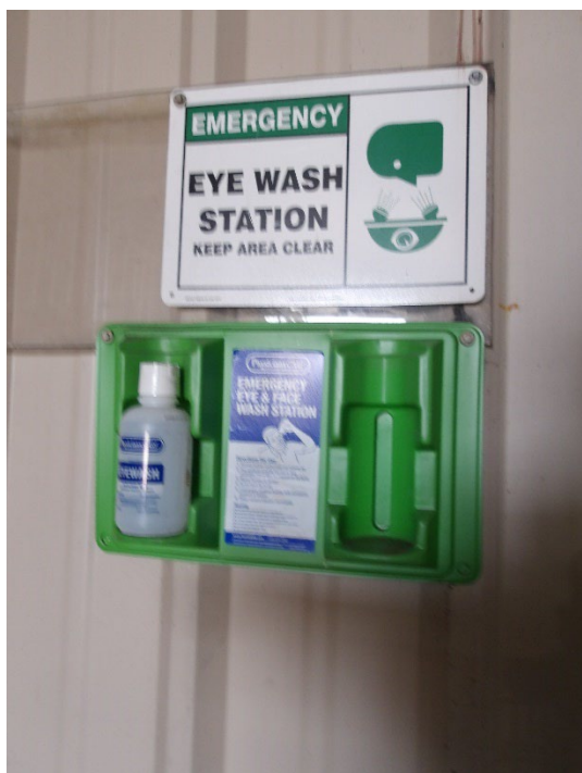
Photograph Seven (7): Eye Wash Station in the CAA
