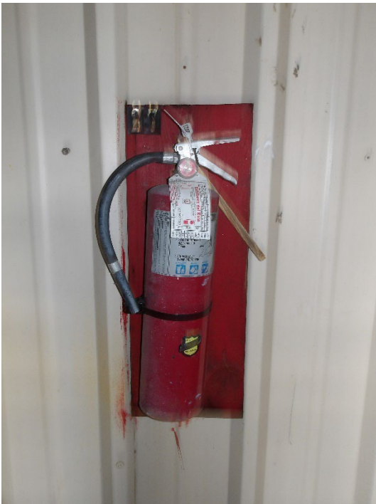
Photograph Six (6): Fire Extinguisher in the CAA
