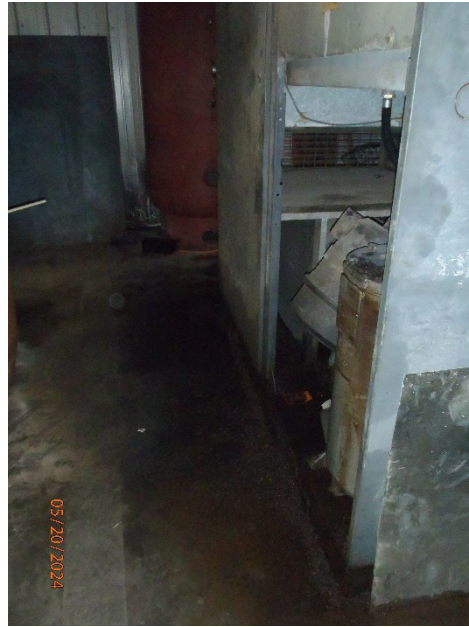
Picture 20 – Air Compressor Room used oil release
