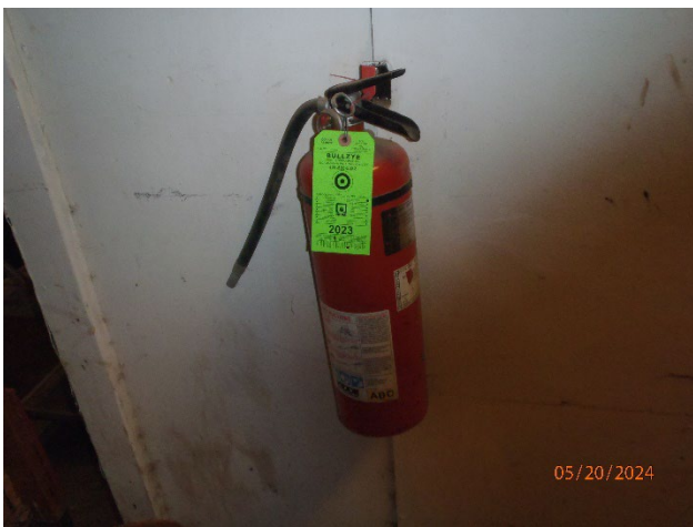
Picture 2 – Expired fire extinguisher annual certification tag
