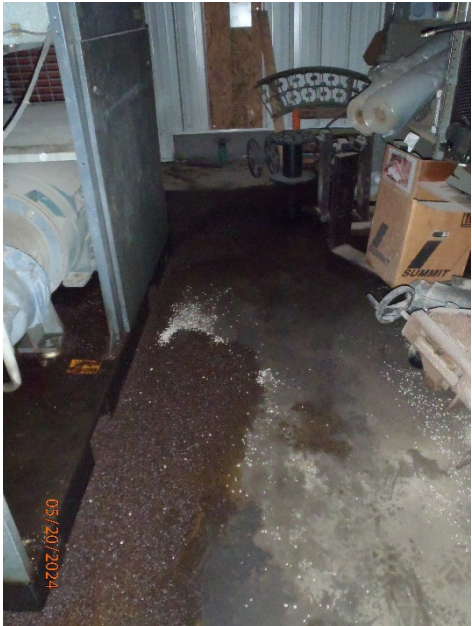
Picture 19 – Air Compressor Room used oil release
