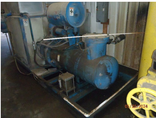
Picture 23 – Air Compressor Room used oil release
