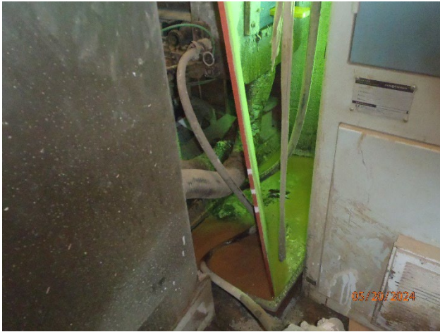
Picture 13 – Grid UV Staining UV catch basin
