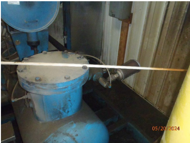
Picture 22 – Air Compressor Room used oil release
