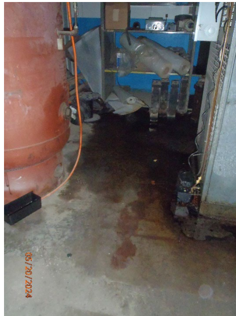
Picture 21 – Air Compressor Room used oil release
