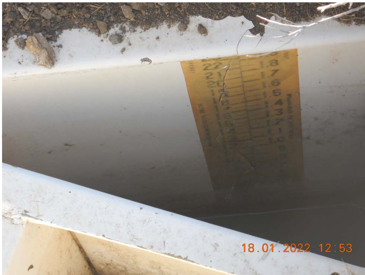
View of the flow staff at the entrance of the influent headworks-Parshall flume. (DSCN2086). Photographed by D. Esparza
