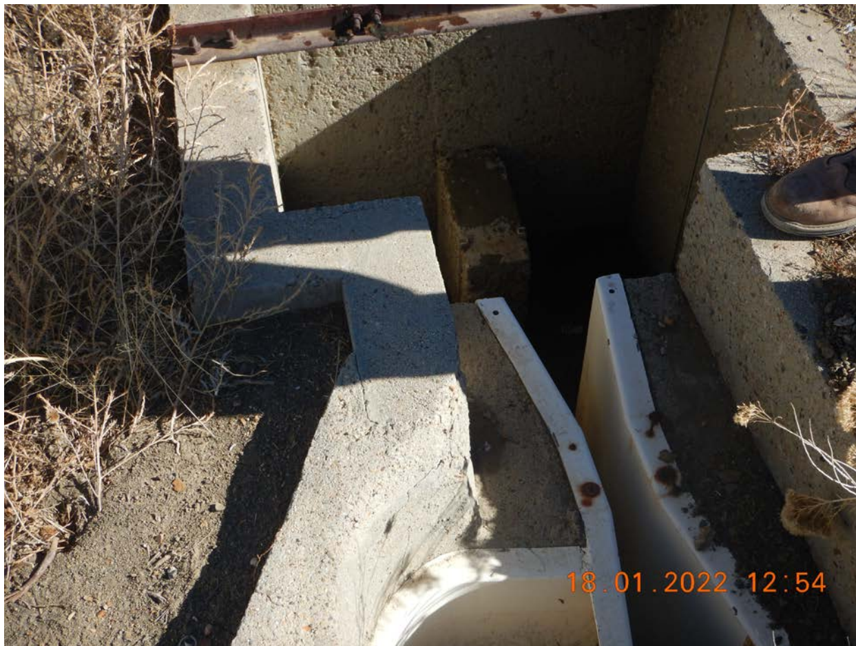
View of the influent headworks that consist of a Parshall flume without any screening of coarse solids, i.e., a bar screen system. (DSCN2085) Photographed by D. Esparza
