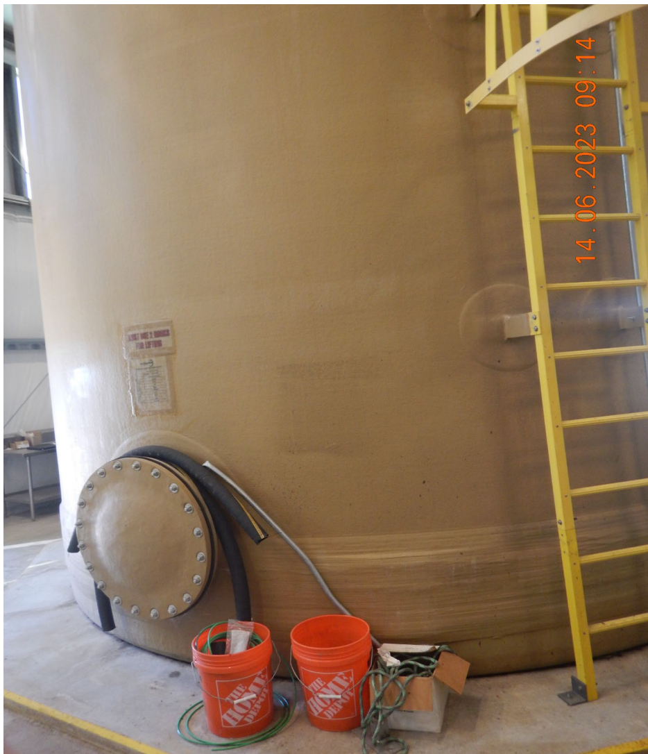
View of equalization (EQ) tank (DSCN2569) Photographed by D. Esparza
