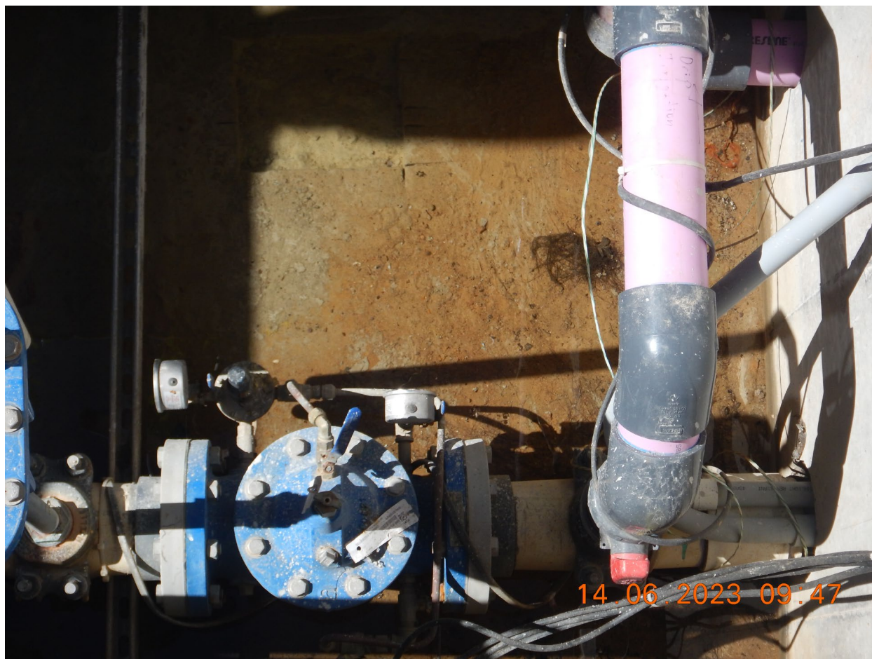
View of the landscape irrigation piping. Note: this piping configuration is located to the right of the above photograph. Additionally, a valve isolates the two (2) systems from each other. (DSCN2585) Photographed by D. Esparza
