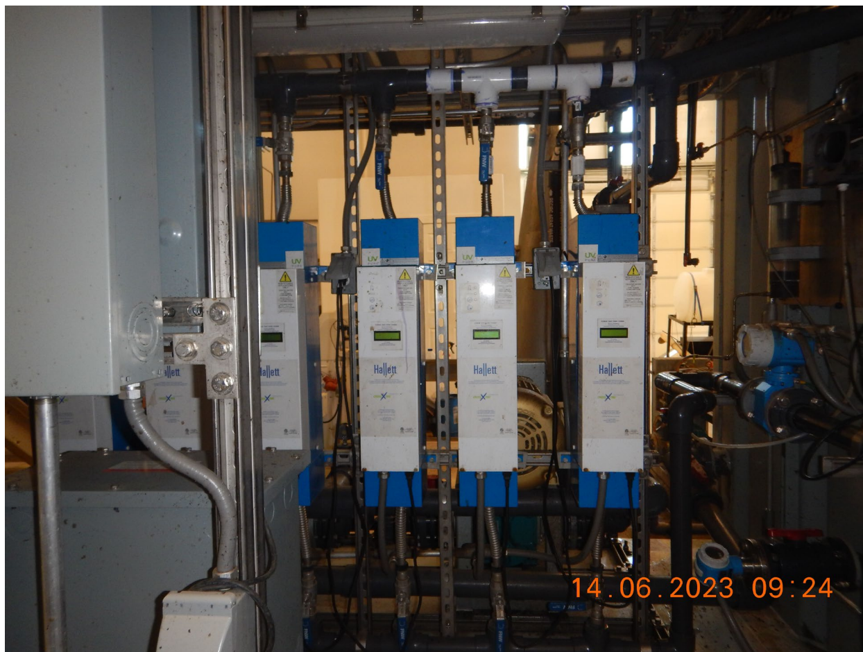
View of the six (6) banks of ultraviolet (UV) disinfection units prior to discharge to a 40K-gallon effluent storage tank. (DSCN2576) Photographed by D. Esparza
