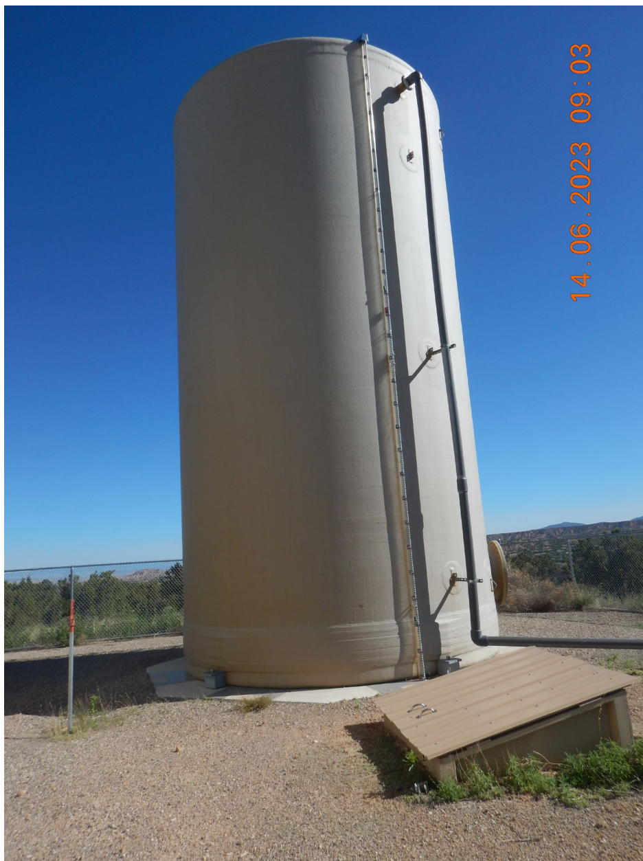
View of WWTP 40K-gallon effluent storage tank (DSCN2568) Photographed by D. Esparza
