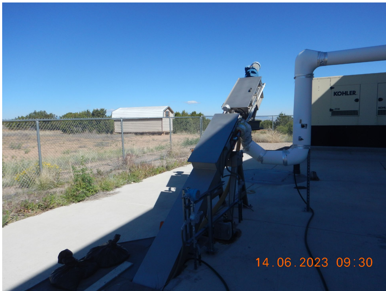
View of the headworks, lift station well pit and generator. (DSCN2581) Photographed by D. Esparza
