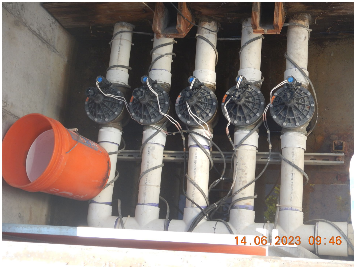
View of the leach field automatic valves piping. (DSCN2584) Photographed by D. Esparza
