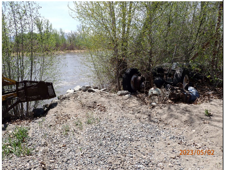
Photo #:16 Description: Facing east, photo of area of potential erosion on the northeastern corner of the property.
