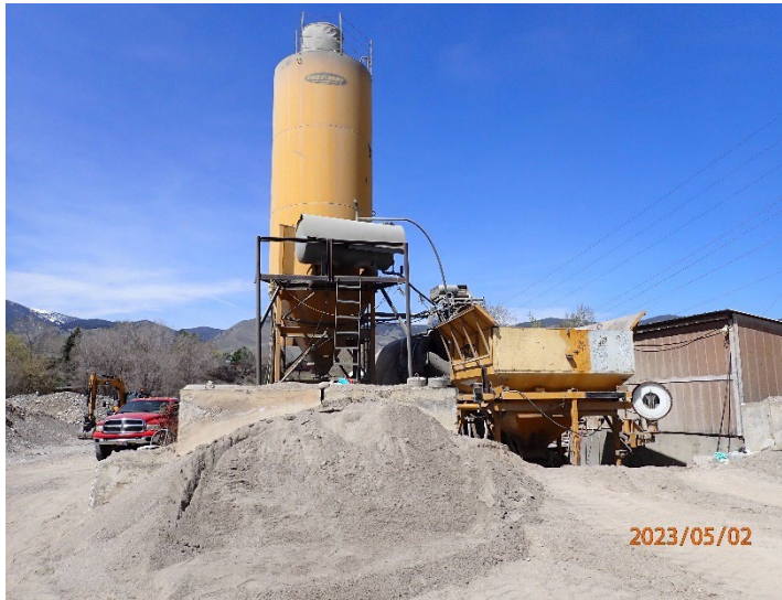
Photo #:13 Description: Facing north, photo of the batch plant.
