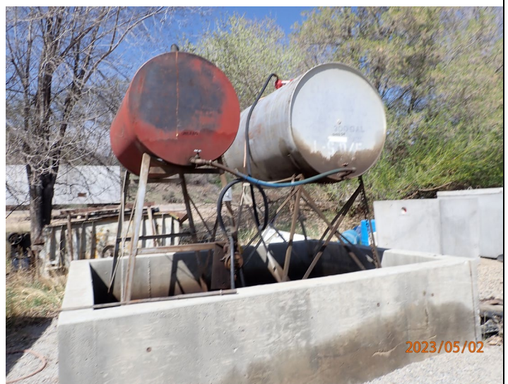
Photo #:08 Description: Facing west, photo of two tanks containing fuel.
