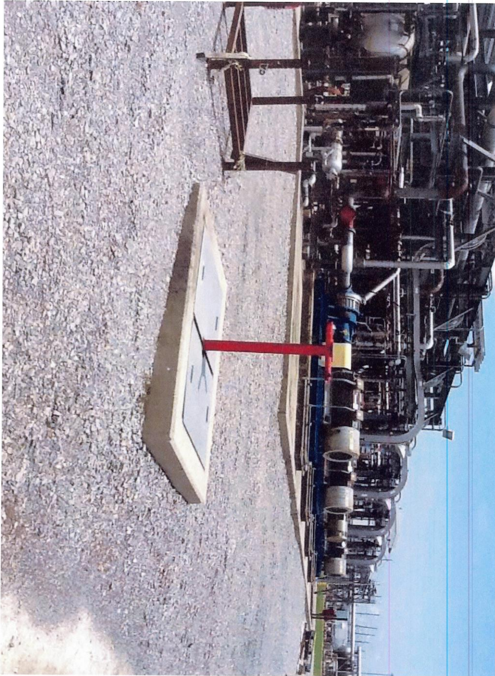
Compressors on Flare Gas Recovery System
