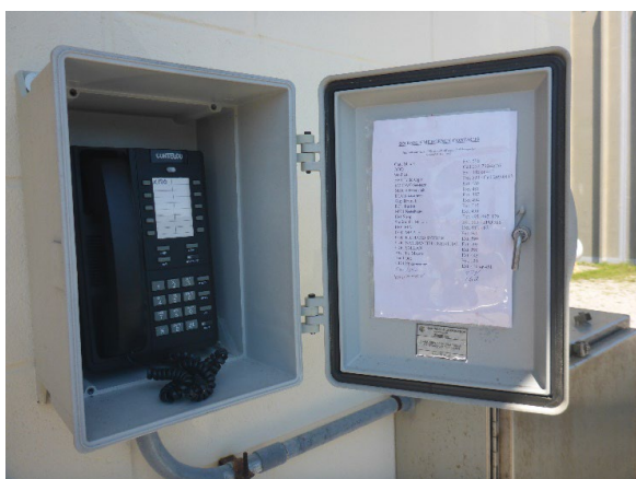
Photo 2: Emergency telephone at the CAA.
