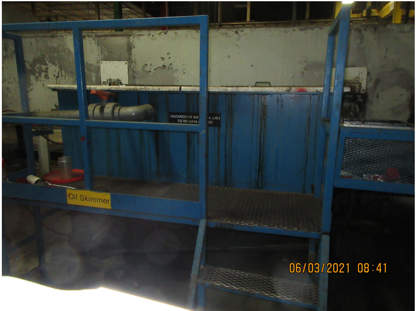
Photo 1 – Oil Skimming tank in Chemical Treatment Tank Area
