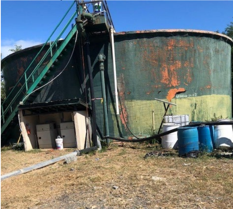
Photo #3: Vessup Plant
