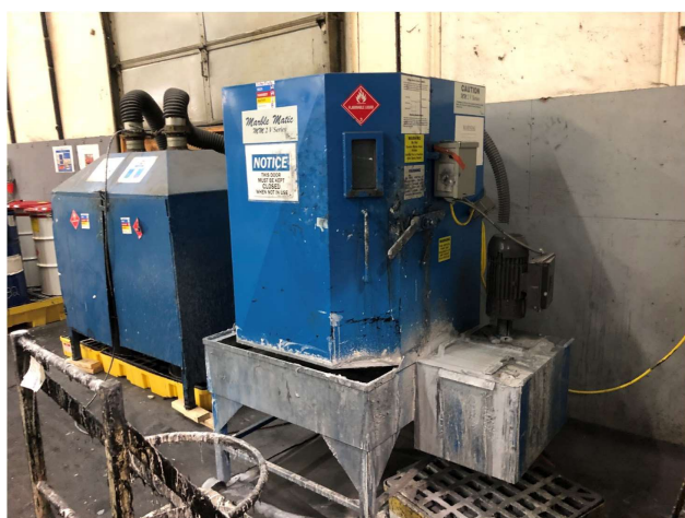
Photo 36: Pot washer machine with solvent reservoir.
