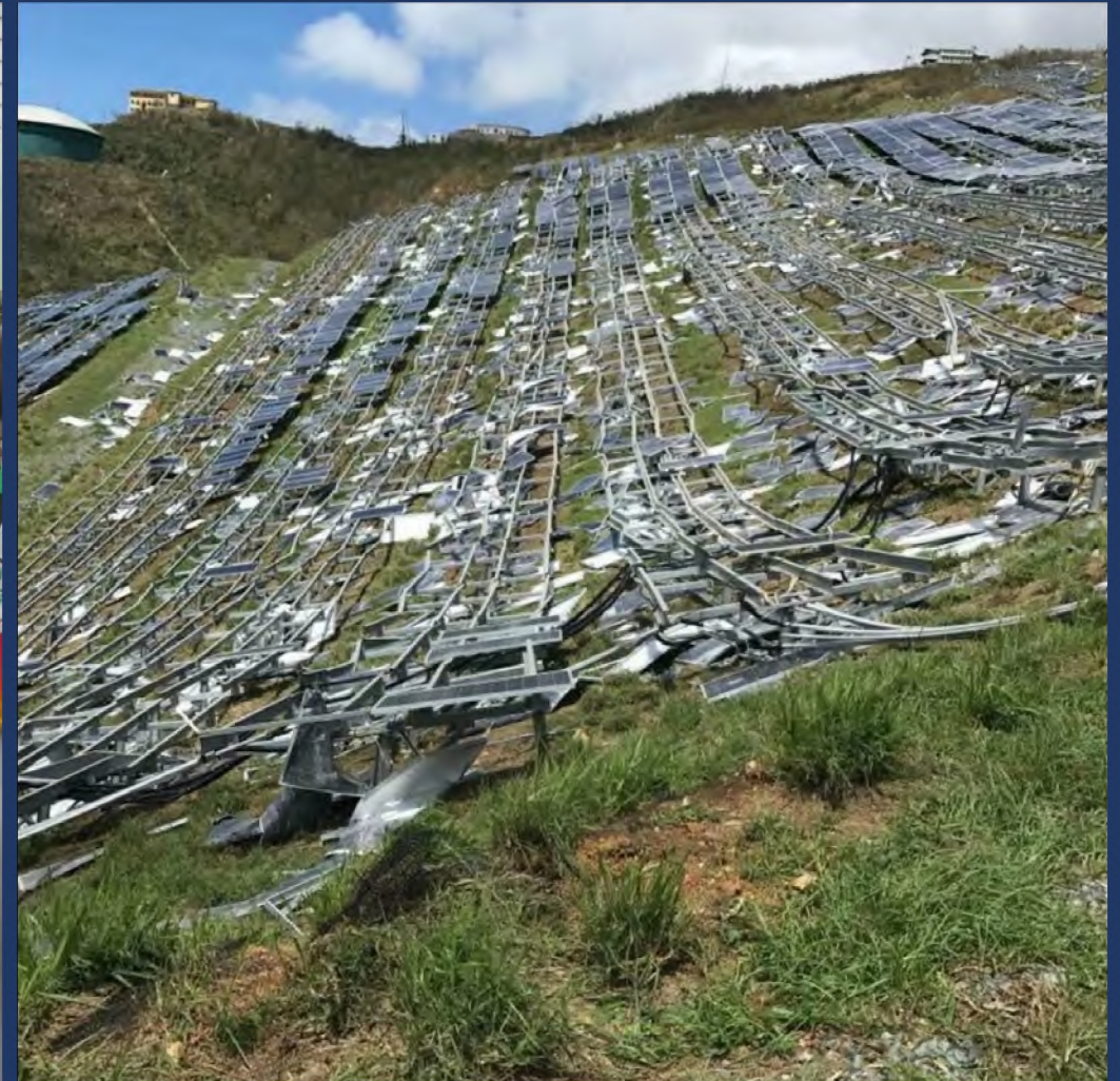
Damage to solar panel fields
