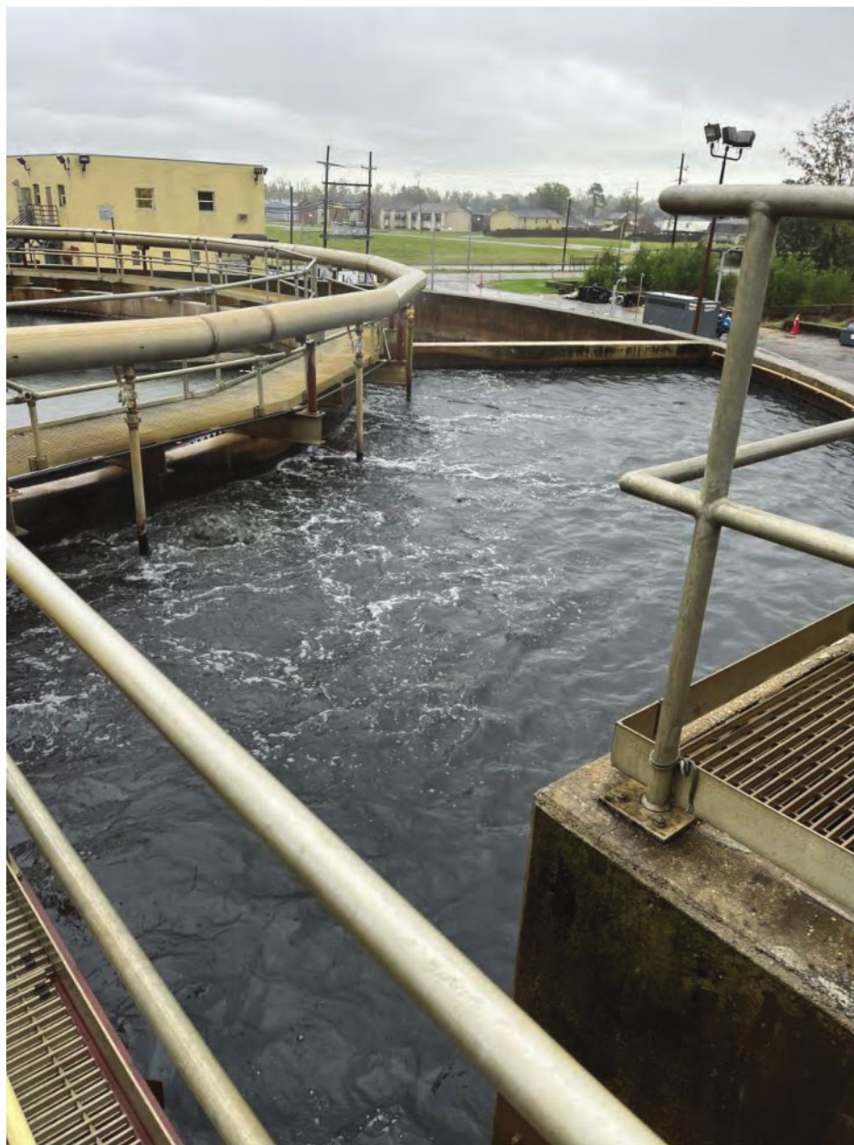
Woodland Treatment Aeration
