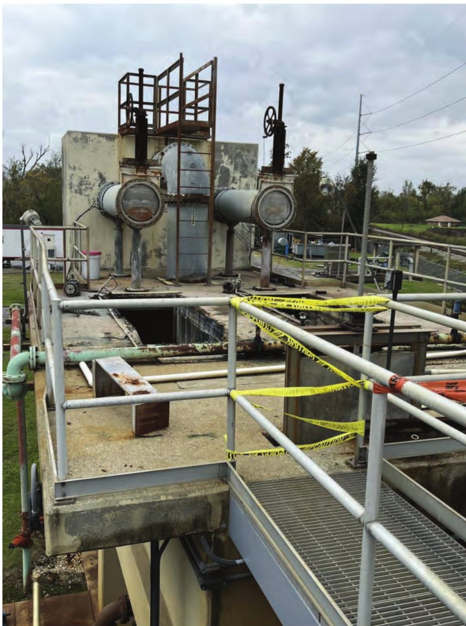
River Road WWTP Out of Service Bar Screen
