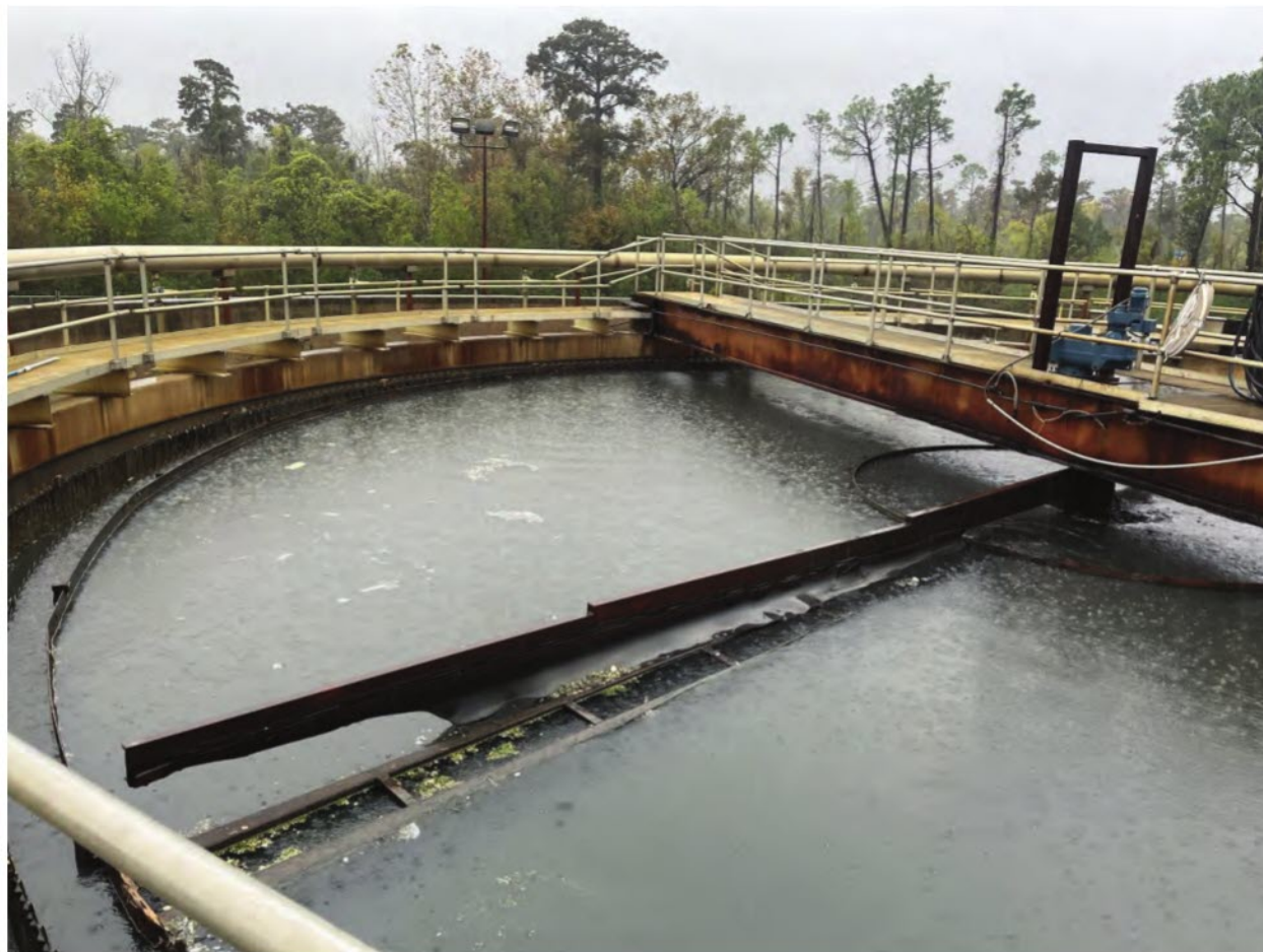
Woodland Treatment Clarifier with broken arm
