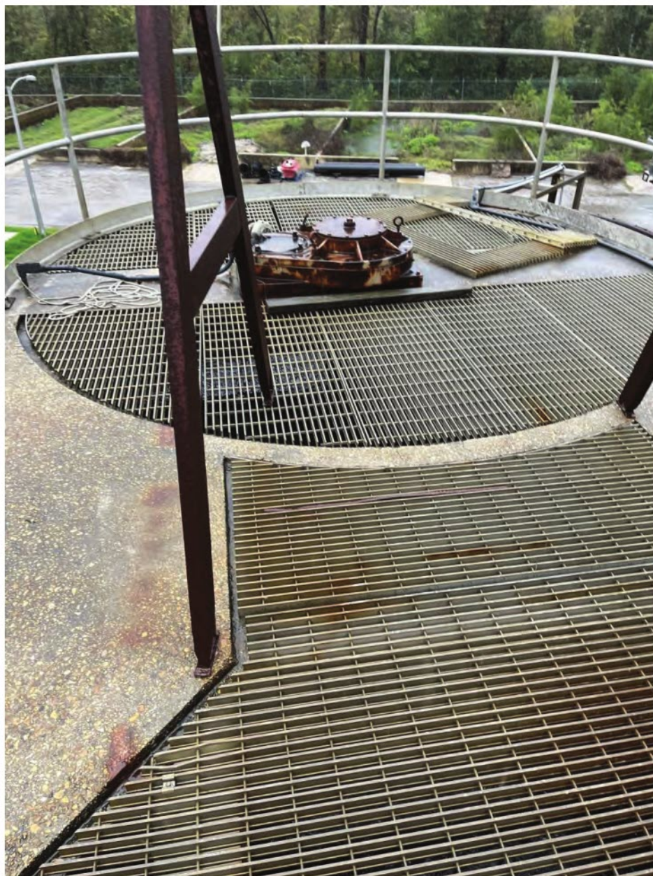
Woodland Treatment Grit Chamber
