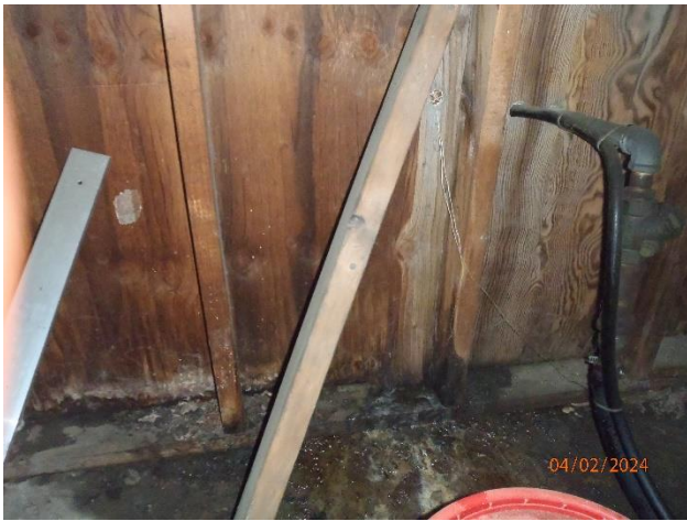
Picture 31 – Air Compressor Room used oil released to ground
