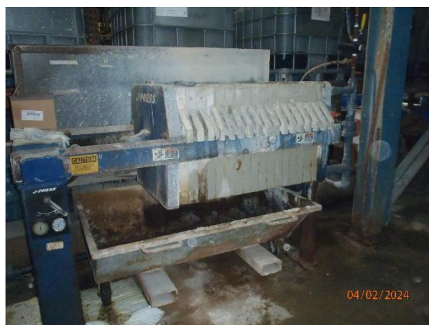
Picture 22 – WWTP floor press
