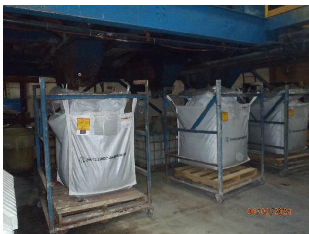
Picture 21 – WWTP CAA open supersacks
