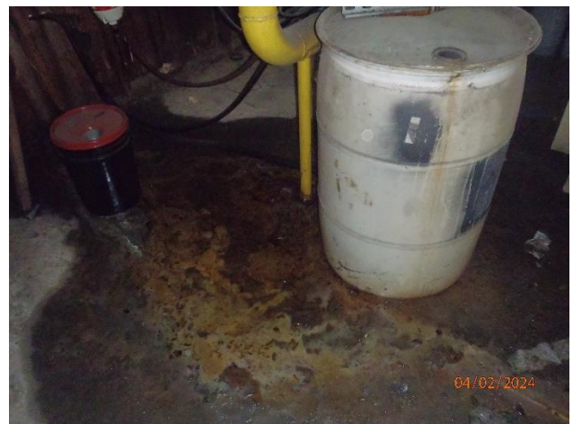
Picture 30 – Air Compressor Room used oil released to ground
