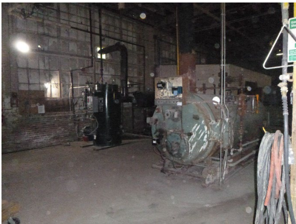
Photo 33: Old and New Boiler.
