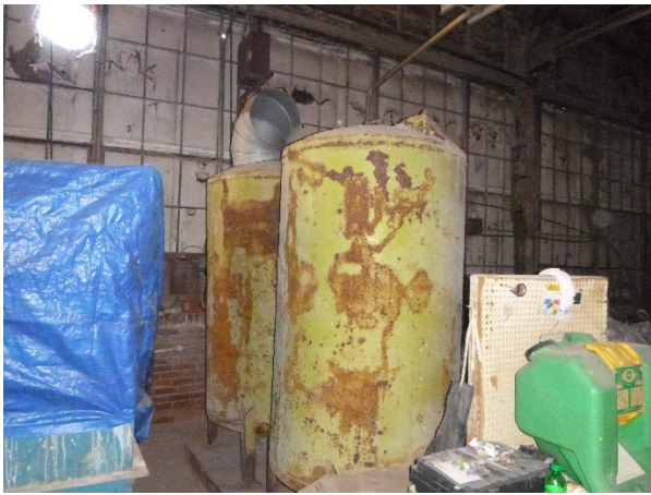
Photo 31: Tank 11 and empty old equipment.
