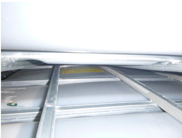
Photo 20: Former Non-Hazardous Waste CAA container with label not turned toward aisle.
