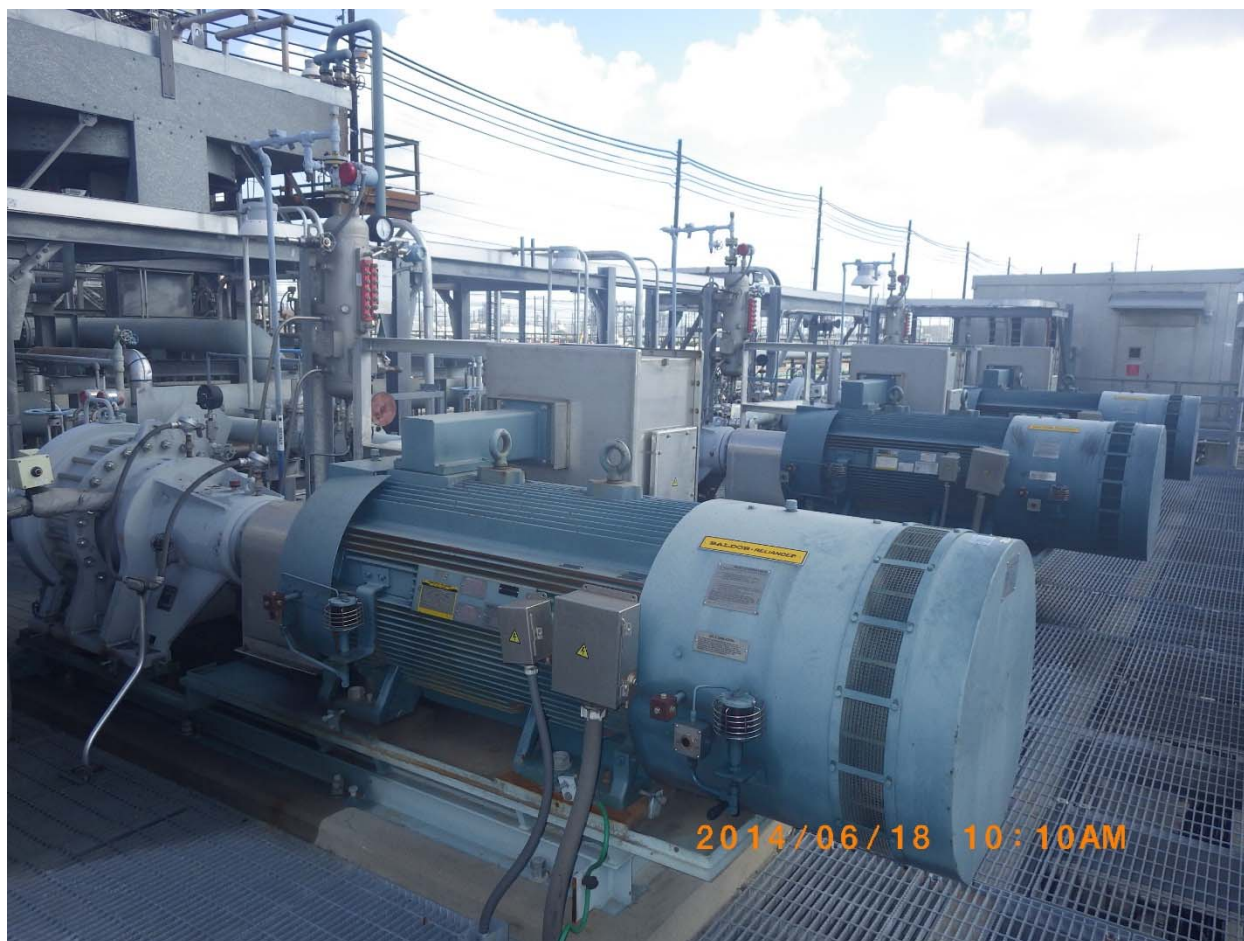
Flare Gas Recovery System (FGR) 7042 compressors (3)
