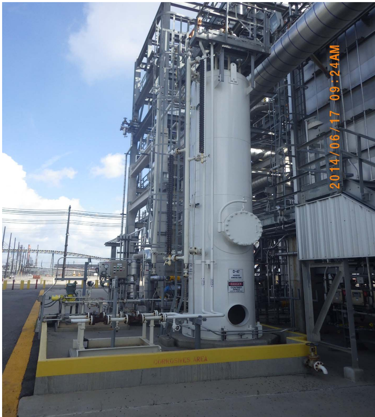
HCU 943 F-3 heater ammonia tanks used for SCR.
