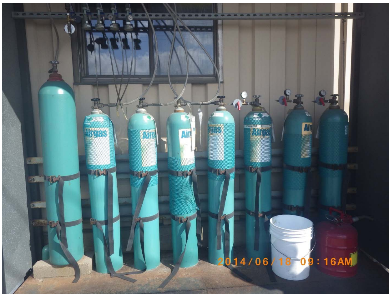
Calibration Gasses for Leak Detection and Repair monitoring instruments.
