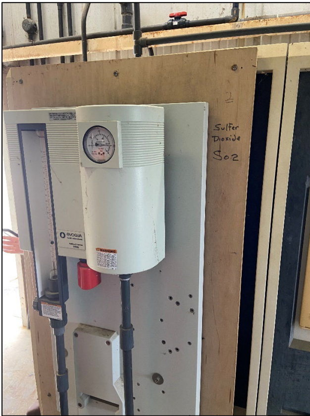
Photo 9: Sulfur Dioxide controls.
