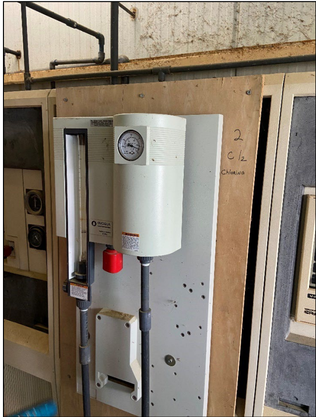
Photo 10: Chlorine gas controls.
