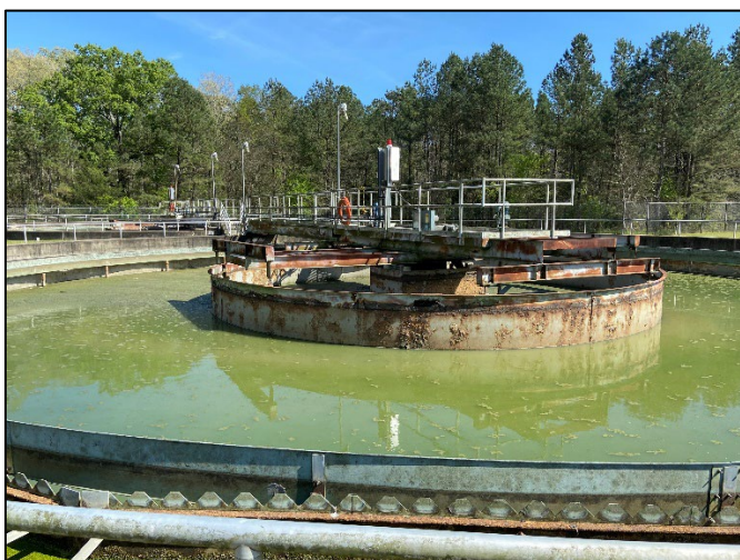
Photo 7: Clarifier #1 (out of service).
