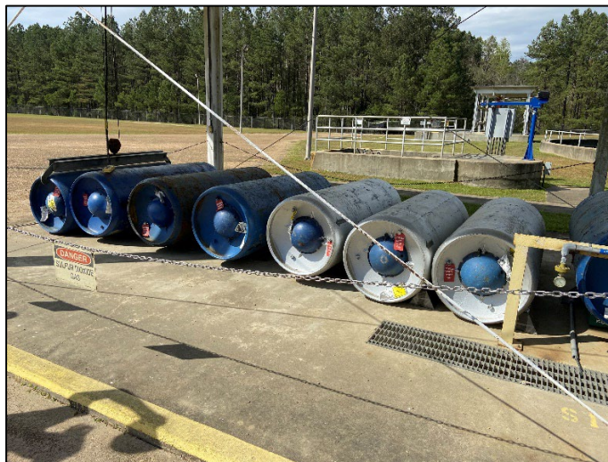
Photo 16: Gaseous sulfur dioxide cylinders.
