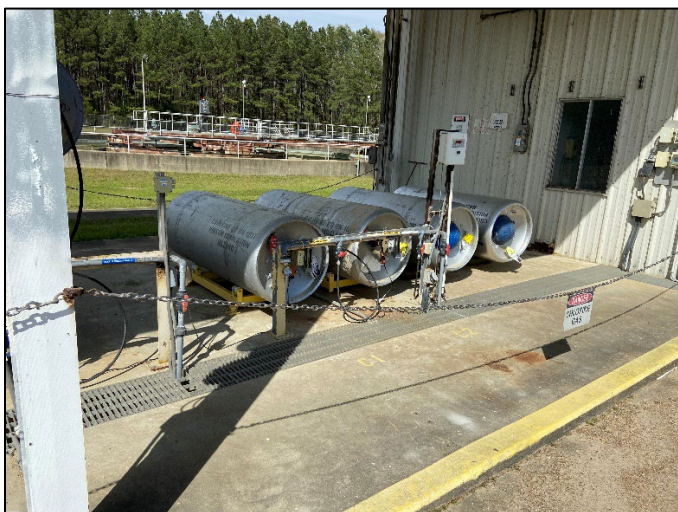
Photo 15: Gaseous chlorine cylinders.
