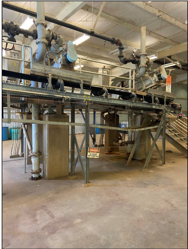
Photo 2: Grit classifiers (out of service).
