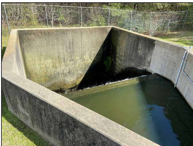
Photo 13: Stair-step aeration of final effluent.
