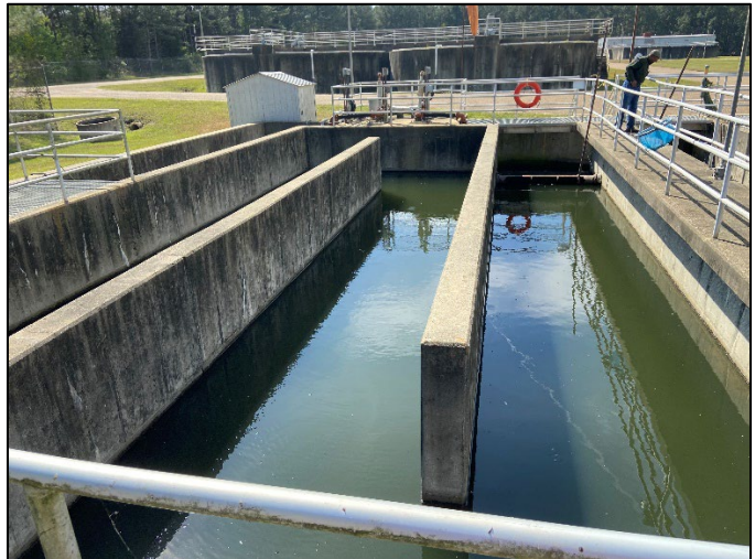
Photo 12: Chlorine contact chamber #2 (not in use).
