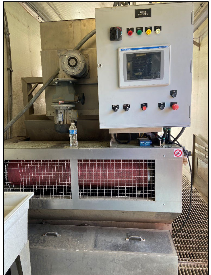
Photo 18: Trailer-mounted sludge filter press.
