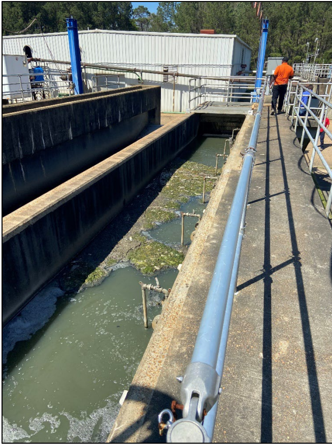
Photo 1. Influent grit chamber.
