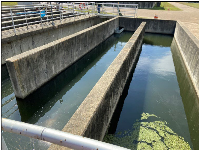
Photo 11: Chlorine contact chamber #1
