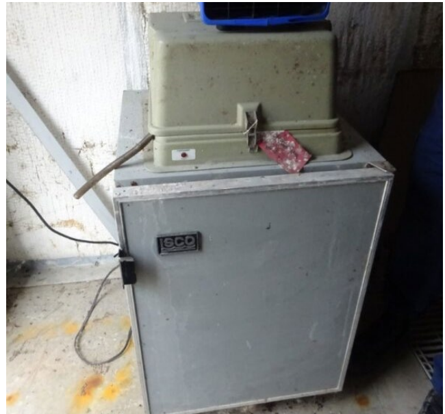
Photograph #14 (DSC03554) Description: The treatment plant's out of service composite sampler.
