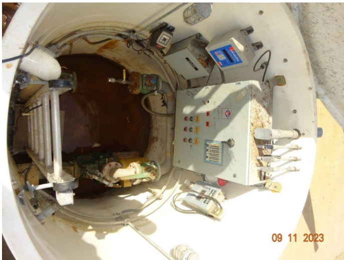
Photograph #19 (DSC03579) Description: Control box for the DC lift station. Note that the controls are located below grade.
