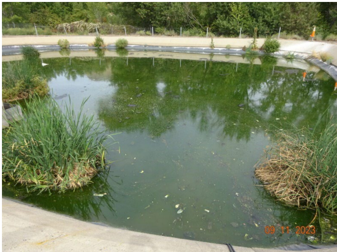
Photograph #07 (DSC03526) Description: Aerobic digester. Note the floating islands of vegetation as well as other solids within the digester. Not pictured are two surface aerators that were out of service.
