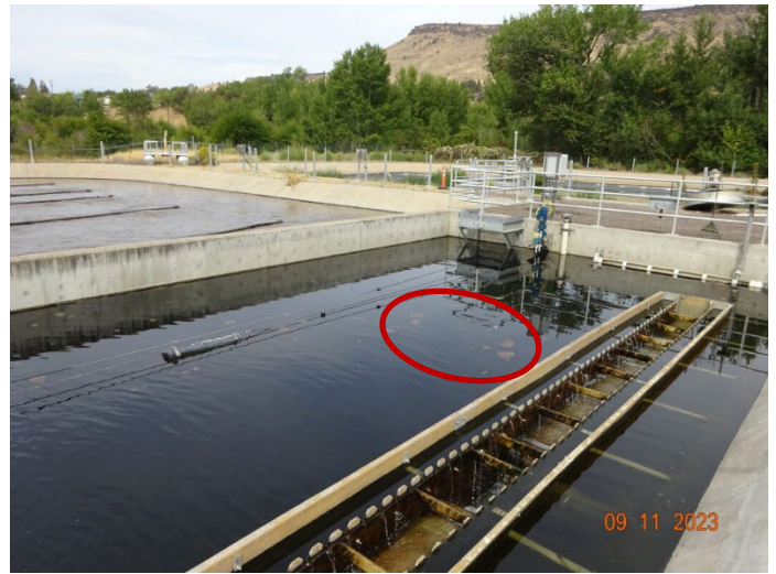
Photograph #06 (DSC03524) Description: North clarifier with a weir in the middle that flows to the UV disinfection room. Note some solids floating at the top of the clarifier, outlined in red.
