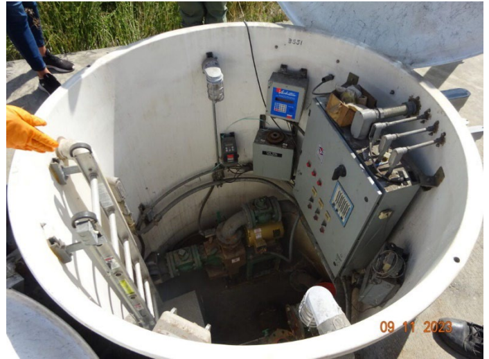
Photograph #18 (DSC03570) Description: Control box for the Composites lift station. Note that the controls are located below grade.
