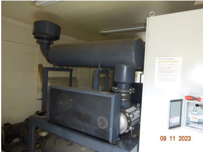
Photograph #05 (DSC03540) Description: One of the treatment plant's three blowers.
