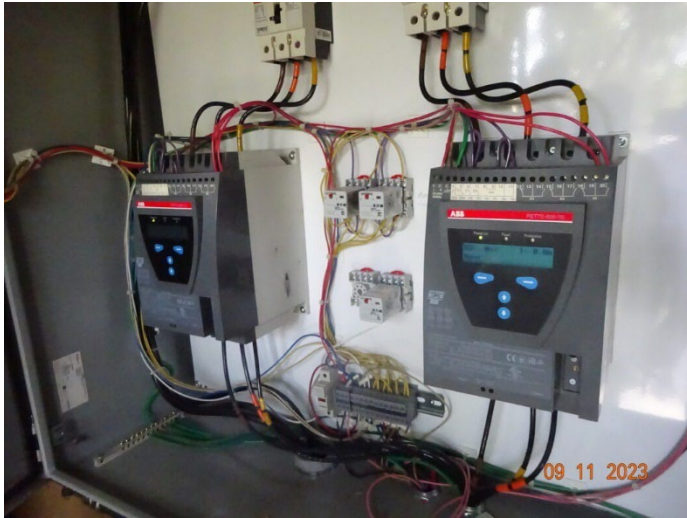
Photograph #17 (DSC03569) Description: Control box for the Museum lift station. The controls were located in a shed next to the pumps.
