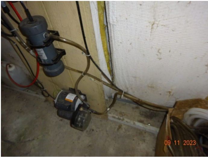
Photograph #13 (DSC03550) Description: Bio-growth observed in the tubing to the online ammonia, pH, and temperature analyzer.
