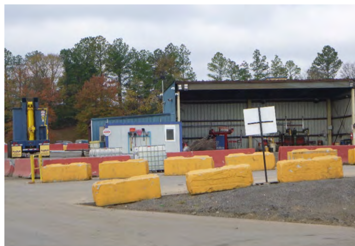
Photograph 5: Vehicle crusher and depollution equipment.
