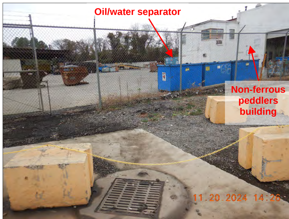
Photograph 14. DSCN0729.JPG View, facing northwest, of a storm drain inlet south of the non-ferrous peddlers building. A BMP was not installed at the storm drain inlet. Facility staff placed an absorbent sock around this inlet during the inspection.
