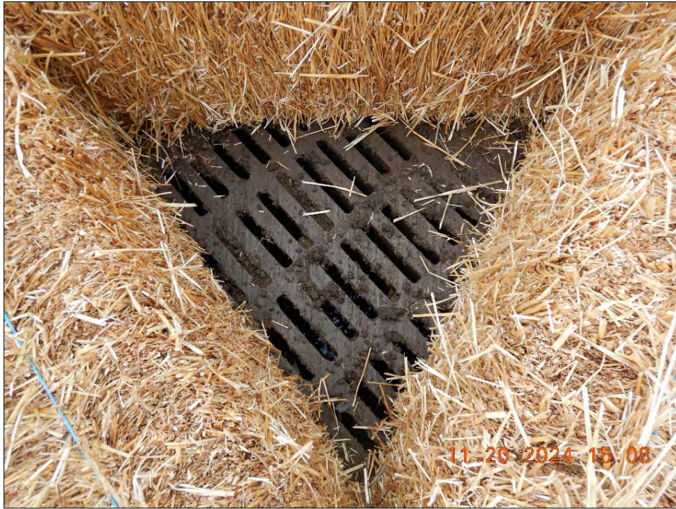
Photograph 31. DSCN0758.JPG Close-up view of the storm drain inlet shown in Photographs 29 and 30.
