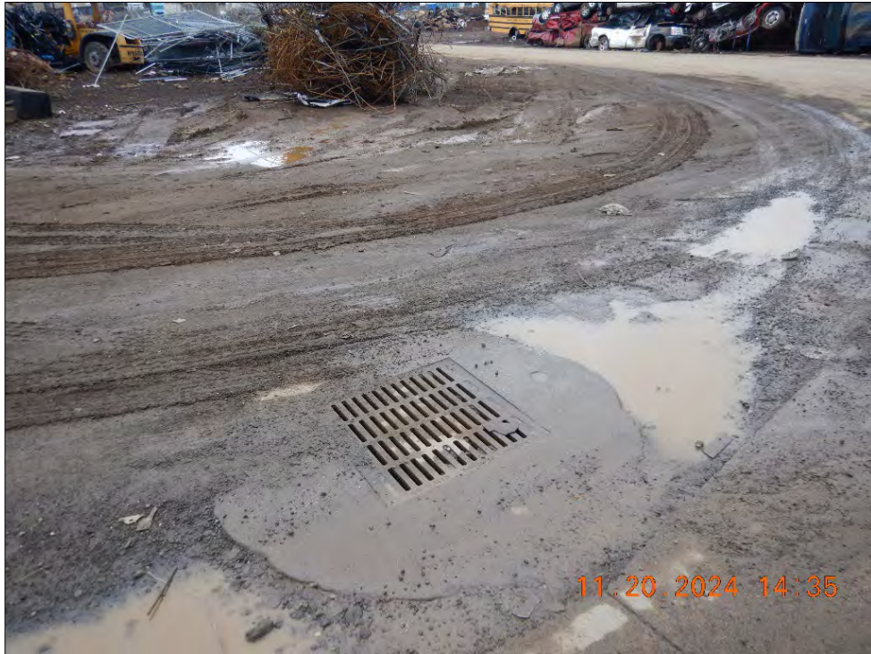
Photograph 21. DSCN0735.JPG View of the storm drain inlet shown in Photograph 20. Note sediment adjacent to and inside the grating of the storm drain inlet.
