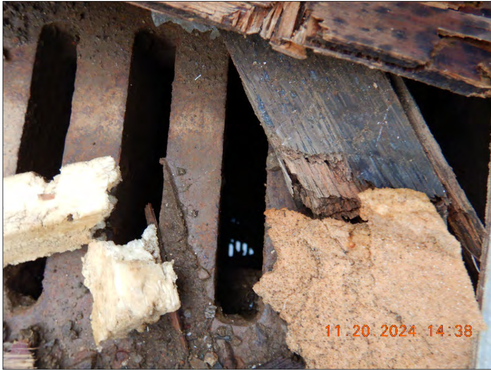
Photograph 25. DSCN0740.JPG Close-up view of the storm drain inlet shown in Photographs 23 and 24.
