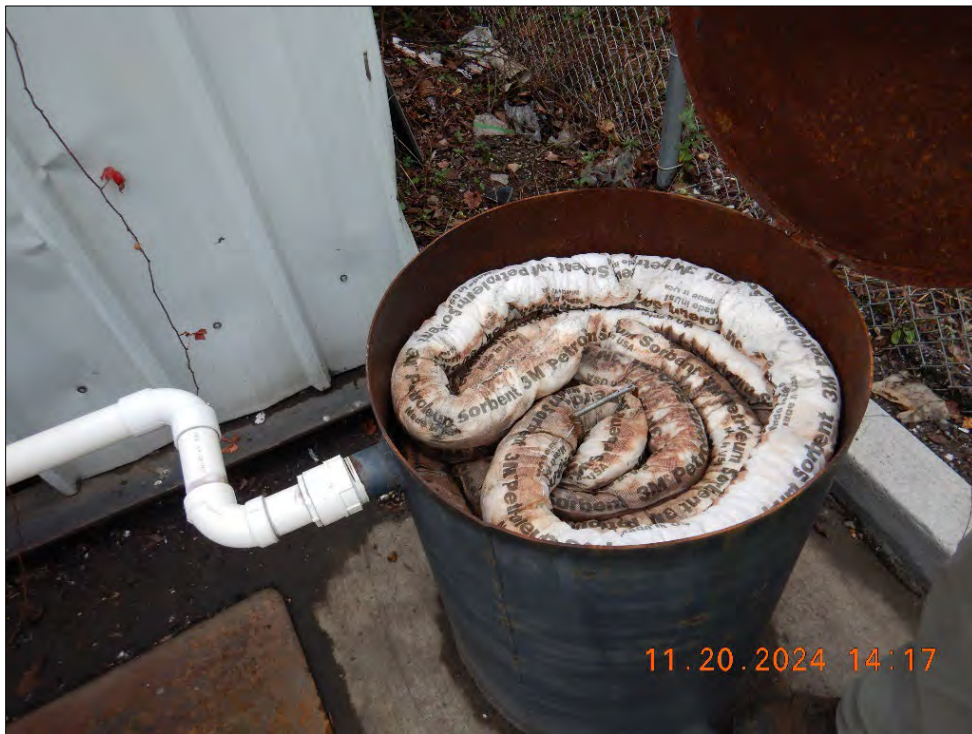
Photograph 12. DSCN0724.JPG View of the container with absorbent socks to which water from the oil/water separator flows. Water then flows to an outside area with hay bales to the east of the oil/water separator.
