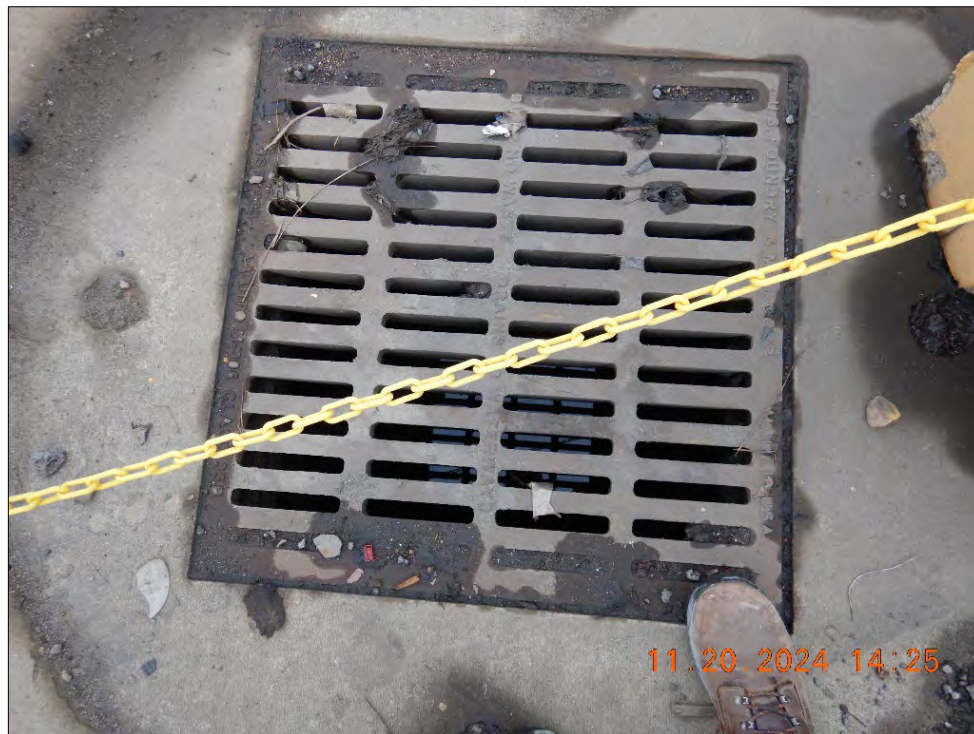
Photograph 16. DSCN0727.JPG Close-up view of the storm drain inlet shown in Photographs 14 and 15.
