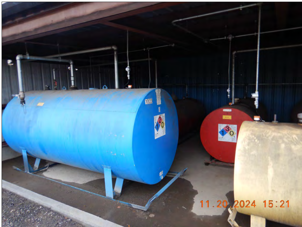
Photograph 42. DSCN0762.JPG View of the SEDA tank farm used to store fluids removed from the SEDA system.
