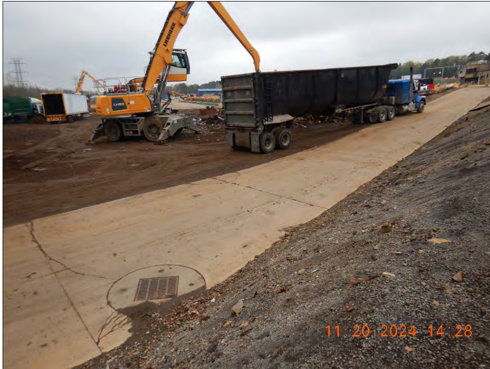
Photograph 17. DSCN0730.JPG View of a storm drain inlet on the north side of the scrap storage/sorting area. A BMP was not installed at the storm drain inlet. The inlet was adjacent to and downgradient of a dirt/gravel slope. A Facility staff placed an absorbent sock around this inlet during the inspection.
