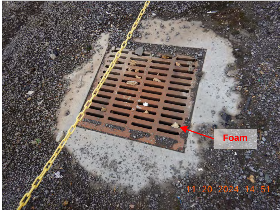
Photograph 38. DSCN0749.JPG Close-up view of the storm inlet shown in Photograph 38. Foam material was observed in the grating and inside the storm drain. Facility staff placed hay bales around this inlet during the inspection.
