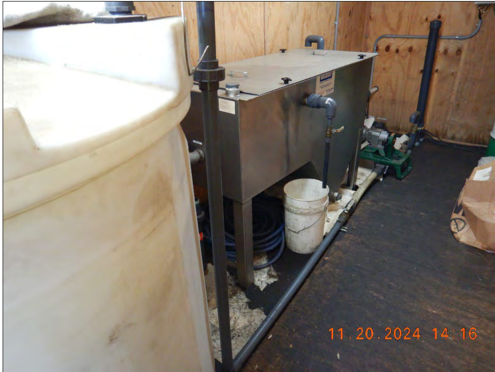
Photograph 11. DSCN0723.JPG View of the oil/water separator that treats oil/water mixture from the sealed components area.
